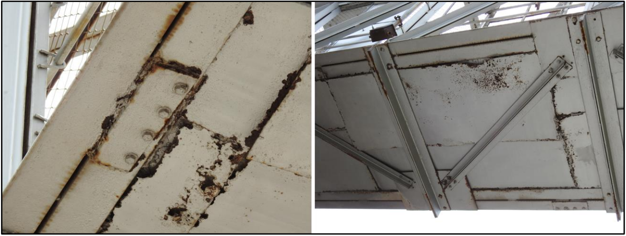
Fig 1.7: Corrosion observed at bottom chord members along the span of FOB
