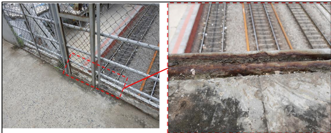
Corrosion at bottom chord members
