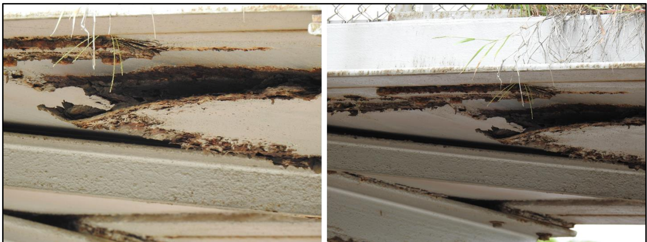
Corrosion of sacrificial plate
