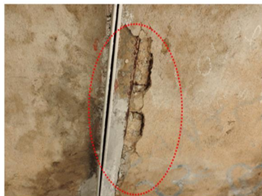
Fig: 2.6 spalling, Reinforcement exposure and cracks is observed at staircase 1
