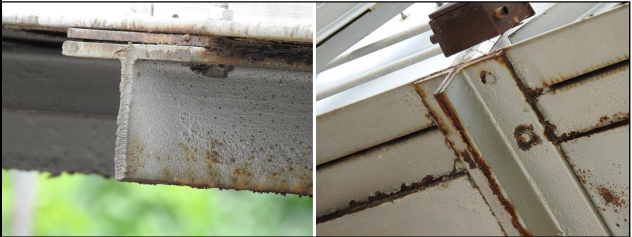
Corrosion observed at gusset plate and floor beams
