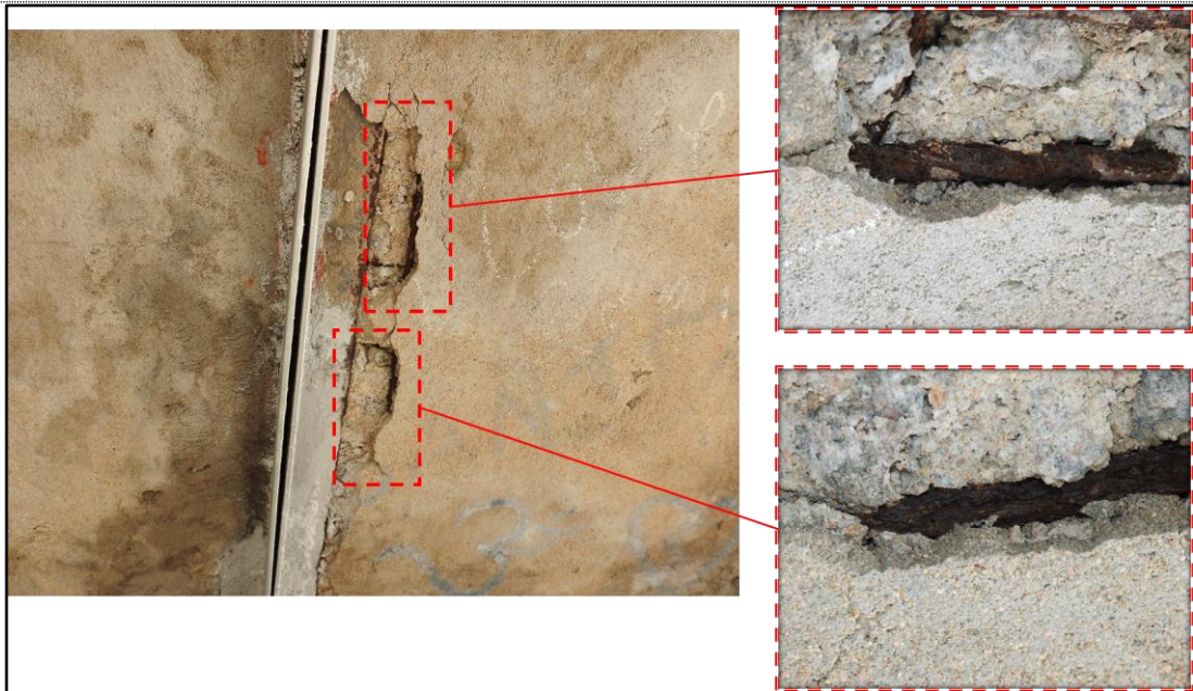
Spalling and corrosion on reinforcement
