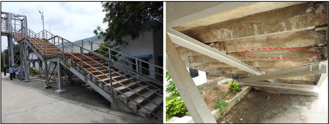
Fig 1.8: View of staircase and cracks in Pre-cast RCC panels in staircase at PF-1
