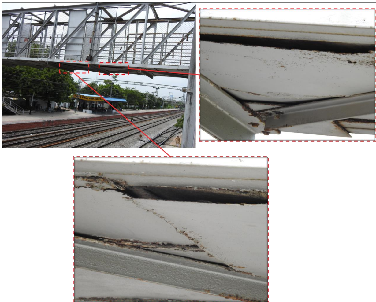
Fig 1.4: Corrosion of sacrificial plate
