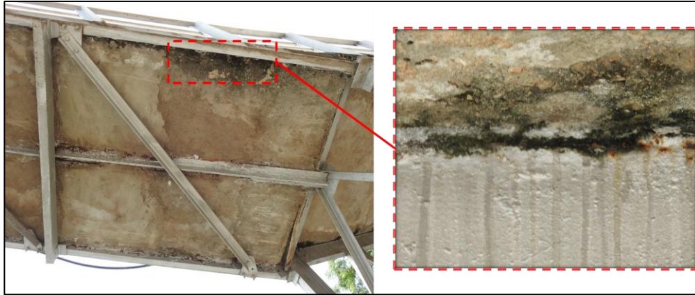
Dampness and formation of algae observed
