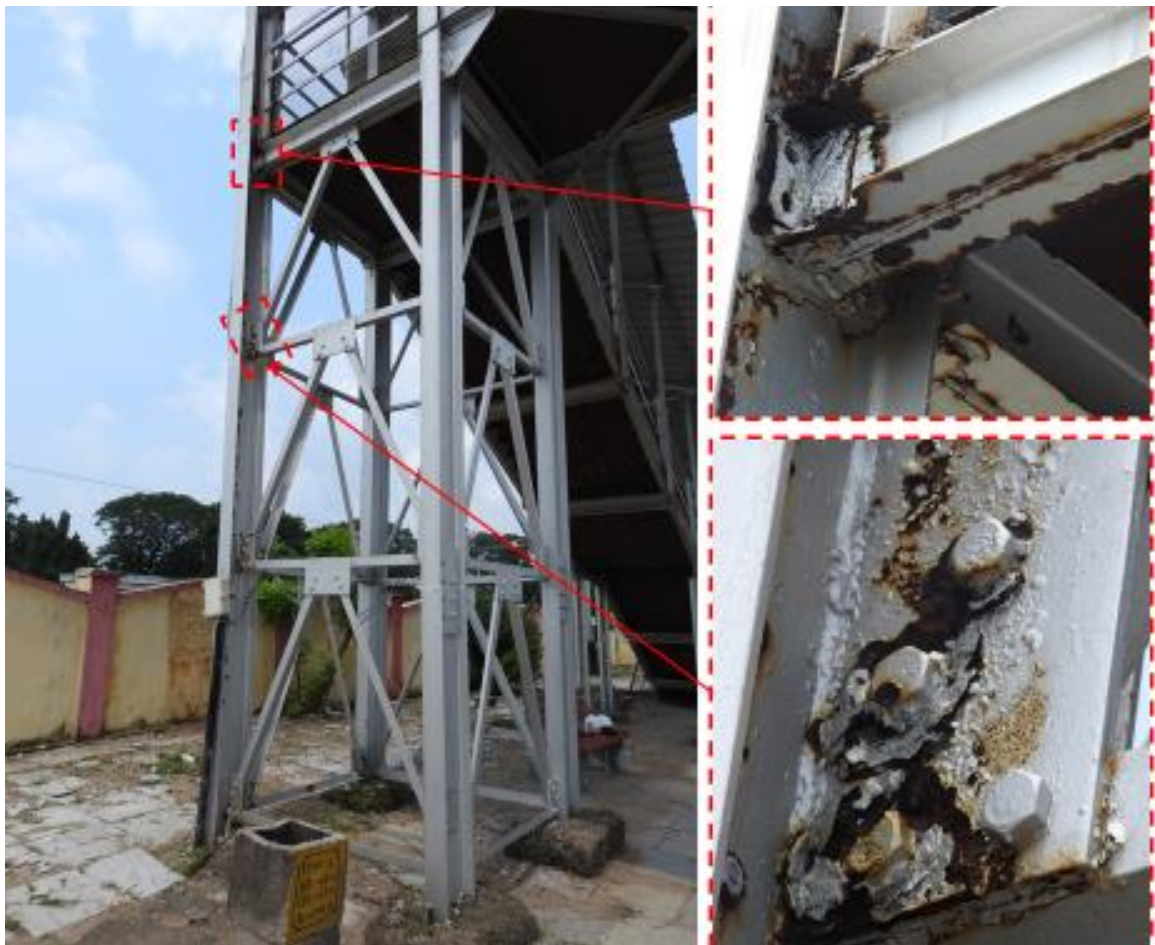
Fig: 2.2 Corrosion in floor beam at beam column joint
