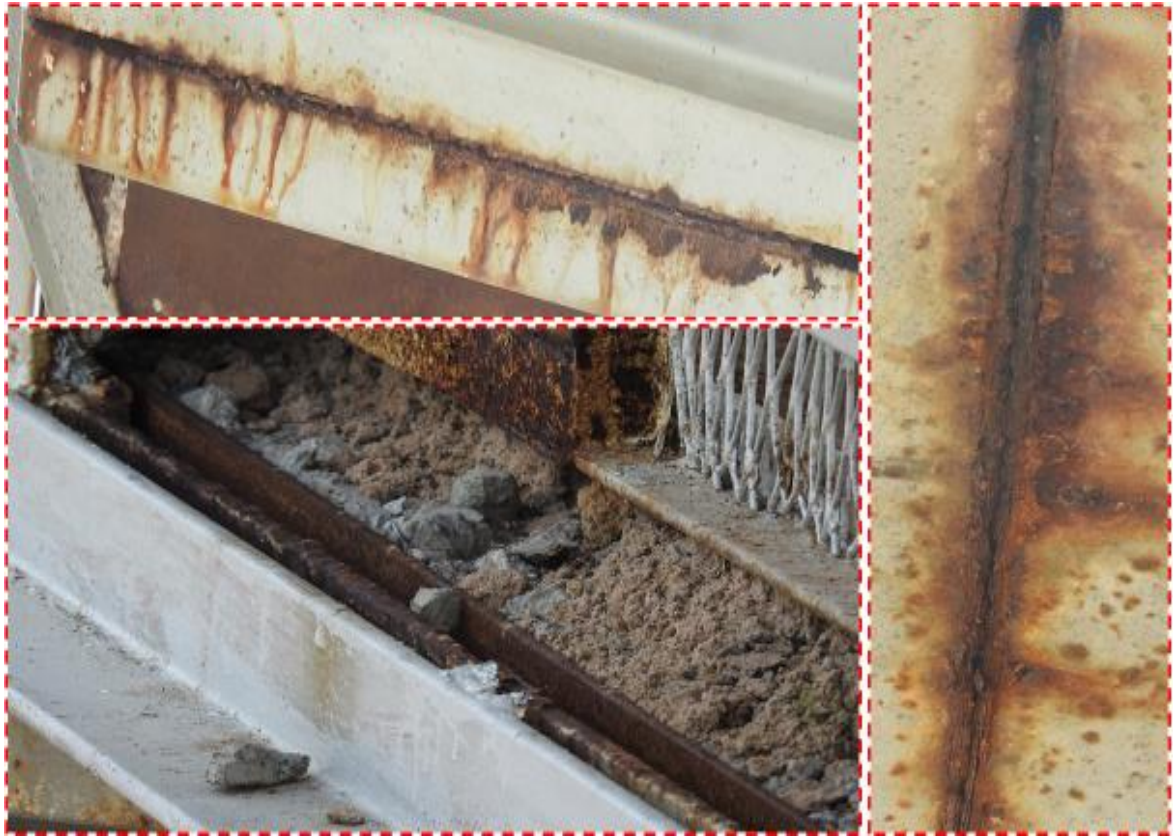
Fig: 2.3 Corrosion at bottom chord members and floor beams
