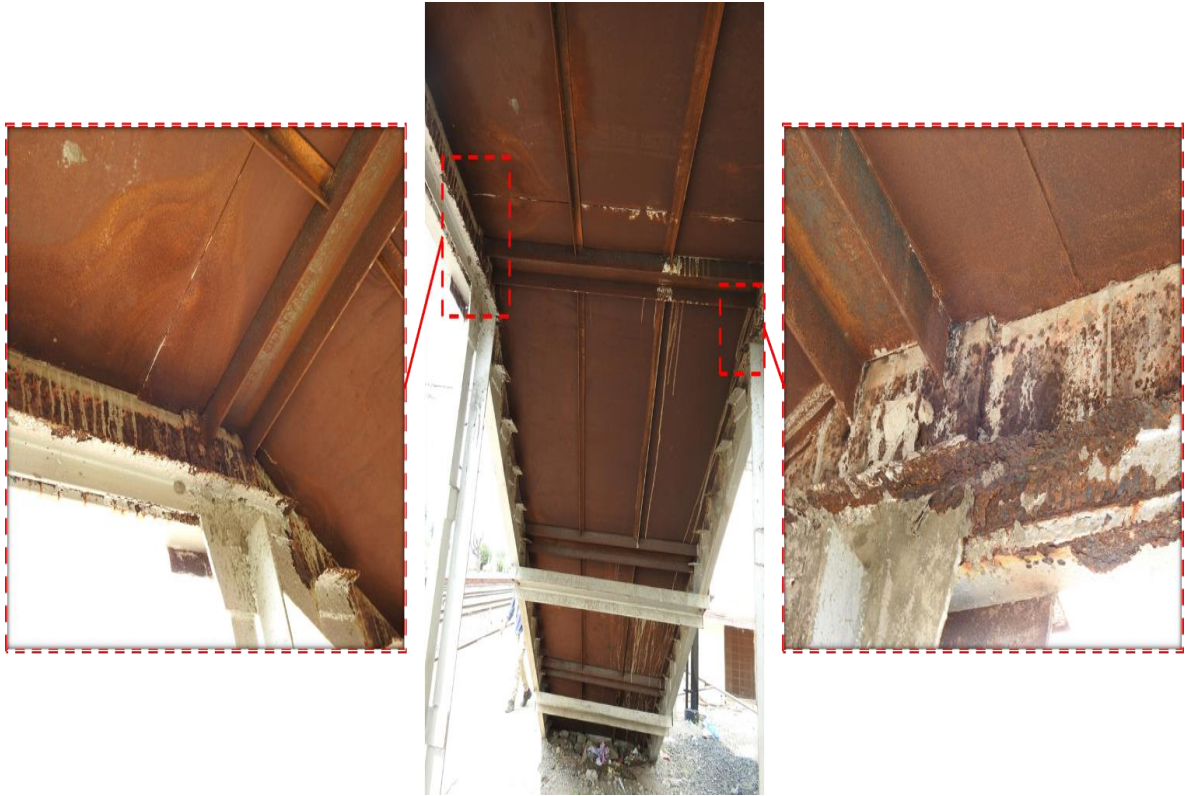
Fig: 2.5 Corrosion of staircase stringer beam
