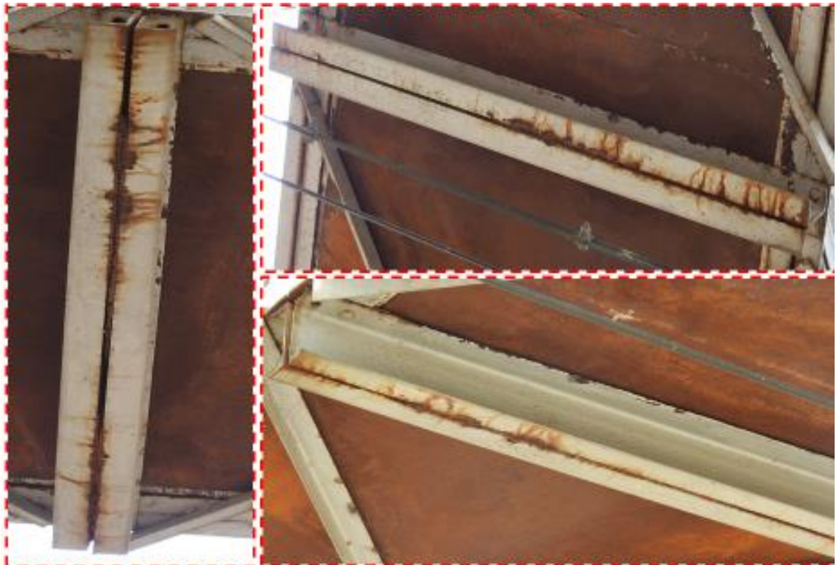
Fig: 2.4 corrosion at floor beams
