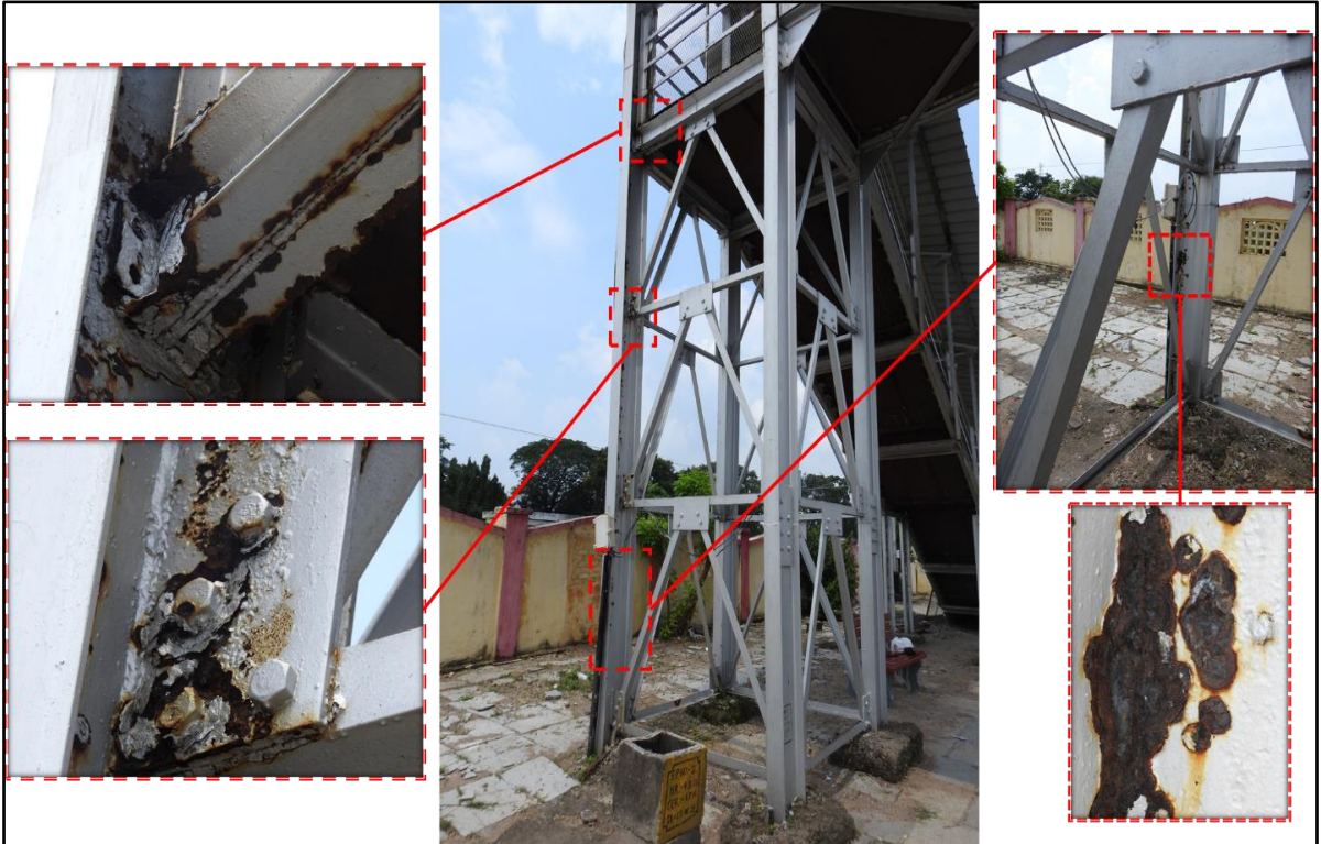
Corrosion Major corrosion observed
