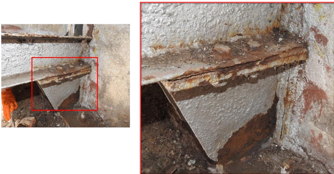
Fig 2.3: Corrosion of bottom chord and gusset plate
