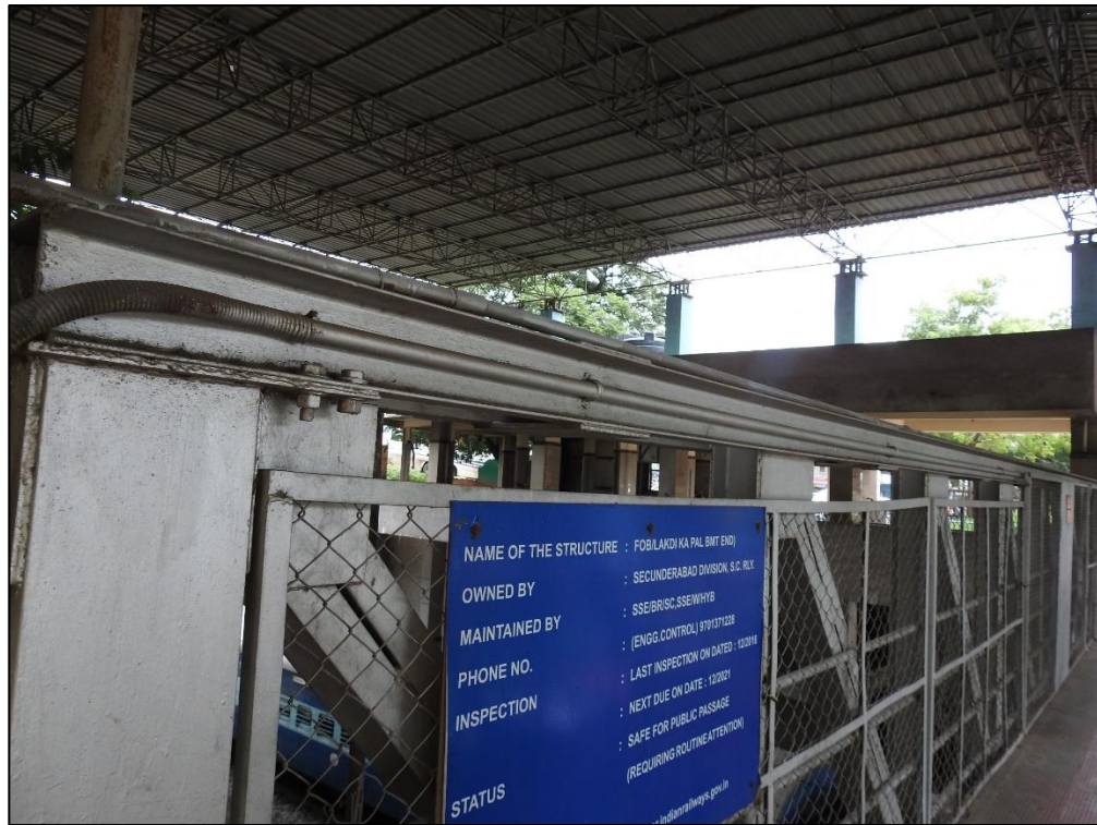
Fig 1.1: Electrical Cables and Protective screening mesh for passengers
