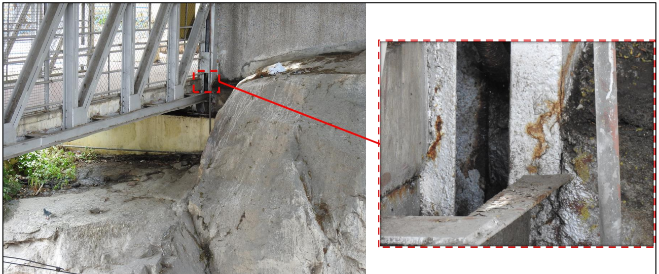
Corrosion observed in Double channel section
