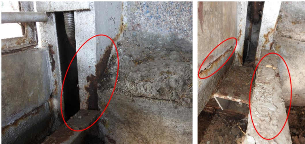
Fig 2.2: Corrosion of vertical member, gusset plate and at steel concrete joint
