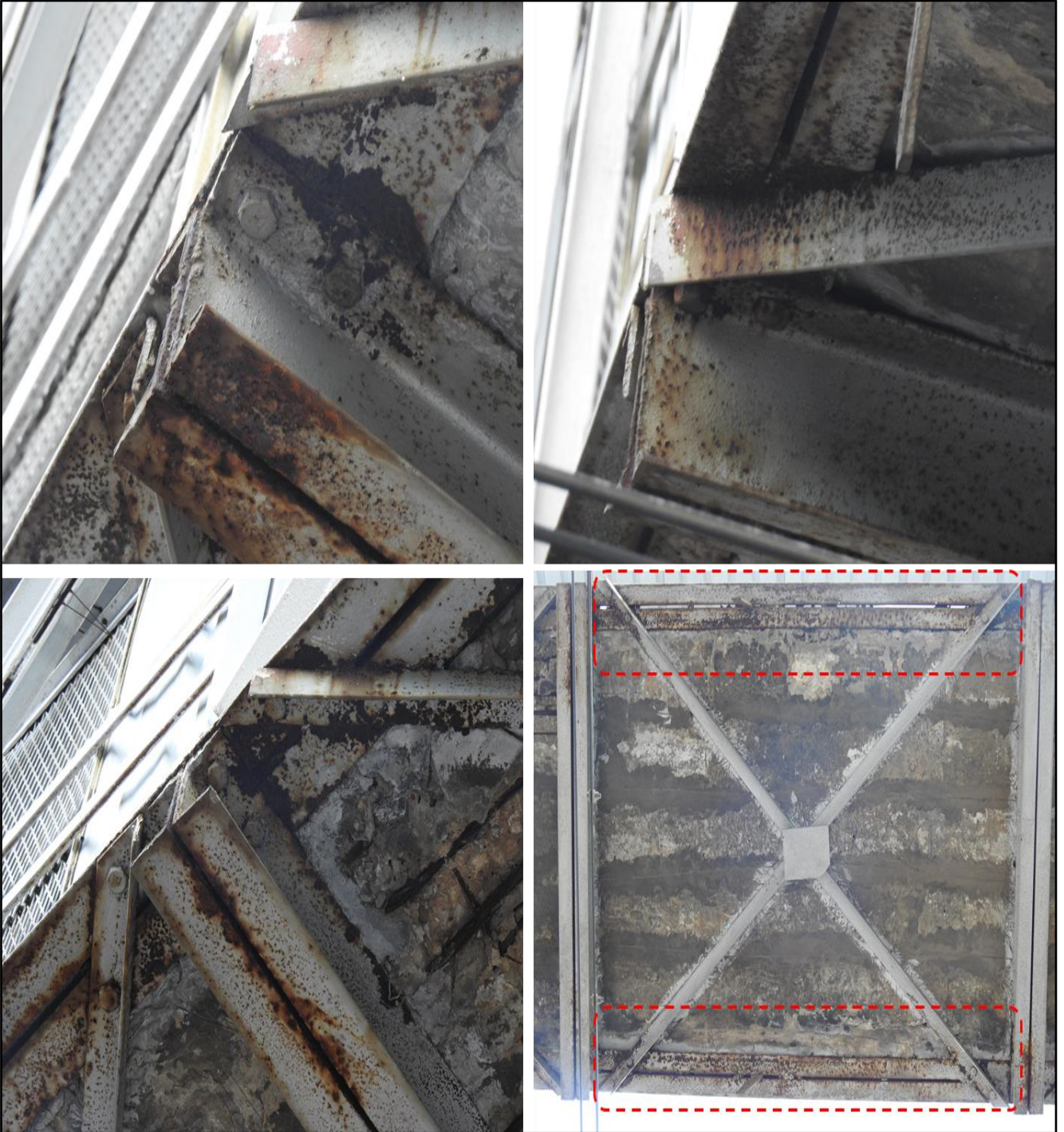
Corrosion observed in Floor beams joints
