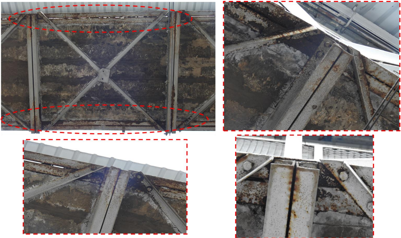
Fig: 2.2 Corroded joints and bottom chord member
