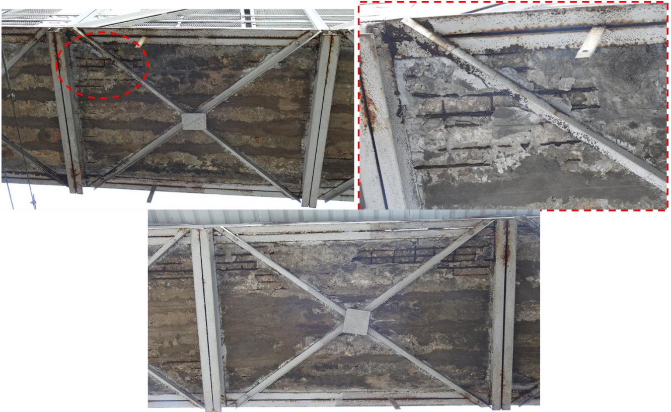
Fig: 2.5 Spalling and Reinforcement exposure at bottom of slab panels
