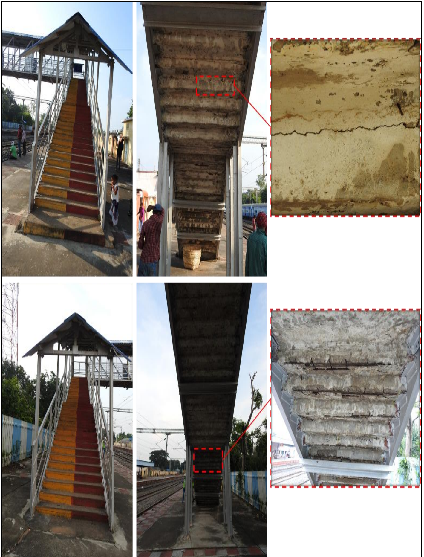
Fig 1.4: Staircase details, cracks and reinforcement exposure
