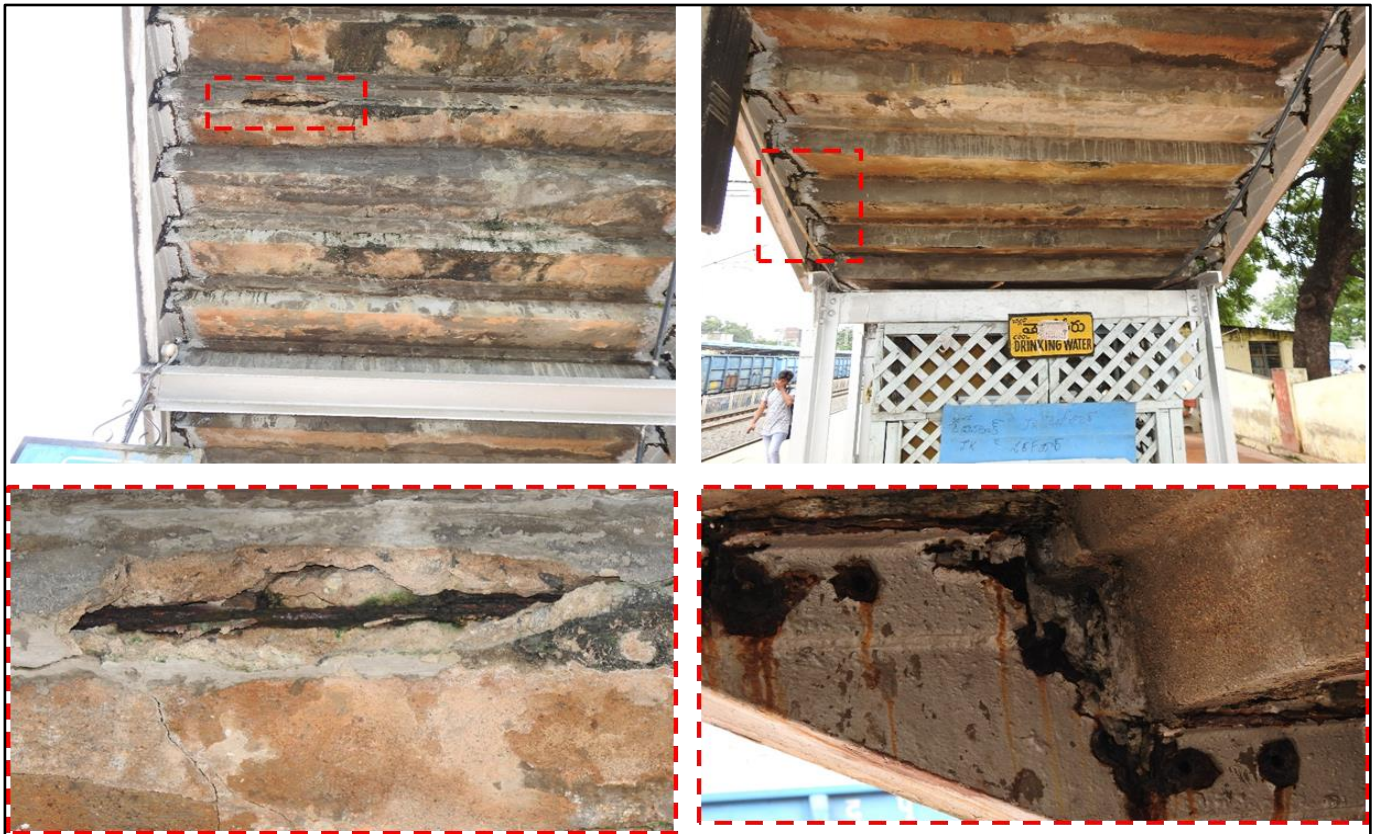
Fig 1.8: Spalling is observed in underneath of staircase
