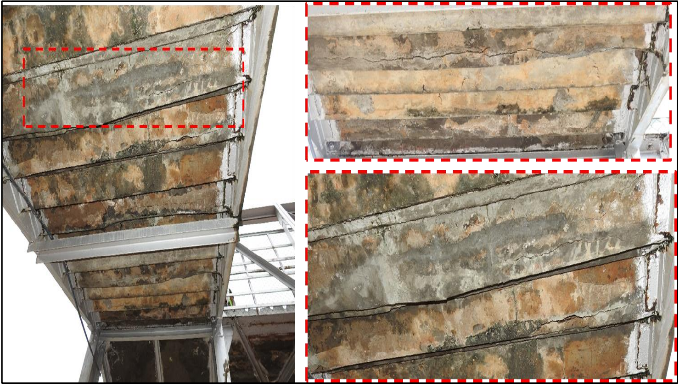
Fig 1.10: cracks are observed on landing of staircase from bottom
