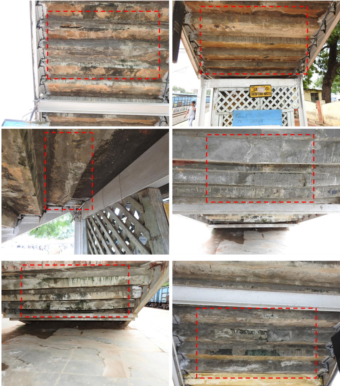
Fig 2.4: Cracking and splitting of concrete in both staircase pre-cast RCC panels
