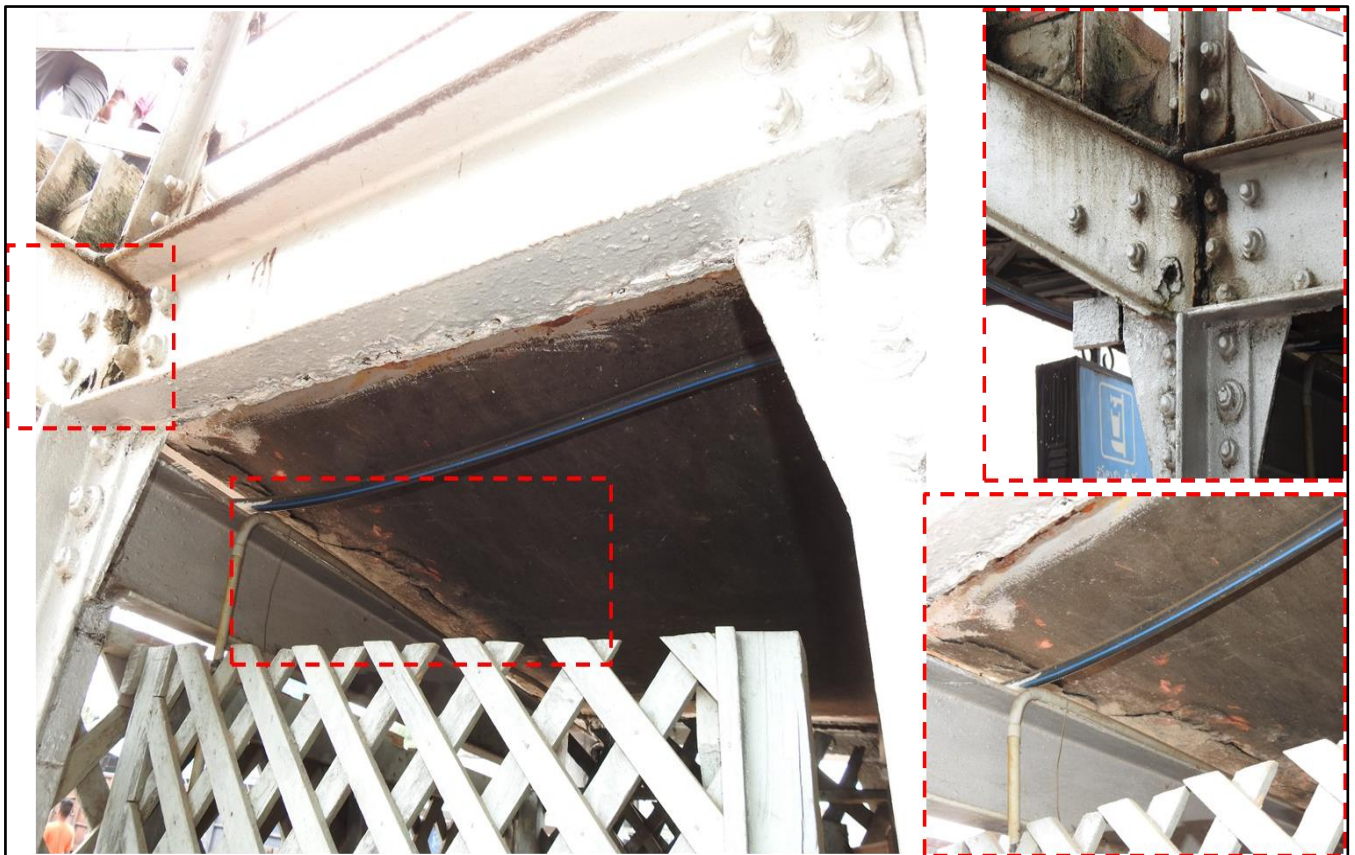
Fig 1.9: cracks are observed on landing floor slab from bottom
