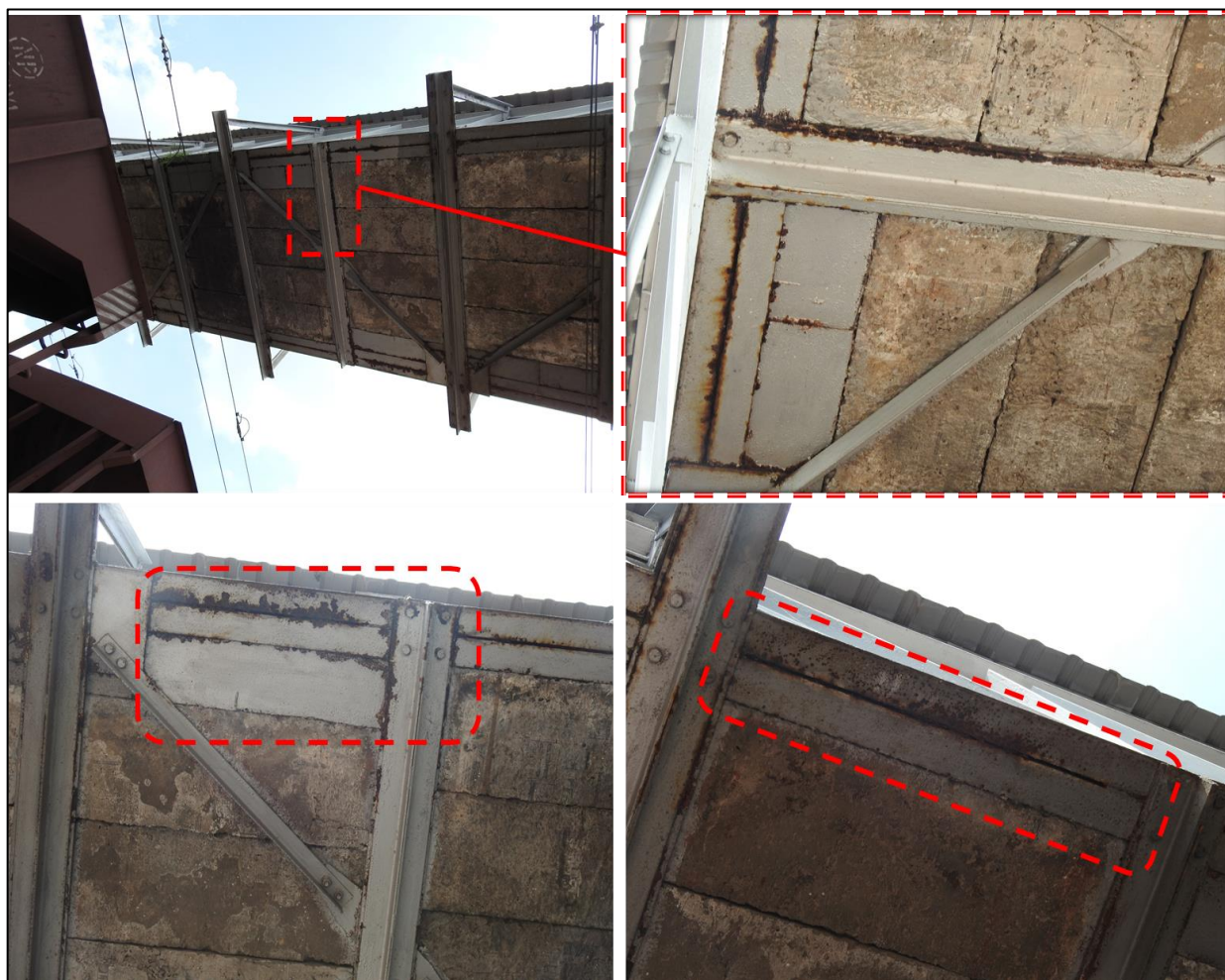
Corrosion of Floor beam and rusting of Chord members
