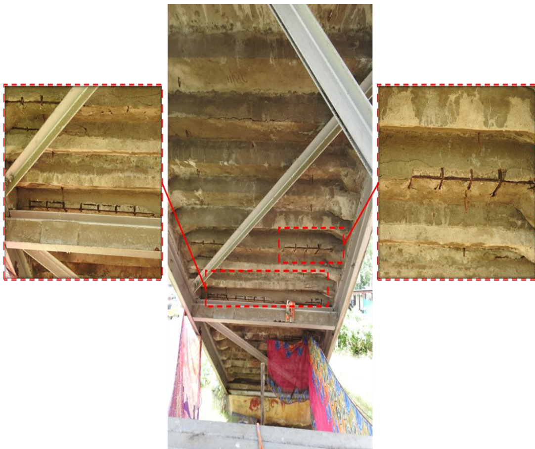
Fig 2.2: Exposed reinforcement in slab panels at circulating area staircase
