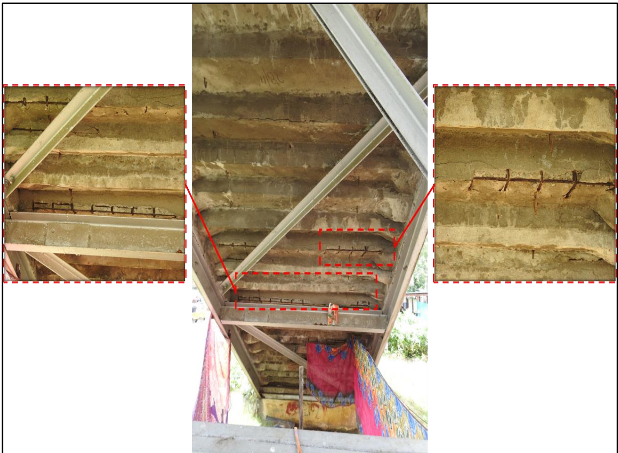
Reinforcement exposed slab panels
