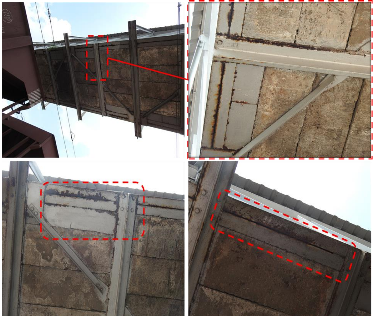
Fig 2.5: Corrosion of floor beams and bottom chord member in span-2
