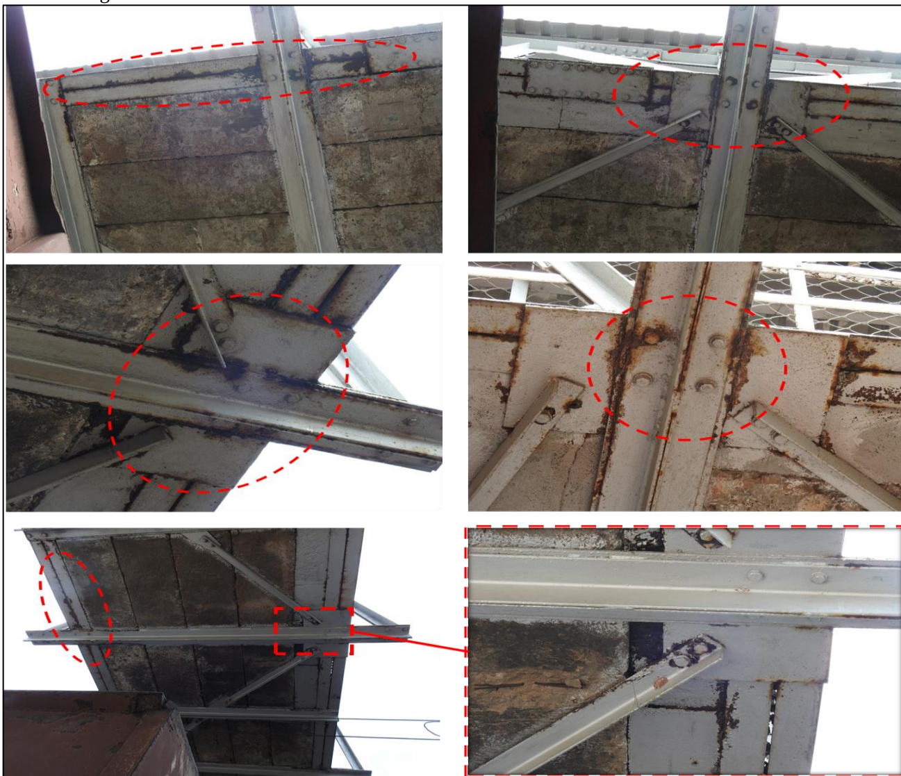
(a) Corrosion in gusset plate joints and bottom main chord double angle section
