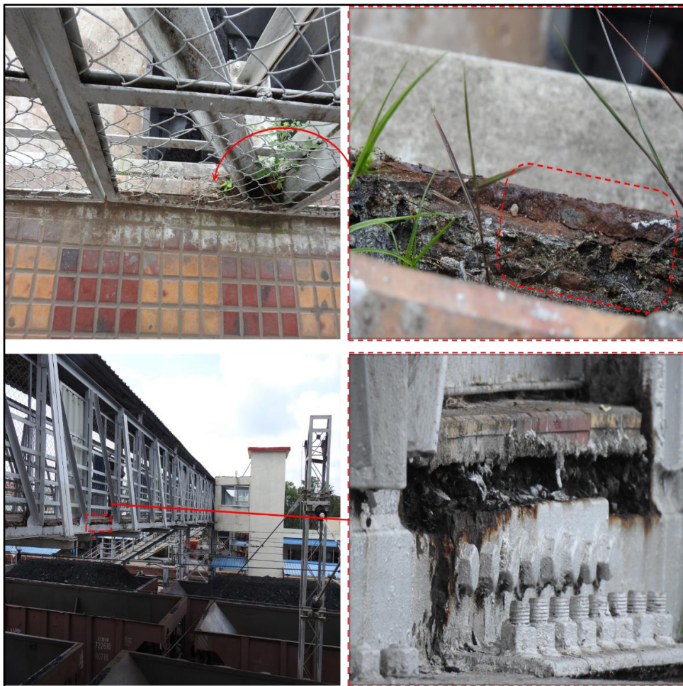
Fig 1.6: Corrosion is also observed at steel concrete joint
