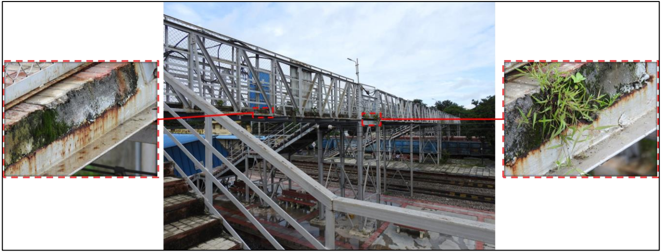
Fig 1.7: Corrosion and vegetation
