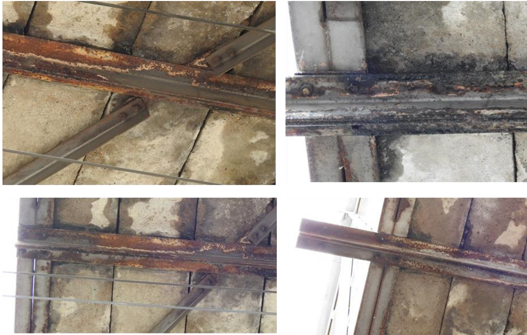
Fig 2.10: Locations of deterioration of bolted connections in span 3
