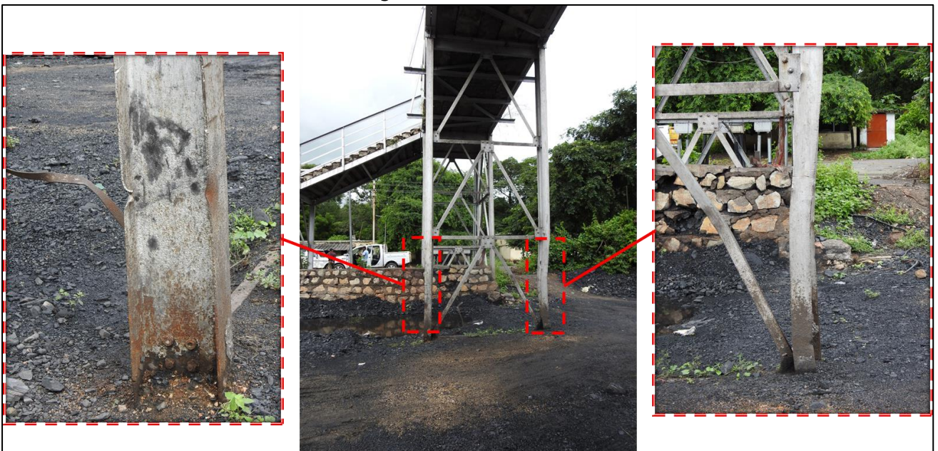
Fig 1.6: Accidental damage observed at stanchions
