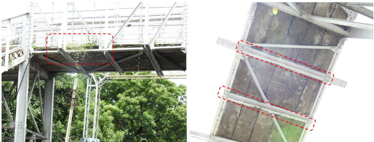
Fig 2.16: vegetation and slight corrosion at floor beam
