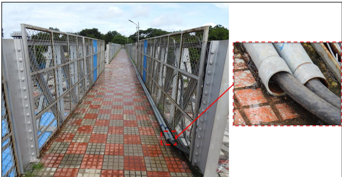
Fig 1.1: Cables, Flooring and protective screen
