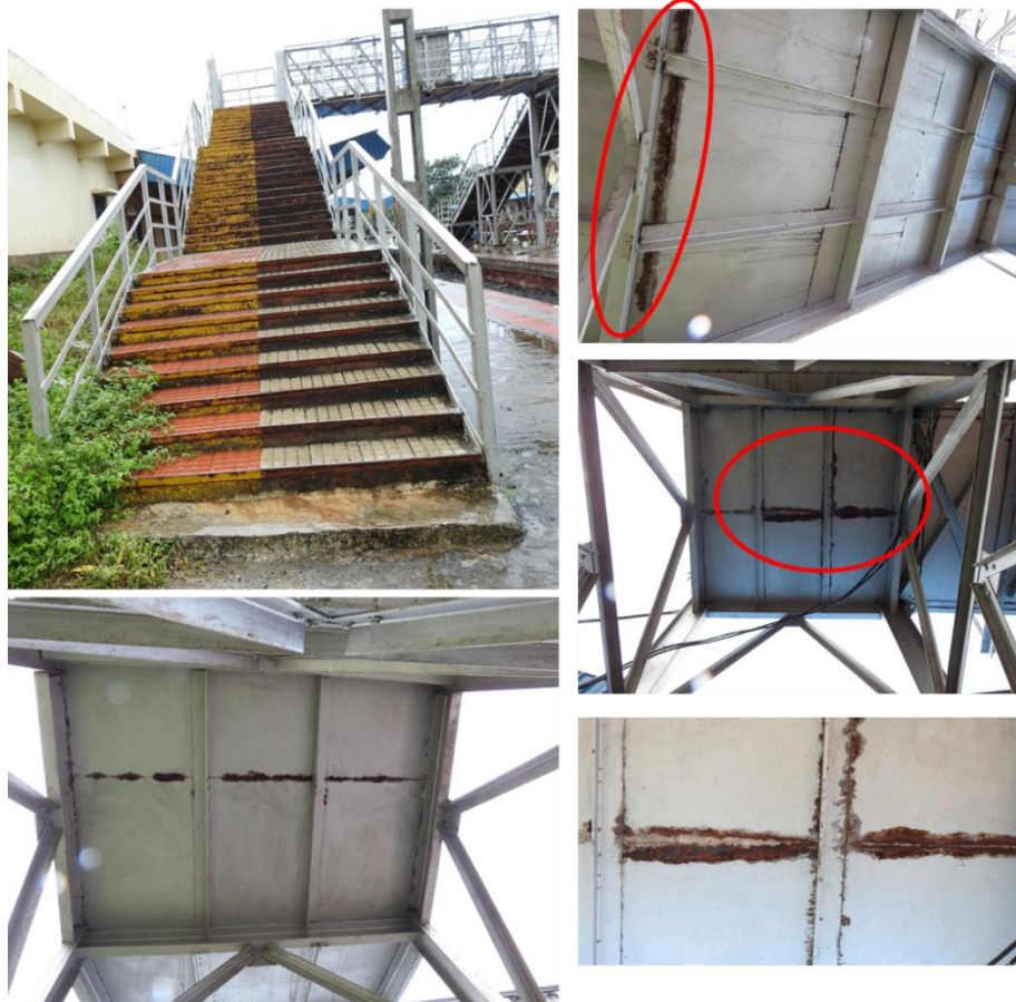
Fig 2.2: Locations of deteriorations in Staircase 1 from bottom
