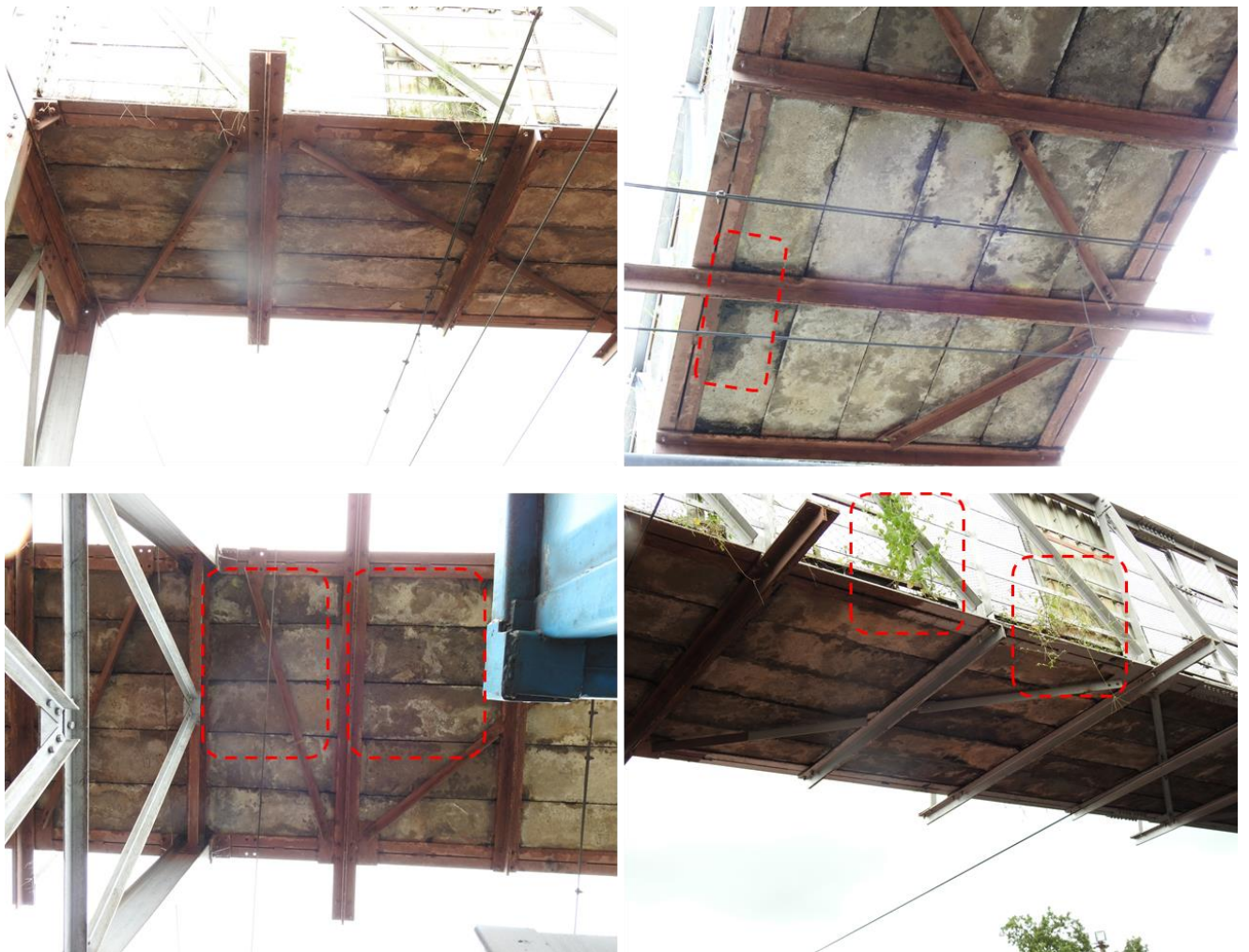
Fig 2.12: Locations of corrosion and vegetation in span 4
