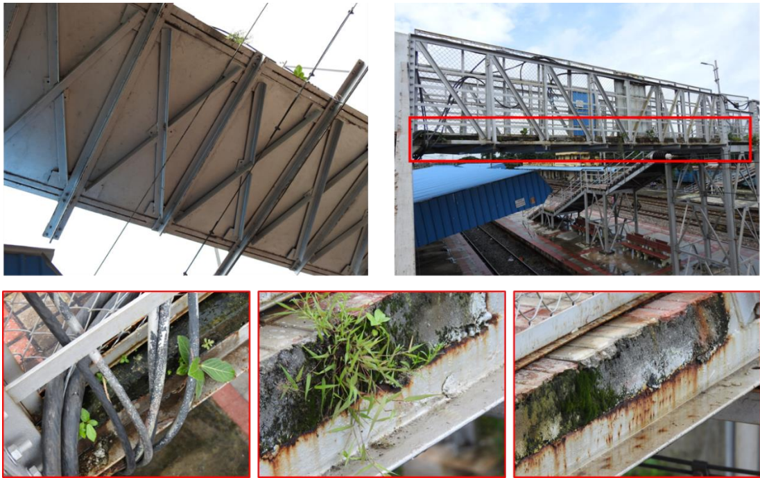
Fig 2.3: Deteriorations of bottom chord and Vegetation at deck level
