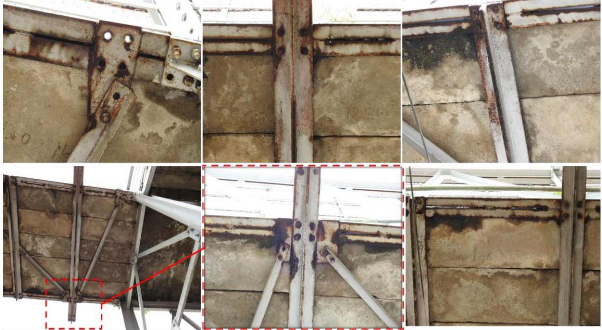
Reinforcement exposed and leaching of slab panels
