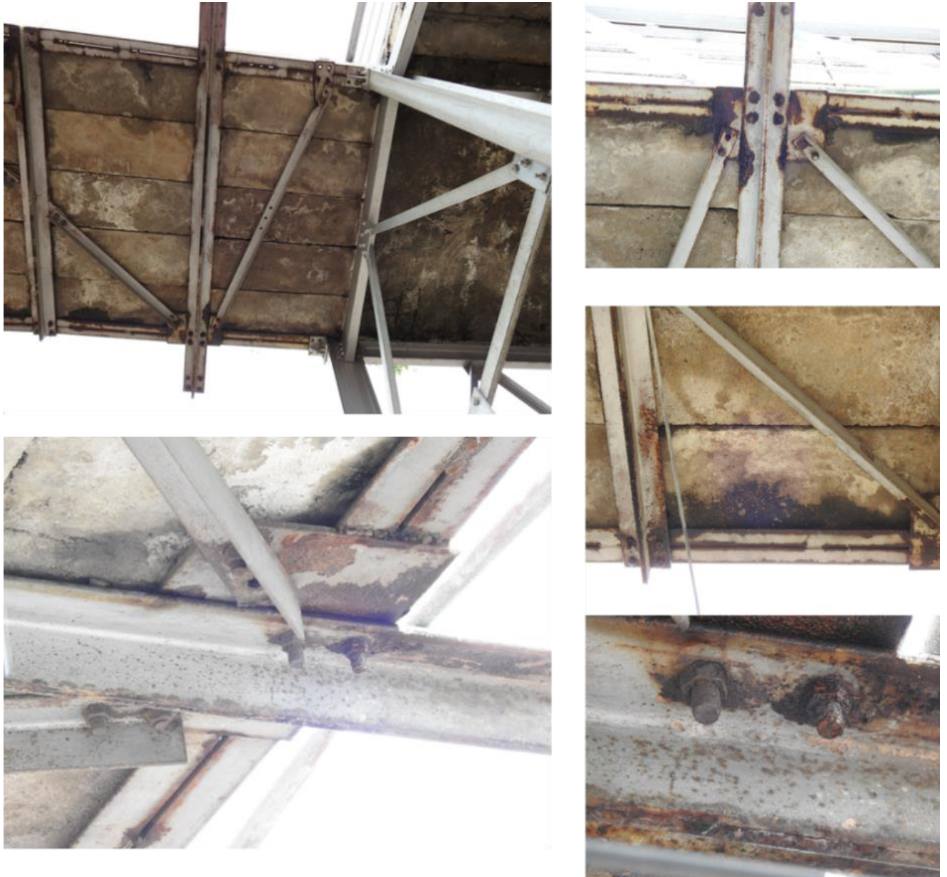
Fig 2.6: Deterioration locations of steel members at slab deck level in span 2
