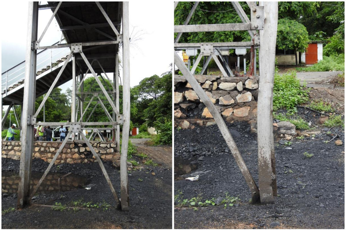
Fig 2.17: Deformed column due to accidental hitting
