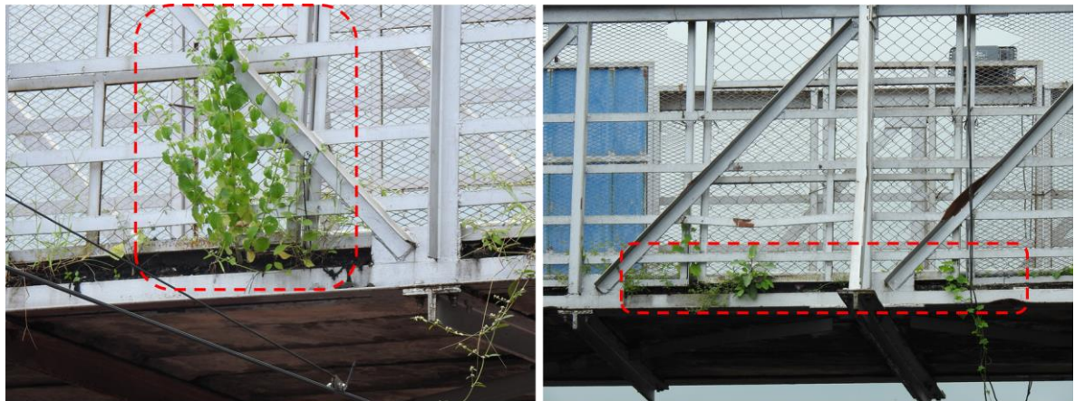
Fig 2.14: vegetation observed near bottom chord member
