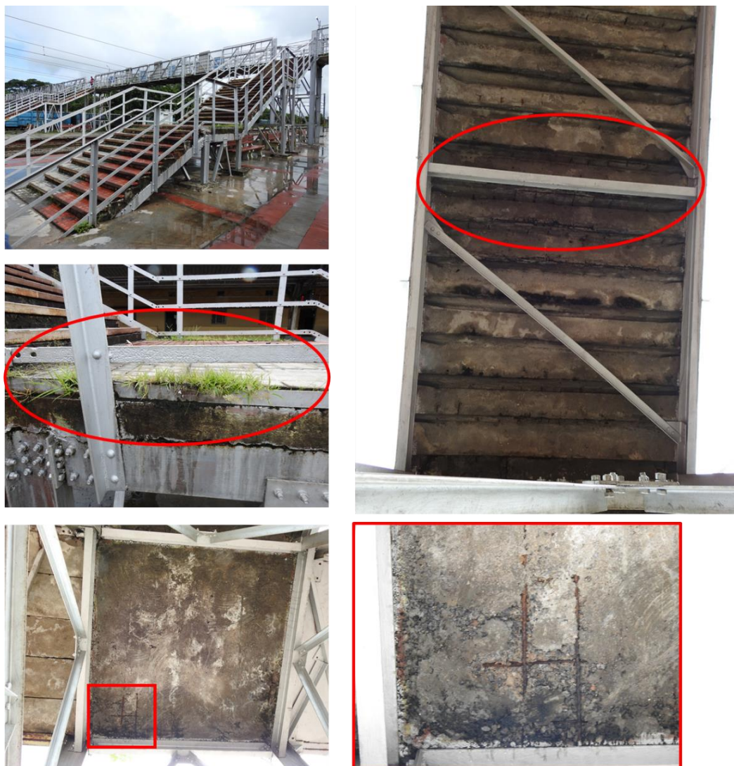
Fig 2.4: Locations of Deteriorations in Staircase 2 from bottom
