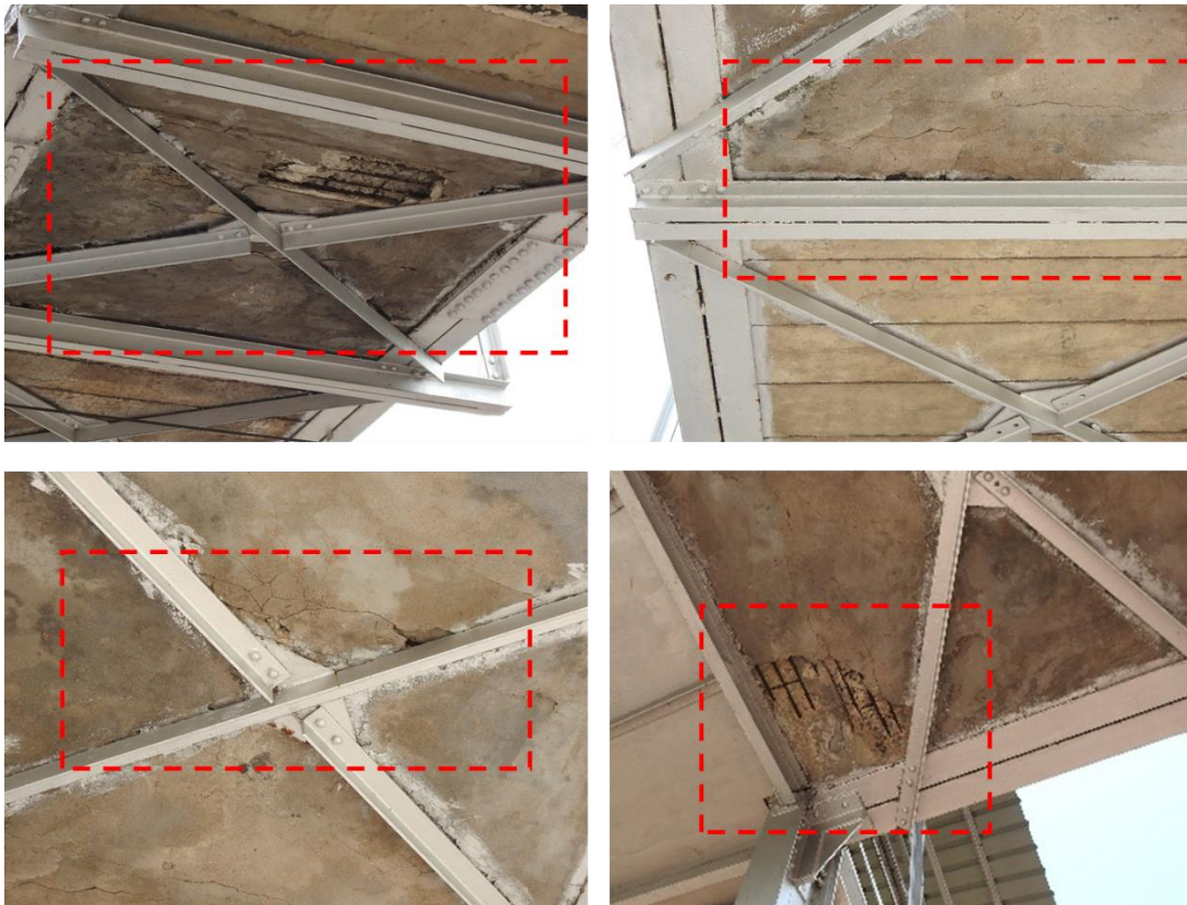
Fig 2.3: Surface cracks and spalling are observed in repaired slab
