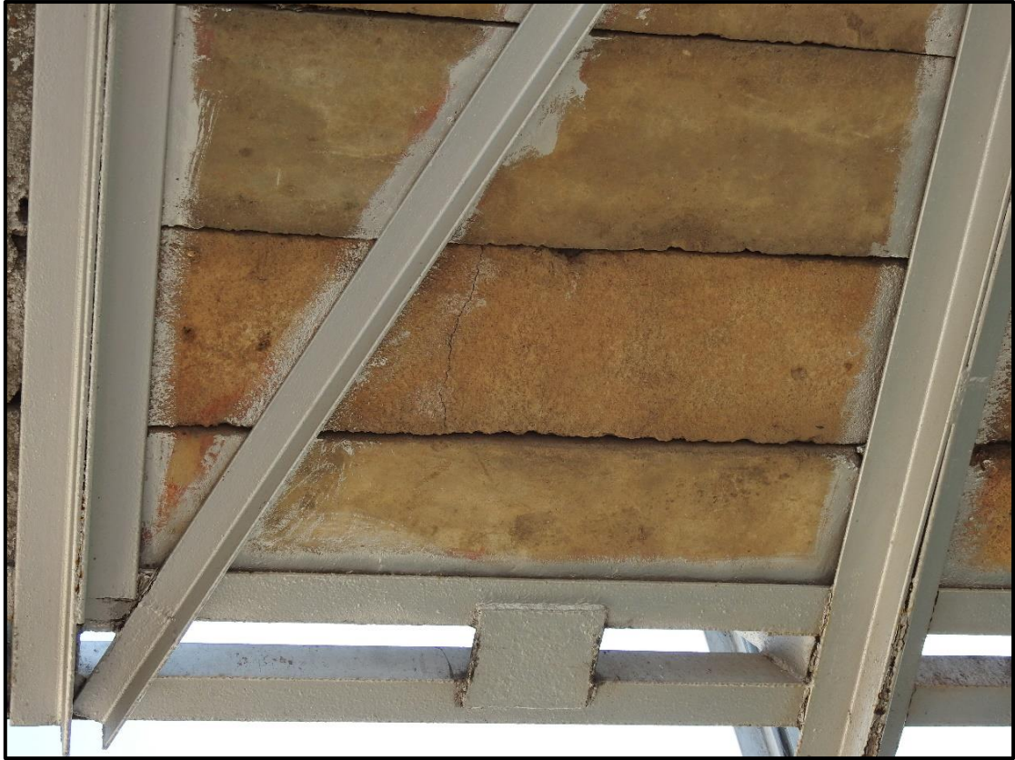
Fig 1.6: Cracks are observed in Pre-cast RCC slab panels (bottom view)
