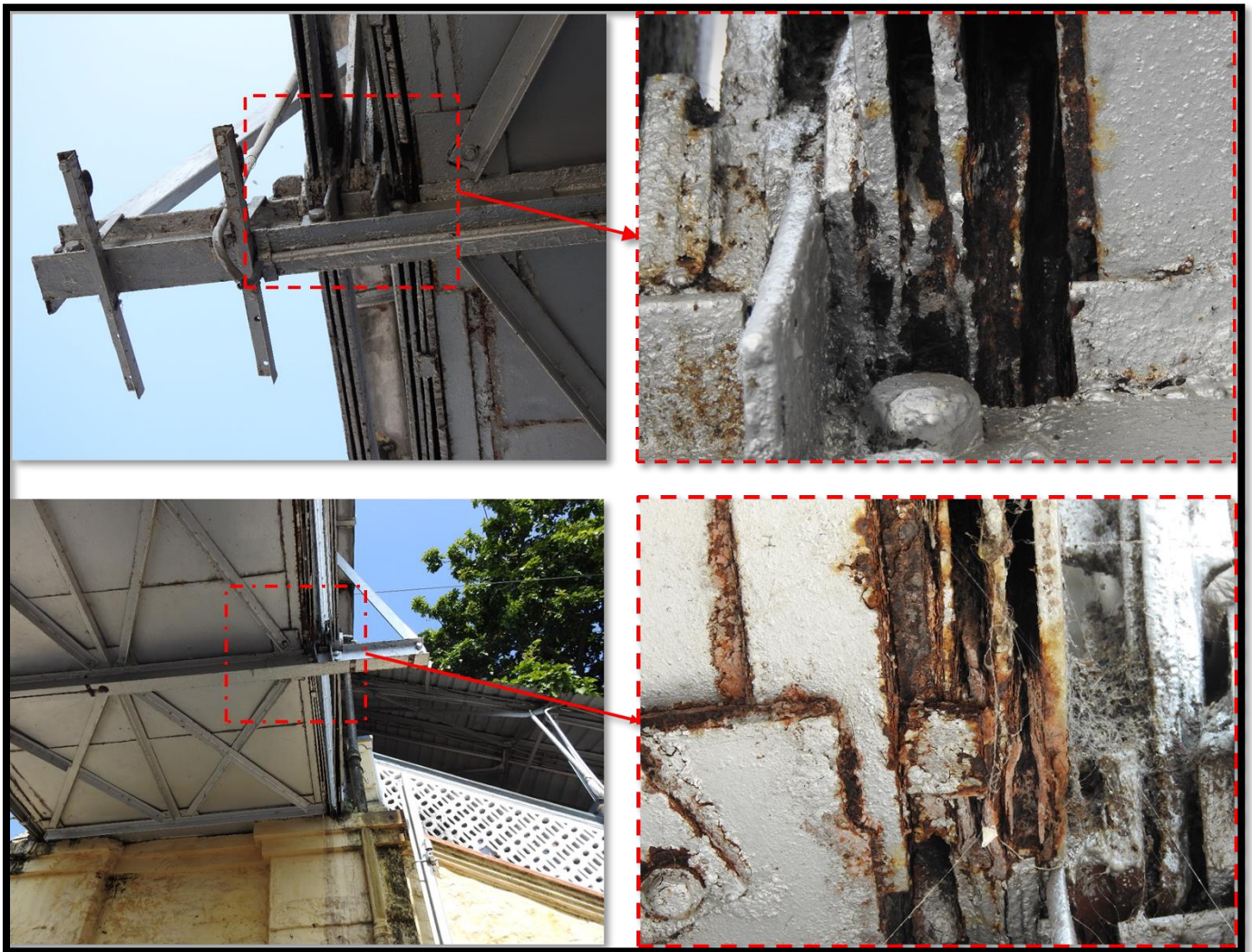
Fig 1.6: Severe corrosion in main plates at bottom of FOB.
