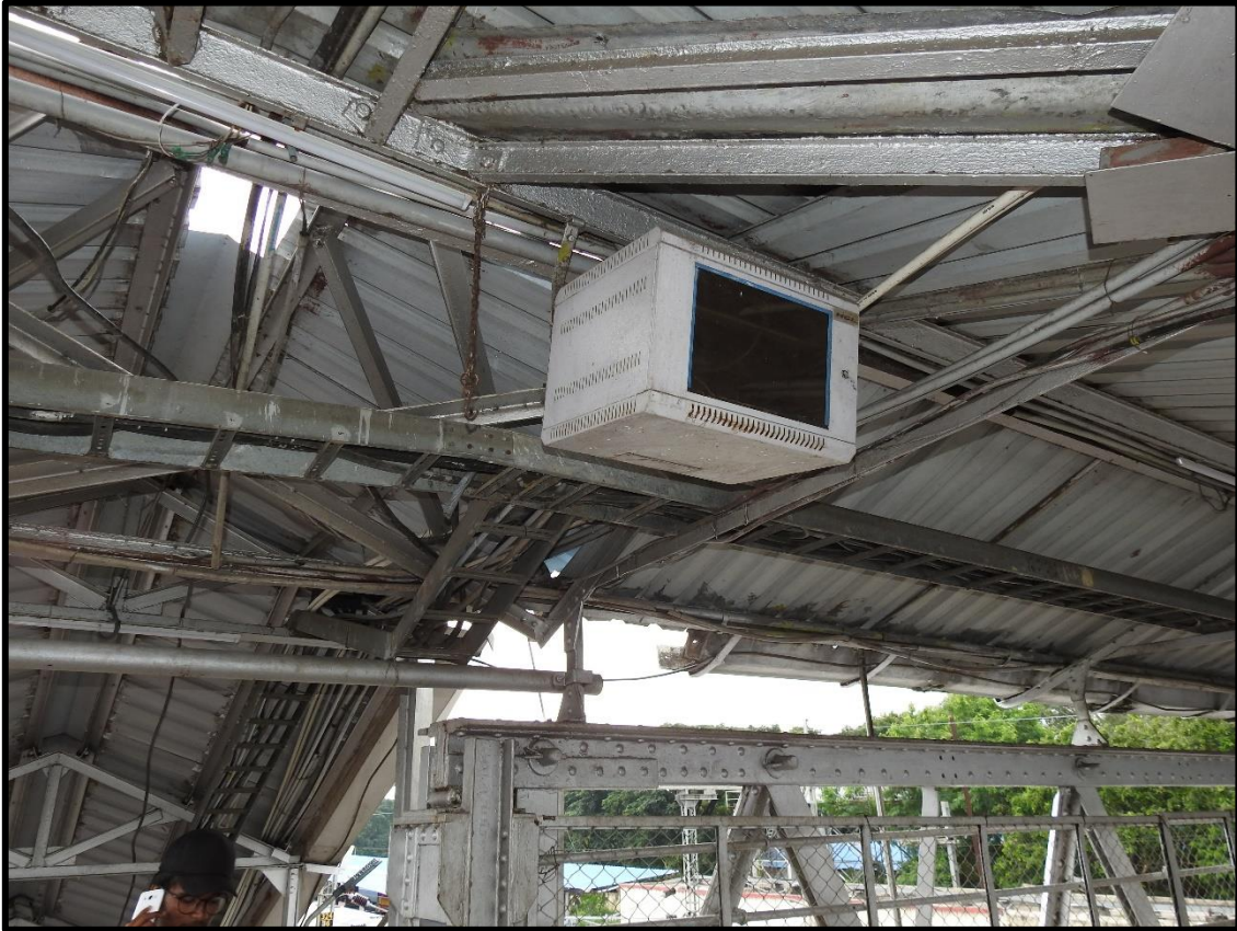
Fig 1.3: Rail Wi-Fi unit supported on roof truss
