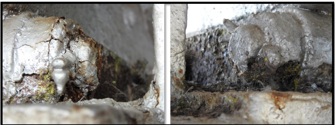
Fig 1.8: Corrosion of rollers near staircase 3
