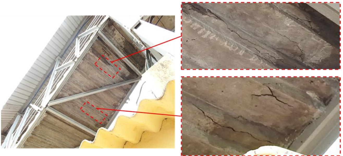
Fig 2.8: Cracks are observed in staircase-1 panels
