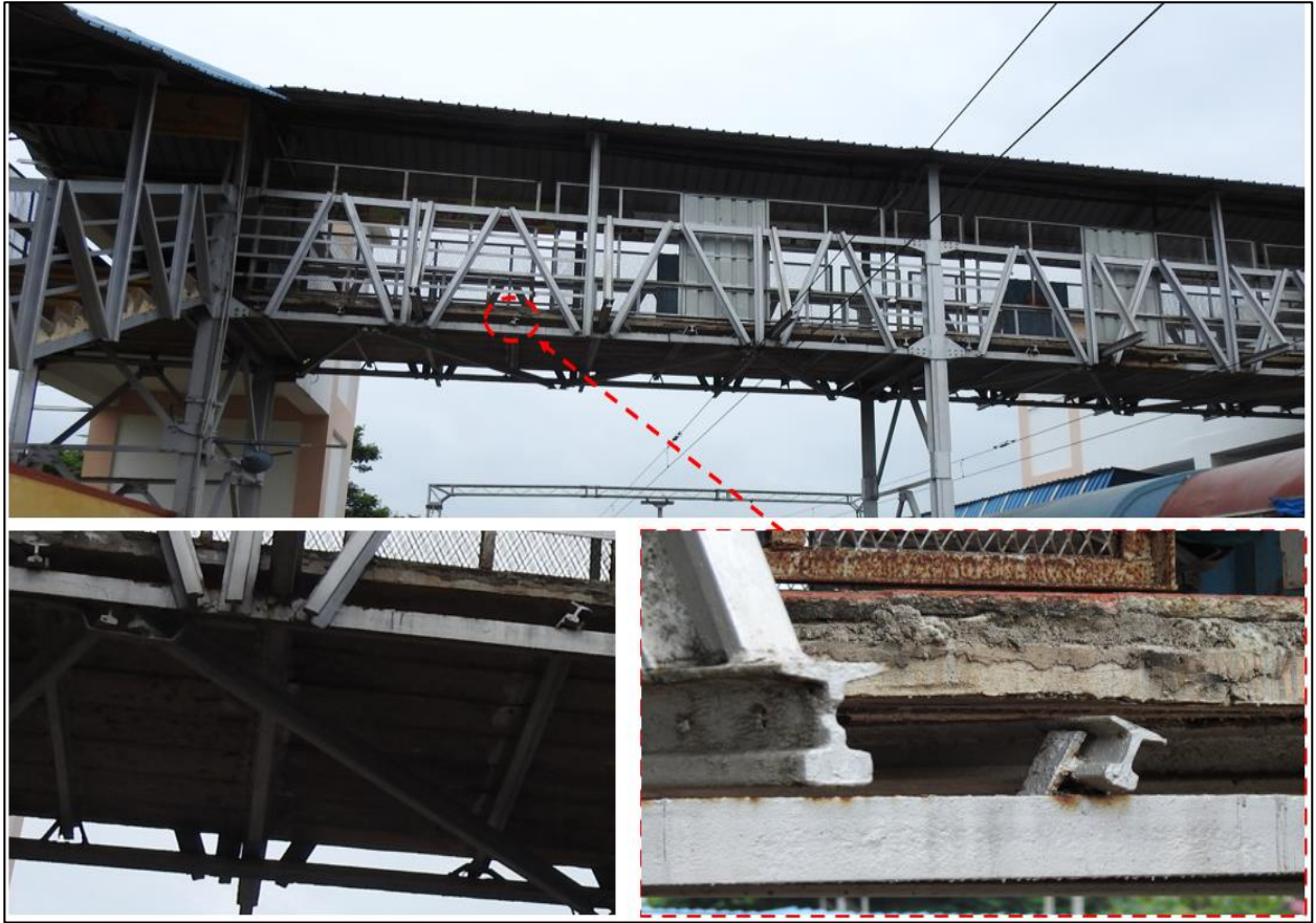
(a) Deformations in floor beam of span 1
