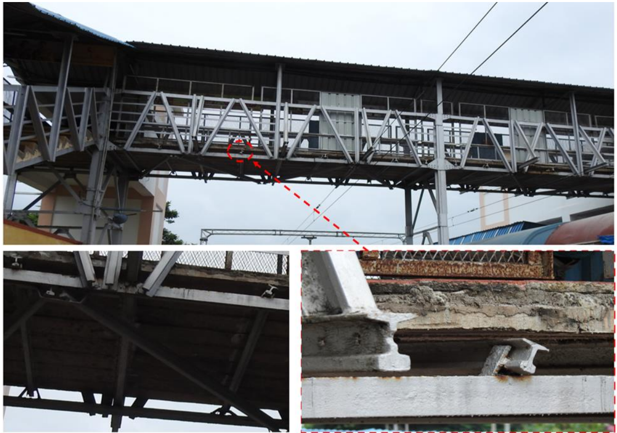
Fig 2.5: Deformation in floor beam connecting bottom chord
