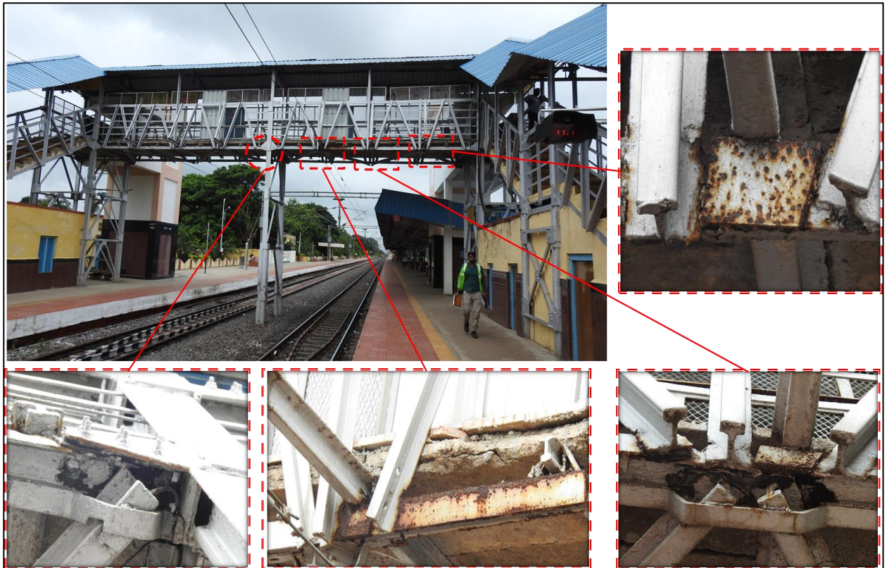
(b) Corrosion observed at Bottom chord and bracings joints.
