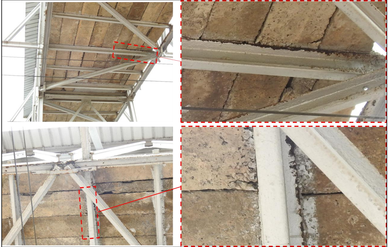
(a) Corrosion observed at floor beams
