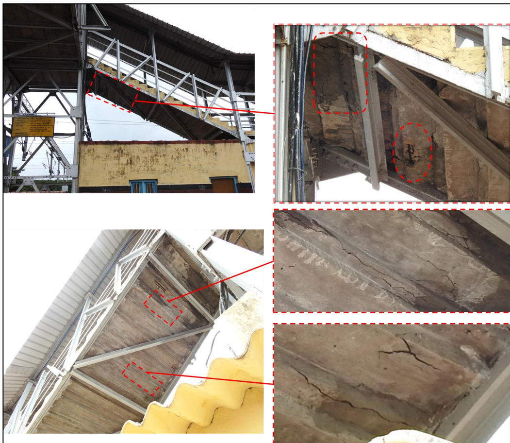
(b) Exposed reinforcement and cracks in staircase panels
