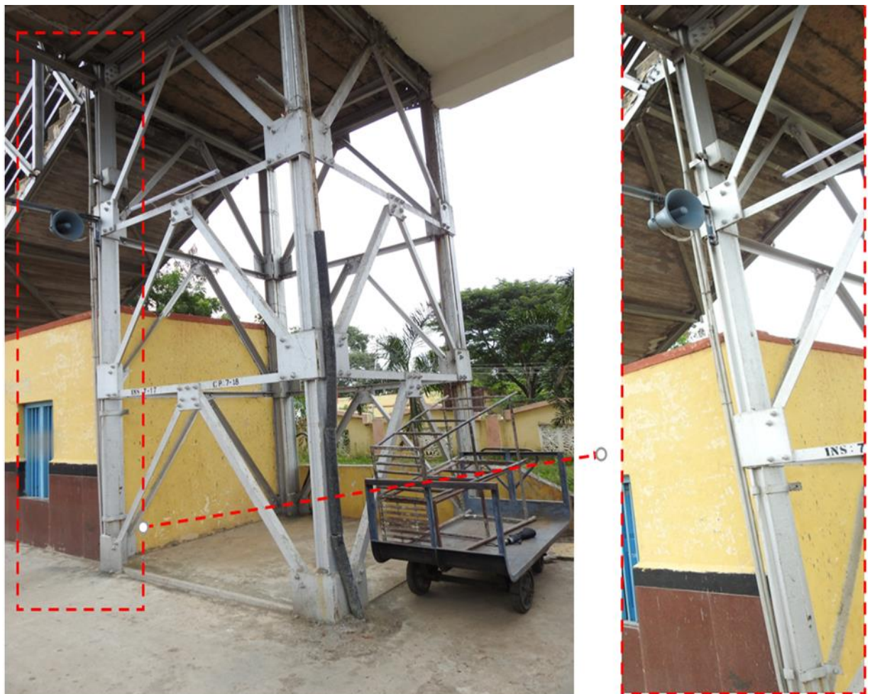
Fig 2.6: deformation in trestle at staircase-1
