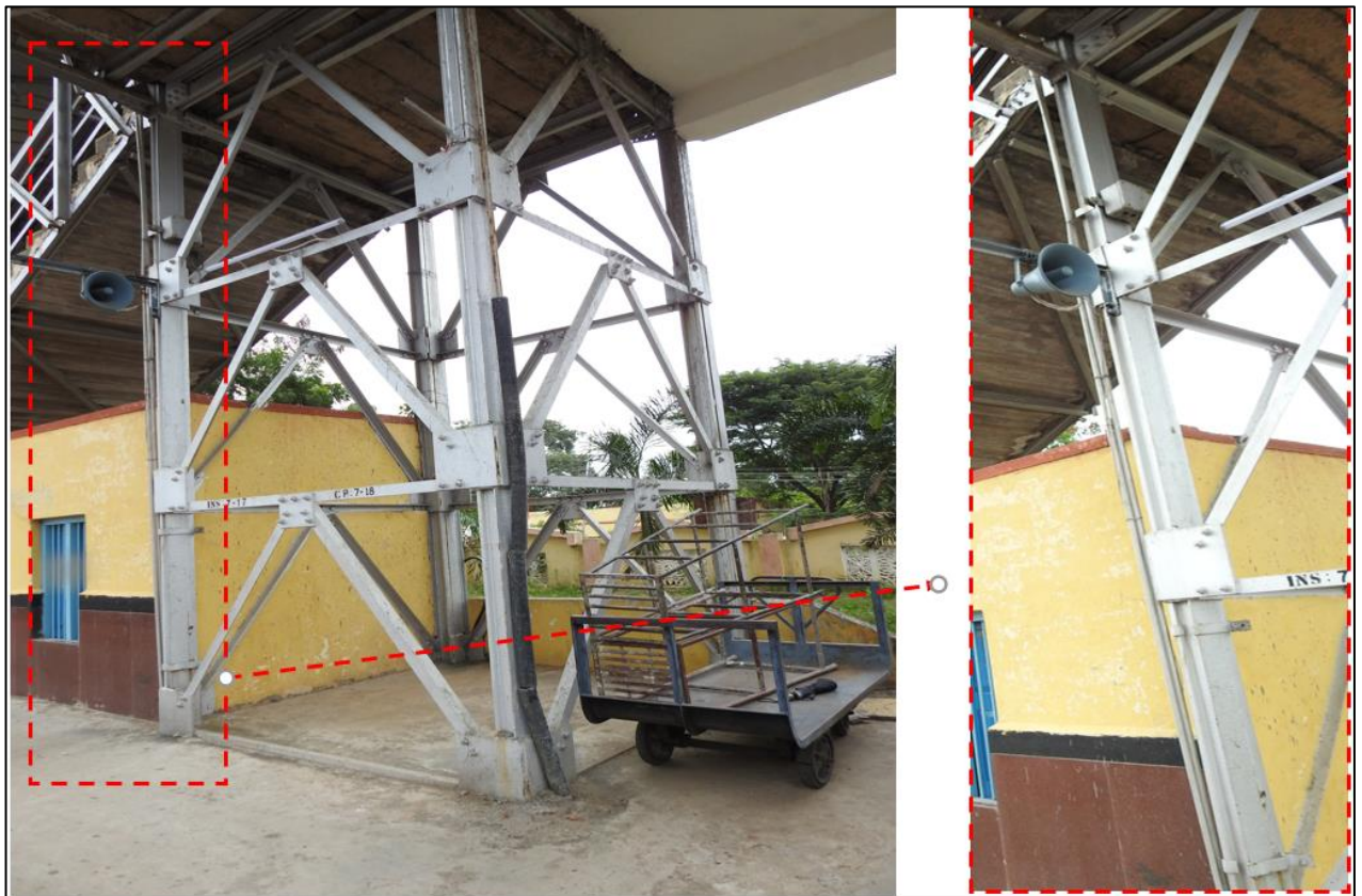
(b) Deformation observed in Trestle-1 column
