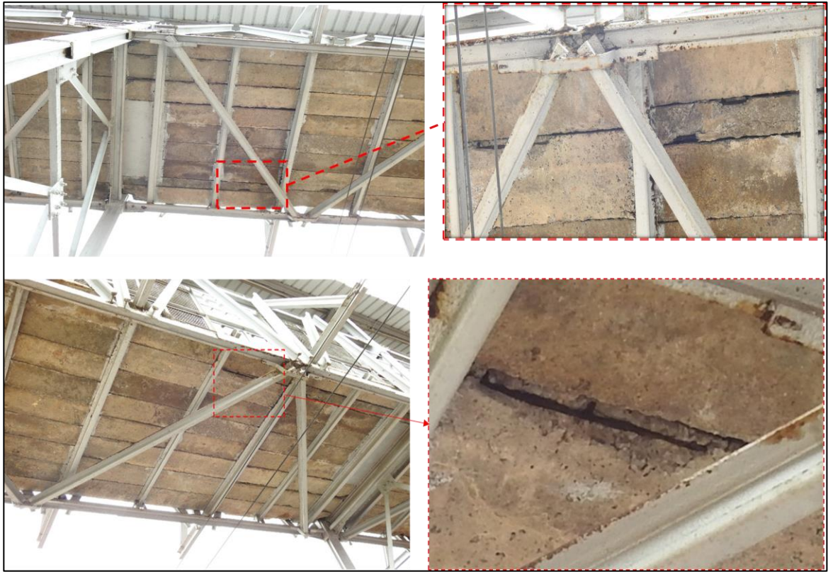
(a) Exposed reinforcement and corrosion of rebar
