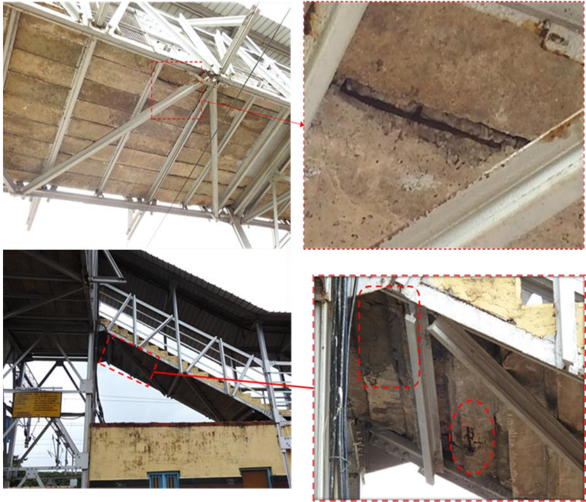
Fig 2.11: Reinforcement exposed in panels
