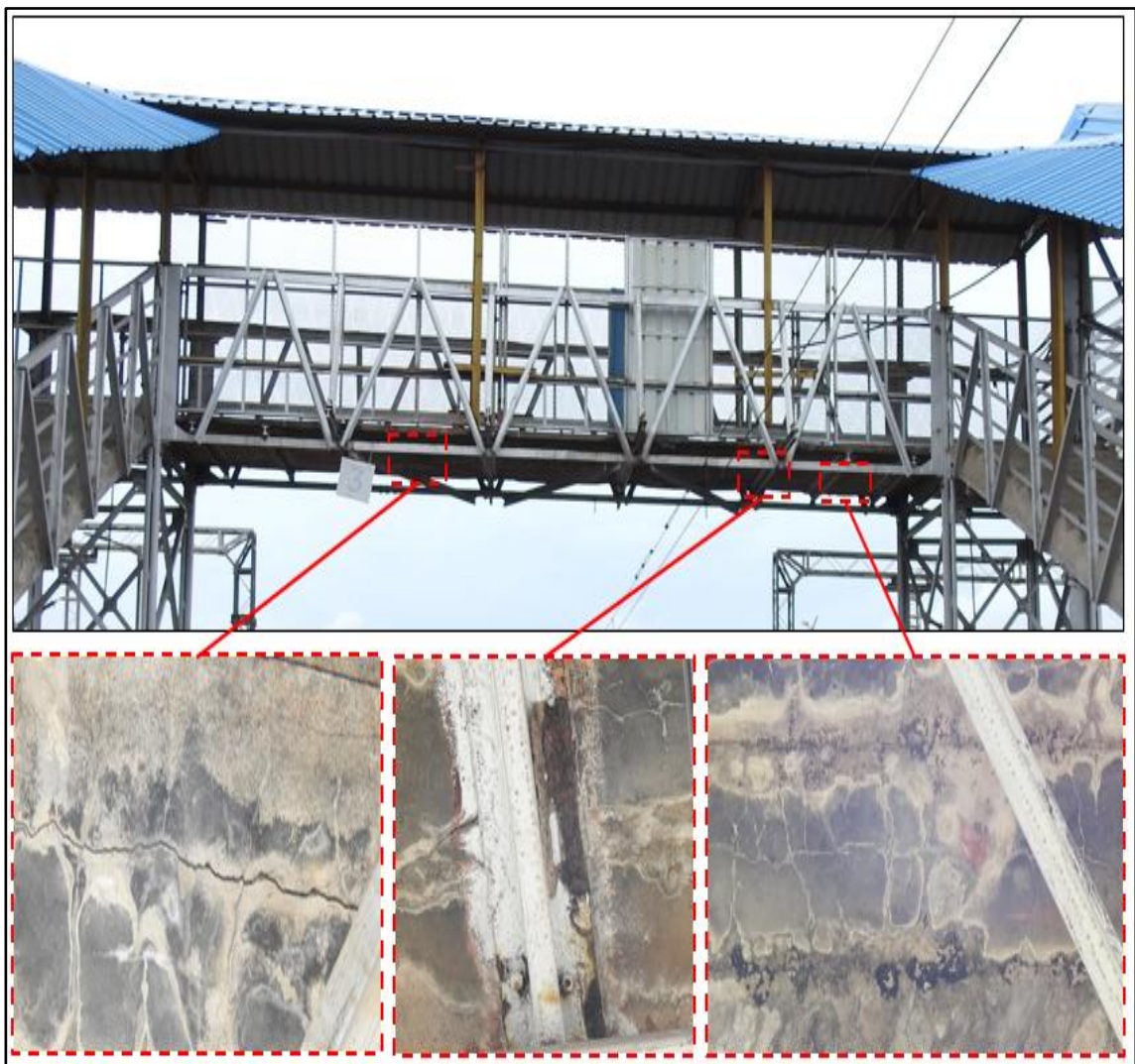
e) Cracks, Corrosion and Leaching at slab panels on Span-3
