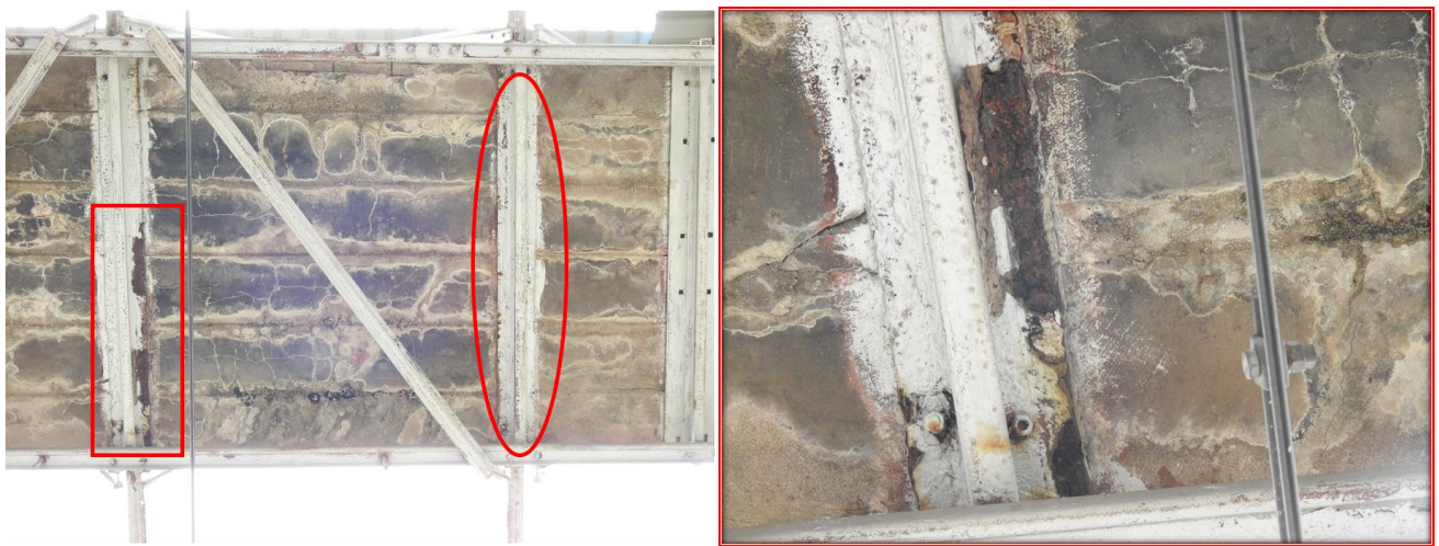
Fig 2.8: Corrosion of floor beam members in span-3
