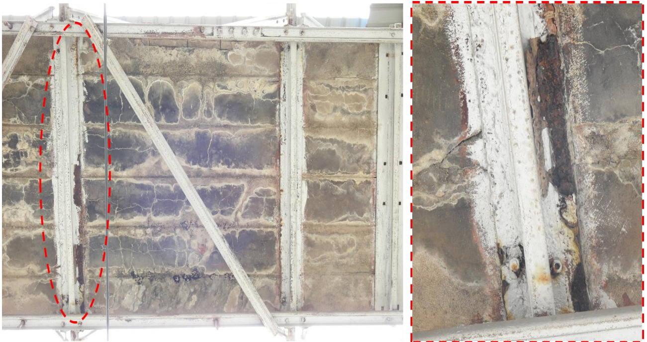
Fig 2.2: Corrosion of floor beam members in span-1
