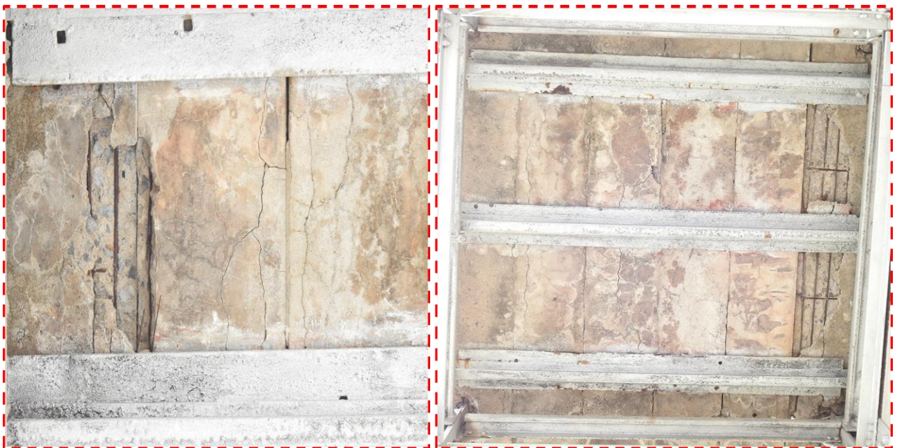
Fig 2.3: Exposed reinforcement at main landing in staircase-1
