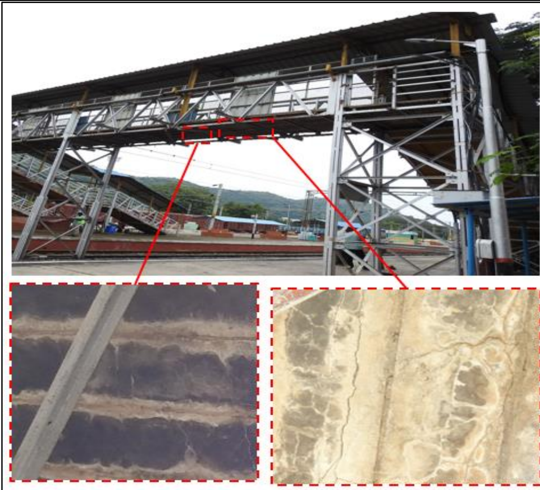
b) Cracks and Leaching at slab panels on Span-1
