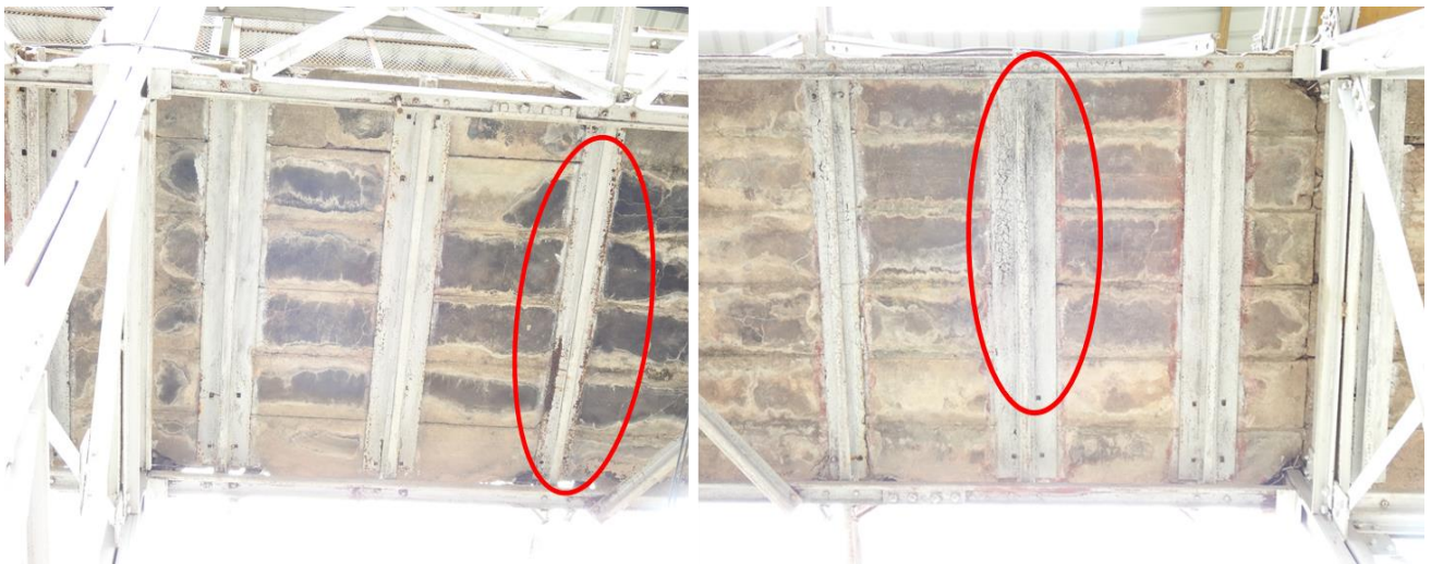
Fig 2.5: Corrosion of floor beam members in span-2
