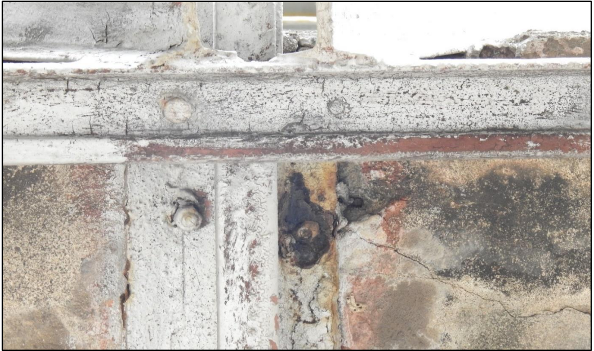
f) Corrosion observed at Floor beam and bottom chord bolt connection
