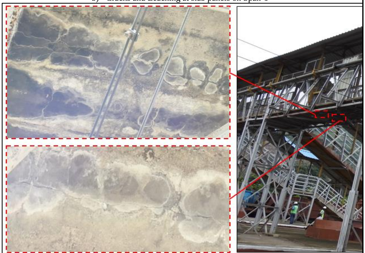
c) Corrosion observed at floor beams and bottom chord on Span-2
