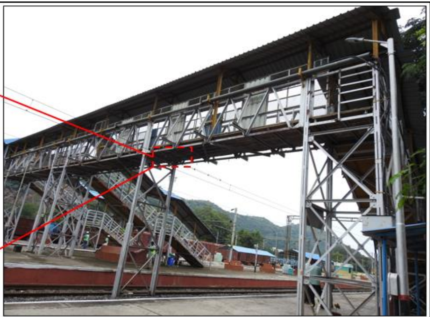
a) Corrosion observed at floor beams on Span-1
