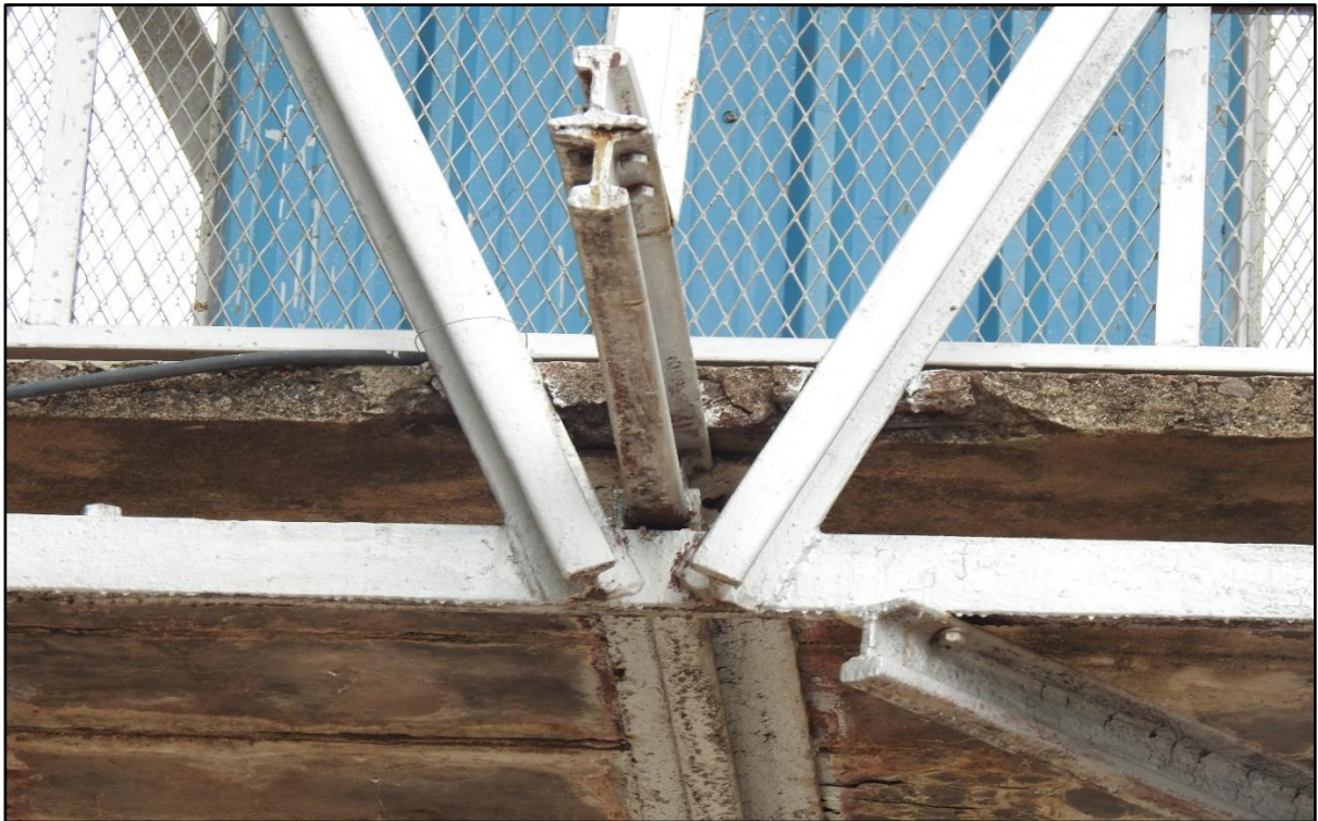
g) corrosion observed at Floor beam and bottom chord
