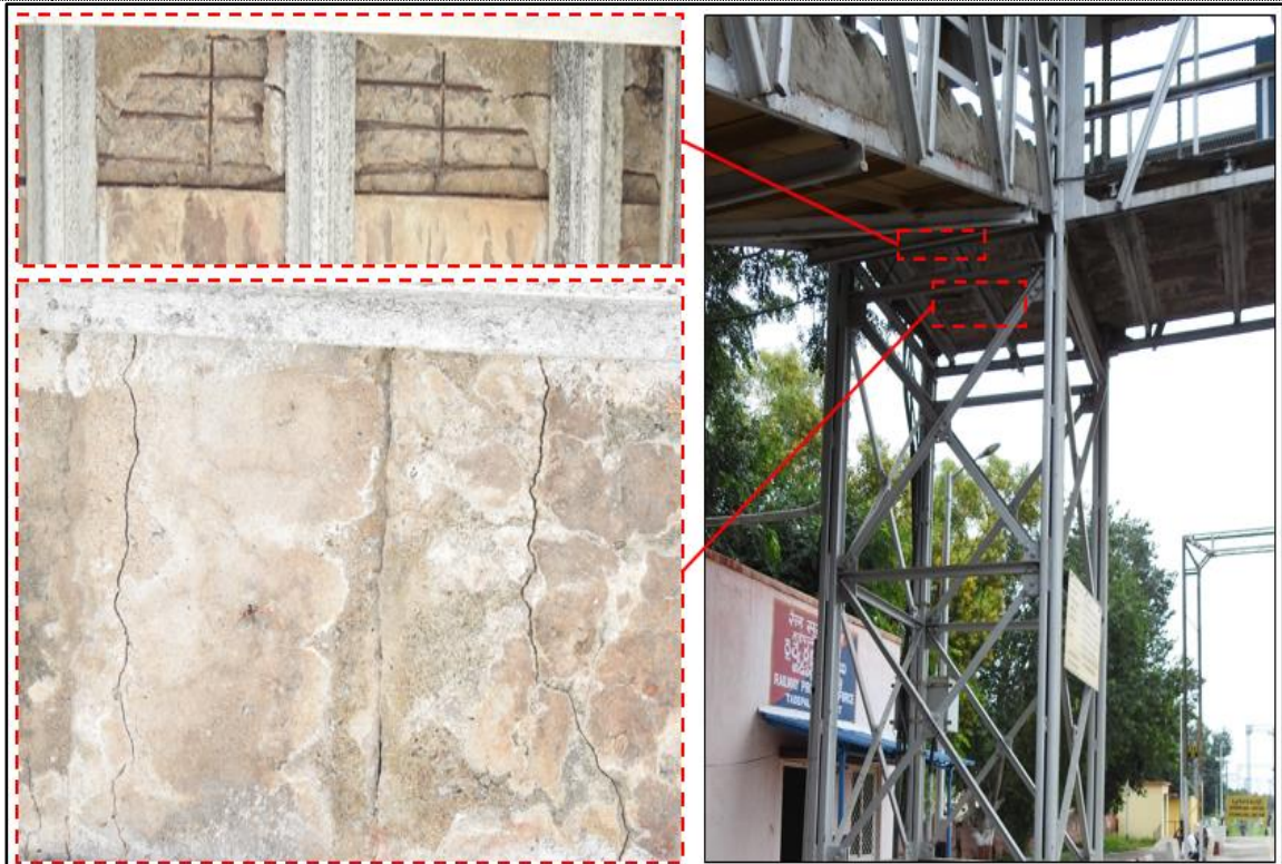
a) Reinforcement exposed and cracks on bottom of slab panels (Staircase 1 Main landing)
