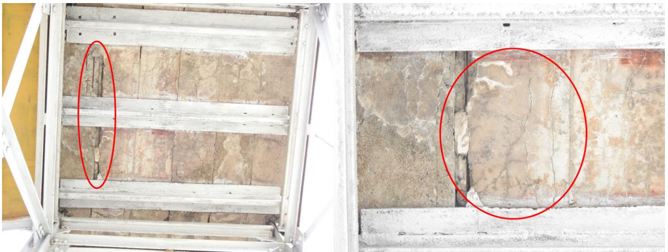
Fig 2.6: Exposed reinforcement at main landing in staircase-2
