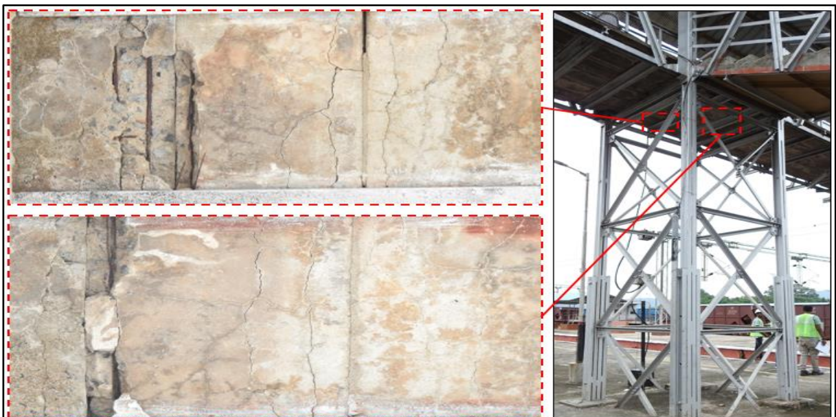
b) Reinforcement exposed and cracks on bottom of slab panels (Staircase 2 - Main landing)
