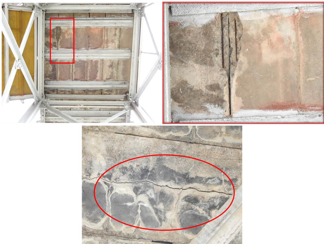
Fig 2.9: Exposed reinforcement at main landing and cracks in pathway slab panels in staircase-3
