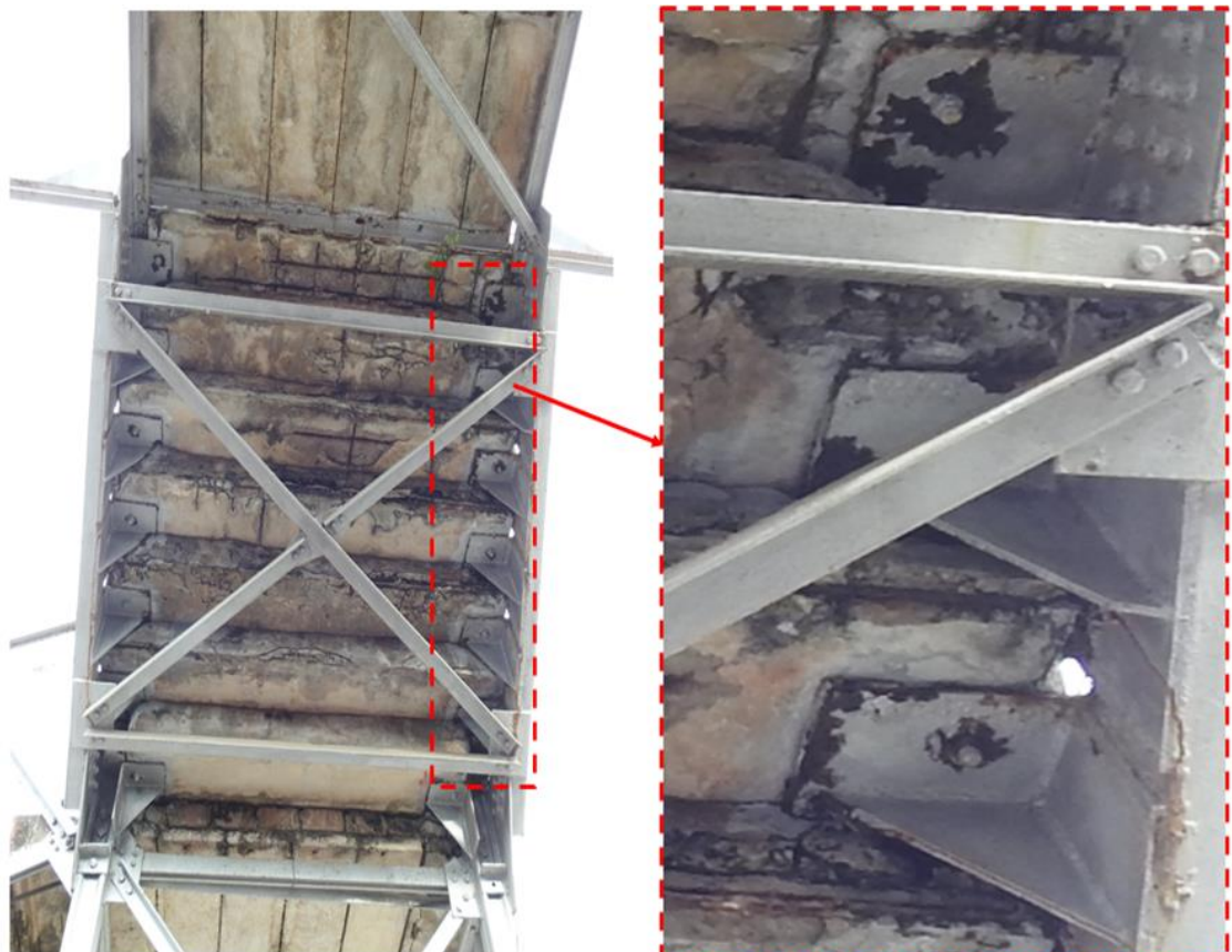
Fig: 2.7 severely deterioration of cleat angle supporting staircase panels
