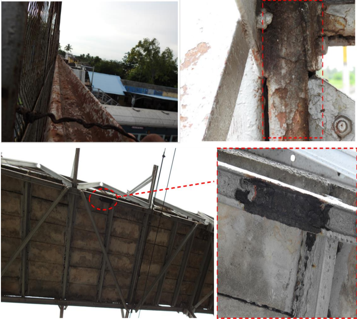
Fig: 2.4 corrosion in top and bottom chord
