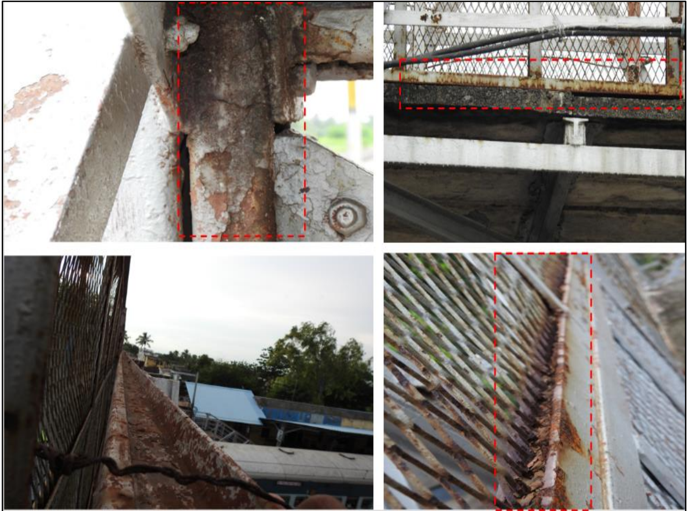
Fig 1.3: Corrosion observed at steel joint & Top chord
