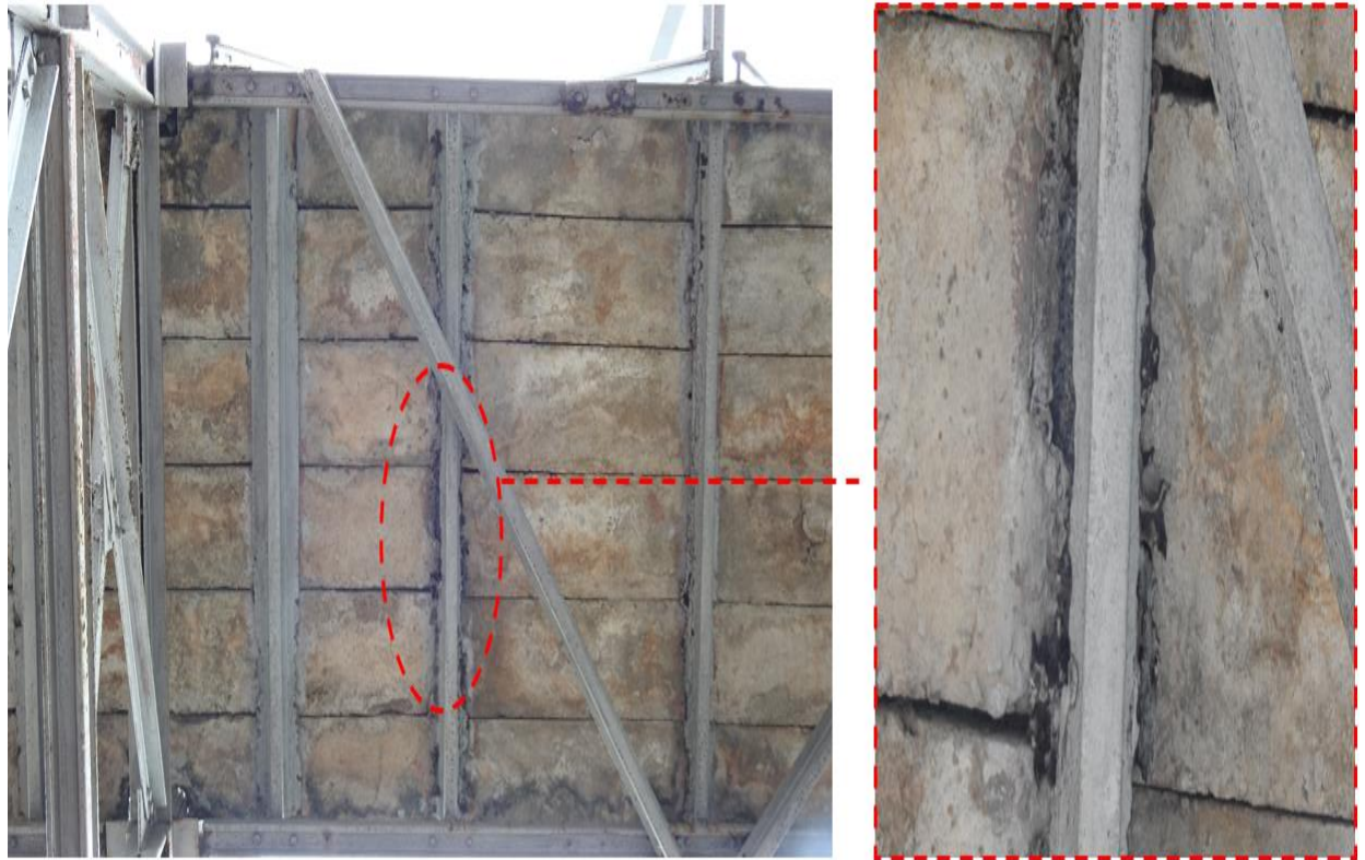
a) Corrosion of Floor Beams at Span-2
