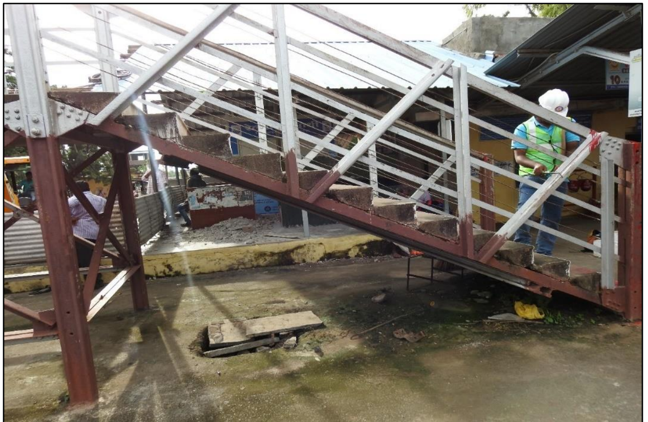
Fig 1.2: Red oxide coating observed at FOB
