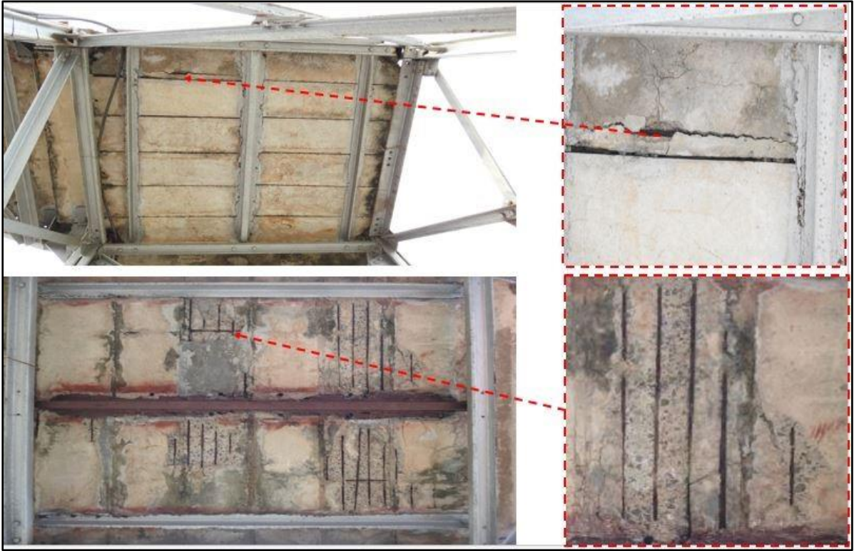
Exposed reinforcement is observed on staircase Landing slab at plat form 1 and 2
