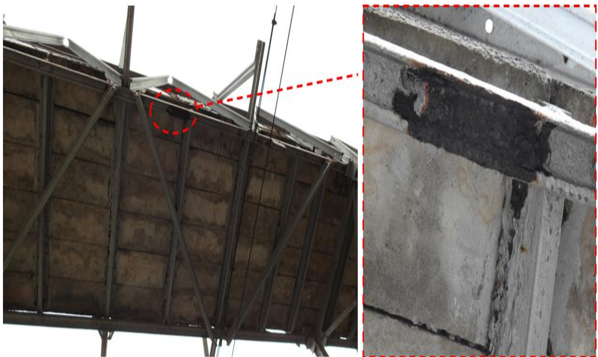
d)Corrosion of Bottom chord in Span 2
