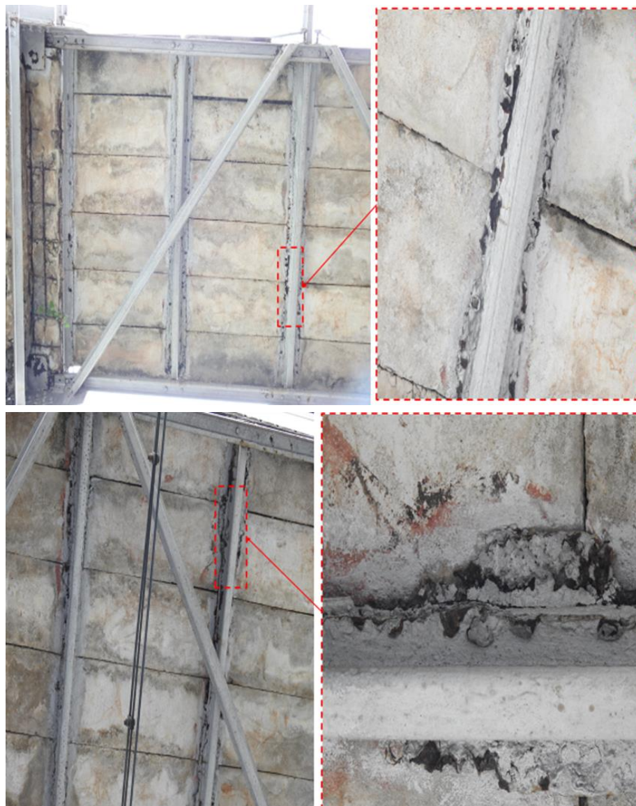
Fig: 2.3 Corrosion observed in floor beams
