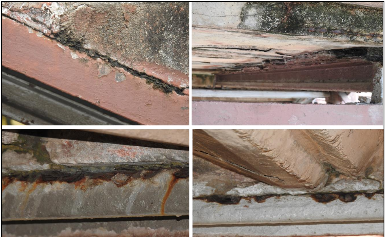
Fig 1.4: Corrosion is observed at Stringer beam joint
