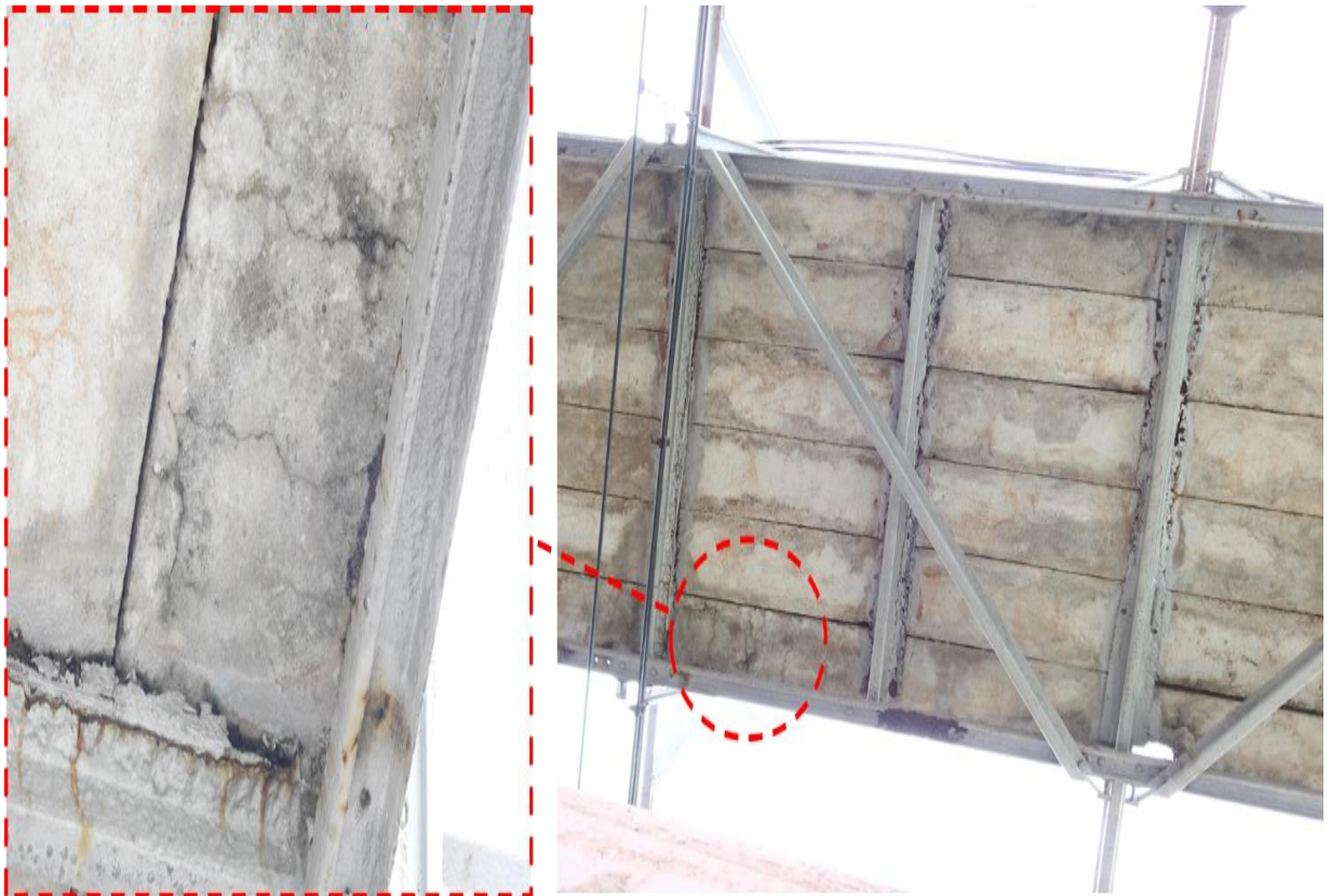
a) Cracks observed at Span-1 & Span 2
