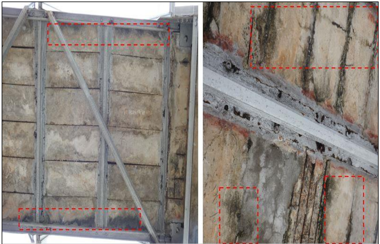
c) Leaching and water seepage is observed at slab panels
