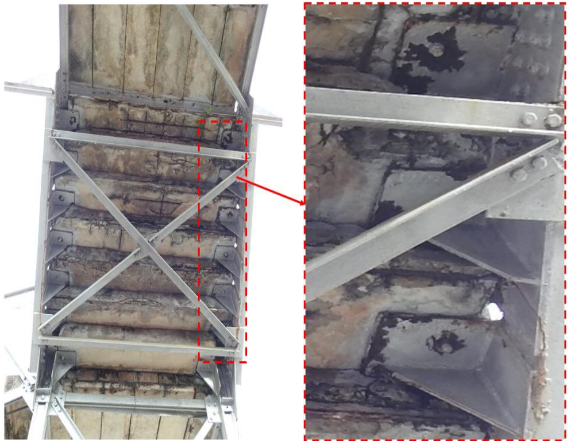
c. Corrosion at Cleat Angles of Stair Case
