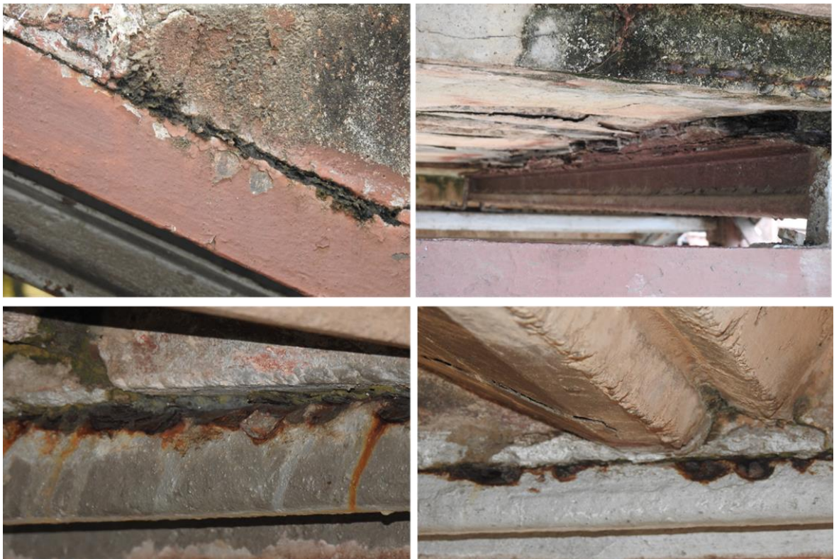
Fig: 2.5 corrosion in staircase stinger beam near steel concrete joint
