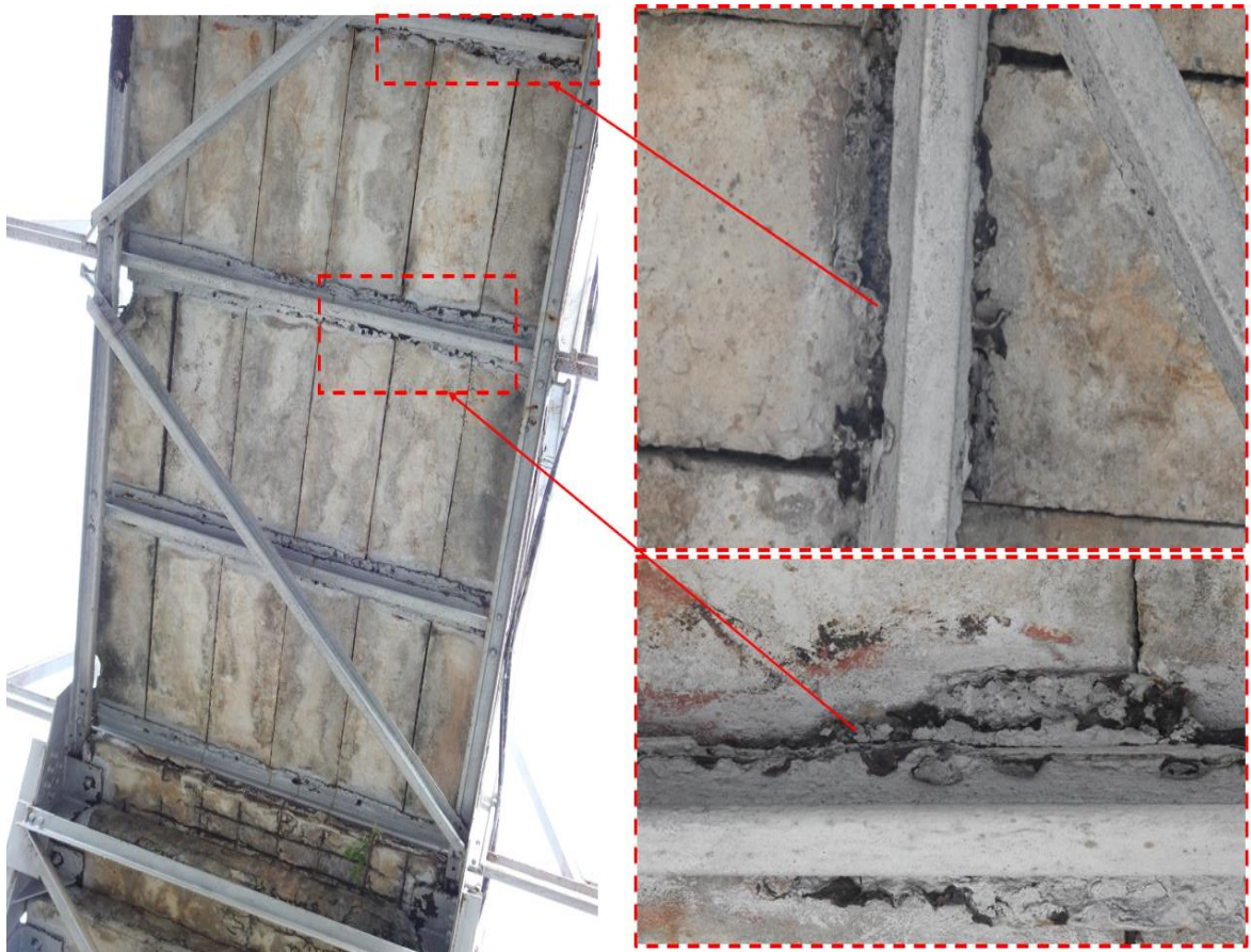
b) Corrosion of Floor Beams at Span-2
