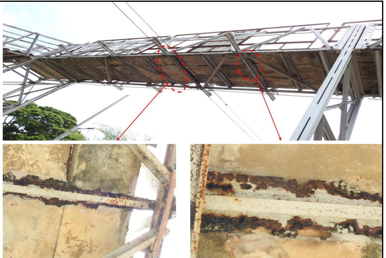
b) Corrosion of Floor beams is observed in 2 st span
