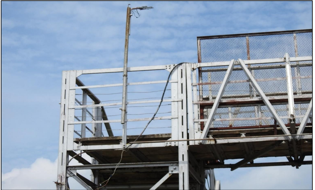
Fig 1.1: Cables, Electric post and protective screen
