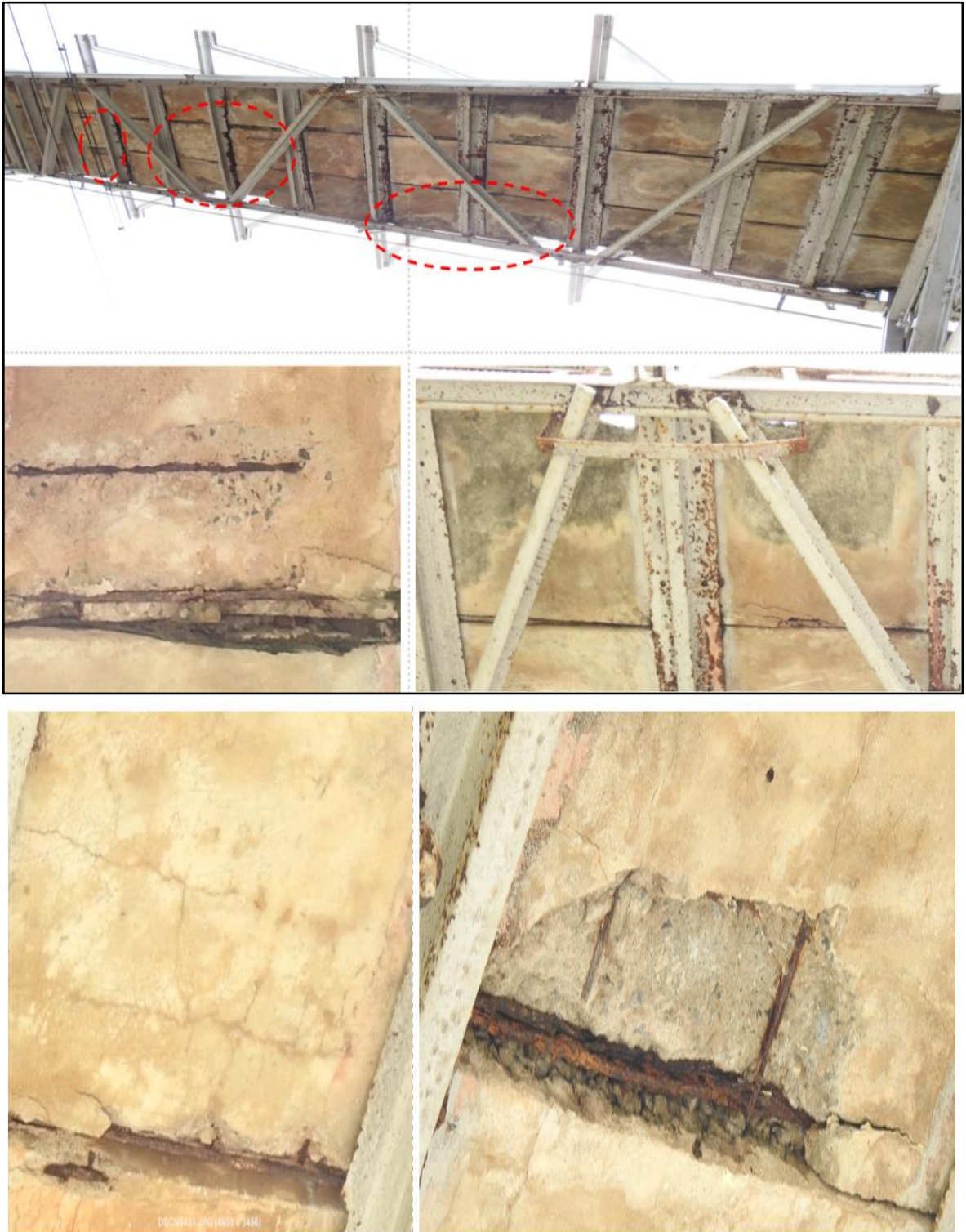
a) Reinforcement exposed at slab panels of 1 st span
