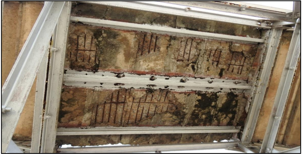
e) Spalling, Exposed Reinforcement and leaching observed in staircase 2 (Mid landing)
