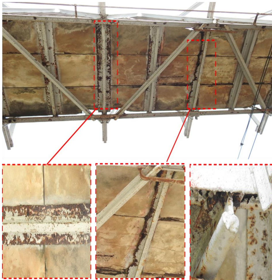
Fig: 2.6 Corrosion of floor beams in span-2
