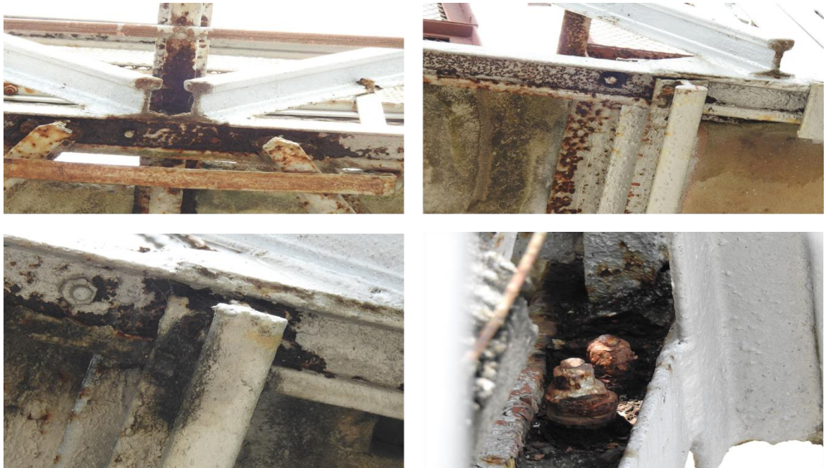
c) Corrosion of bottom chord
