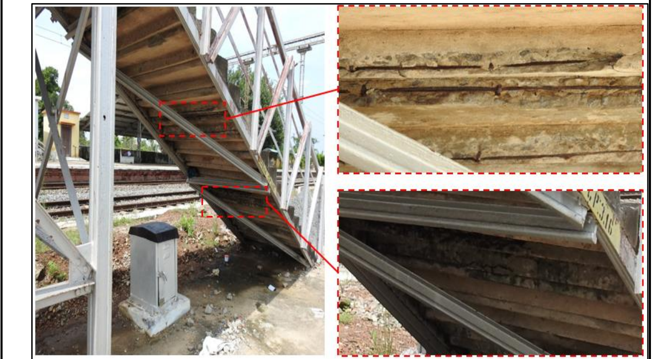
d) Reinforcement exposed slab panels on bottom of staircase-2
