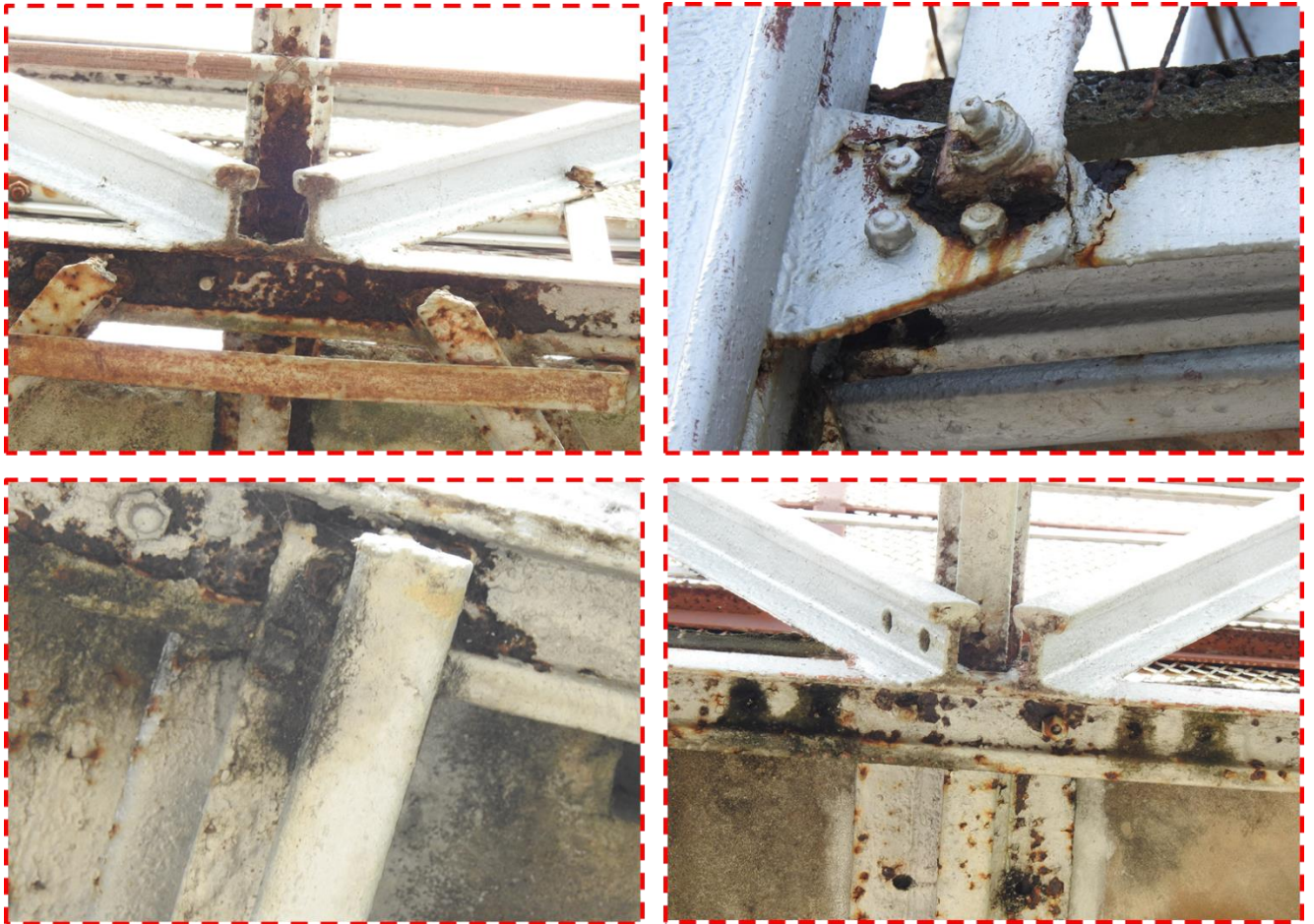
Fig: 2.3 Corrosion at joints and bottom chord
