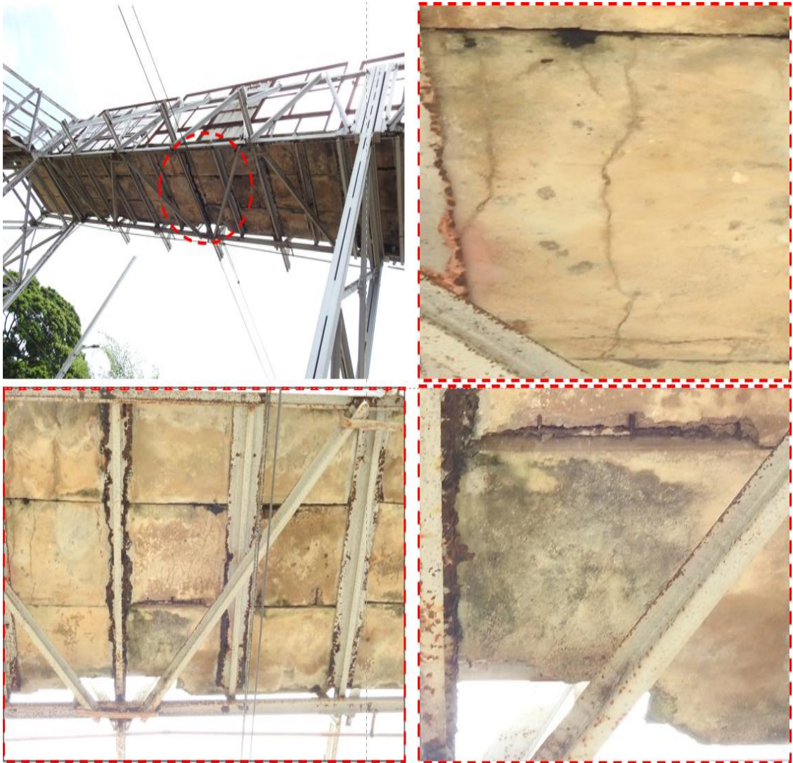
b) Reinforcement exposed at slab panels of 2 nd span
