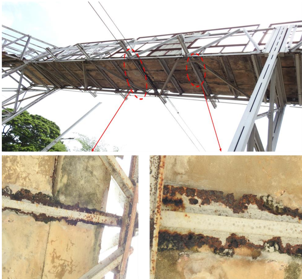
Fig: 2.5 Corrosion of floor beams in span-1
