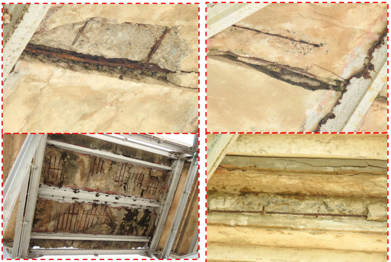
Fig: 2.4 exposed reinforcement in pathway pre cast panels and staircase mid landing
