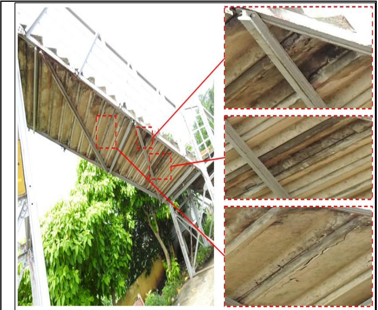
c) Reinforcement exposed slab panels on bottom of staircase-1
