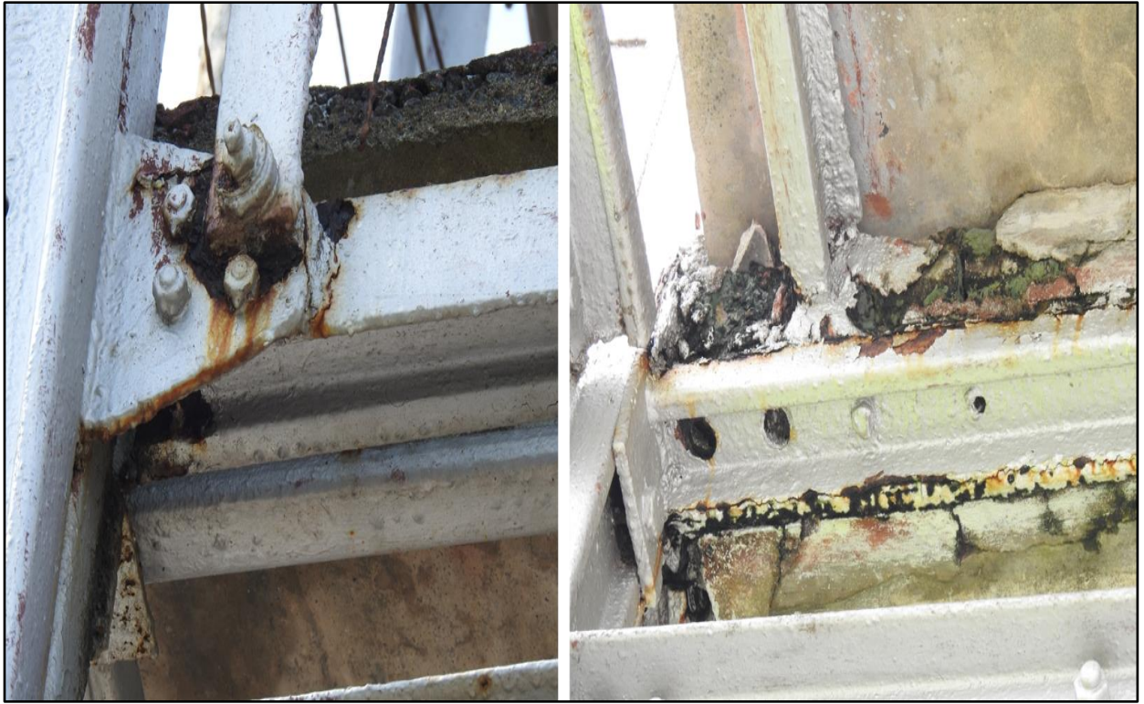
Fig 1.7: Corrosion is also observed at steel concrete joint gusset plate
