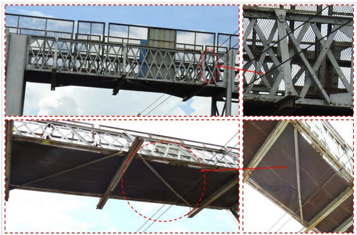
Fig.2.10 Deformation in Diagonal members, Slab bottom lateral bracing
