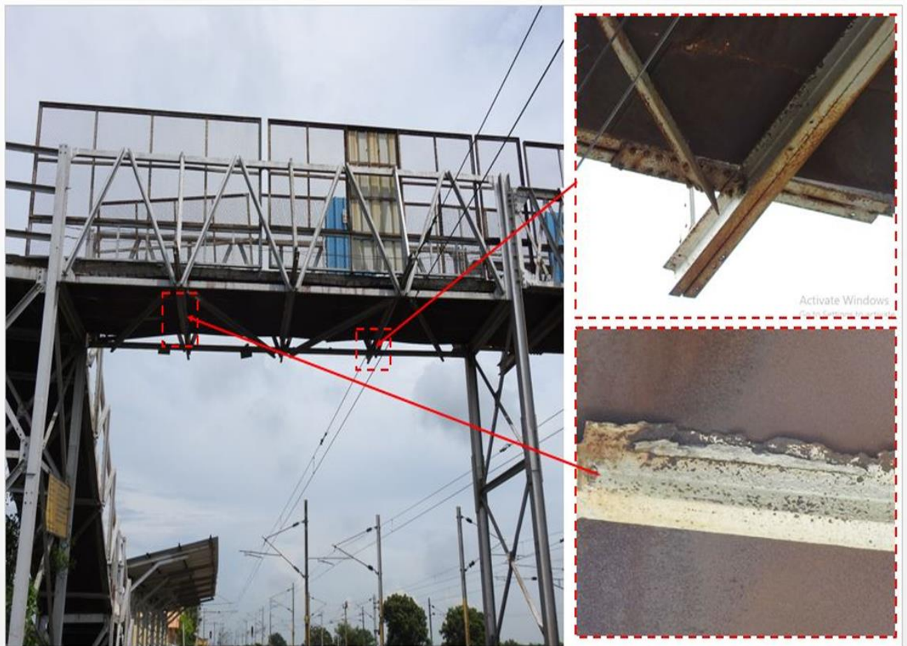
Fig.2.8 Corrosion of floor beams at span-4
