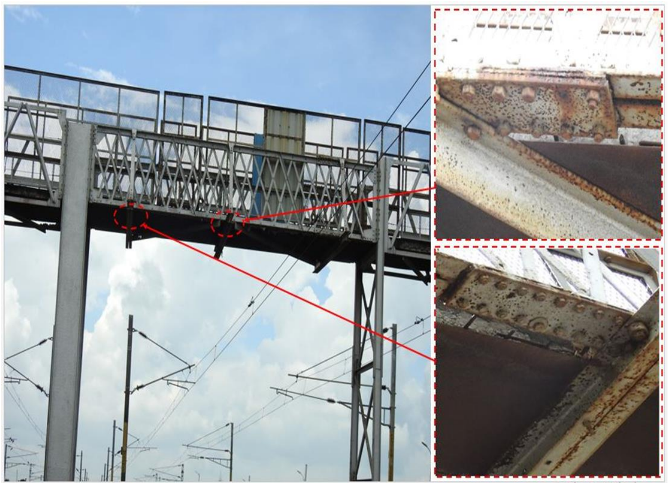
Fig.2.4 Corrosion of floor beams and slice joint at span-2
