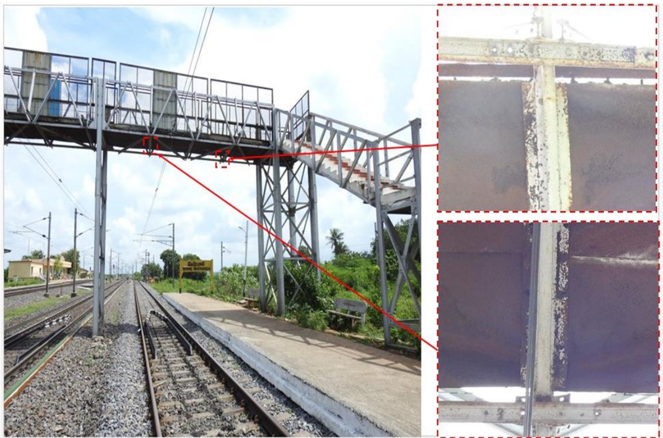
Fig.2.2 Corrosion of floor beams at span-1
