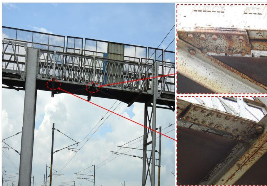
b) corrosion in splice joint at Span-2
