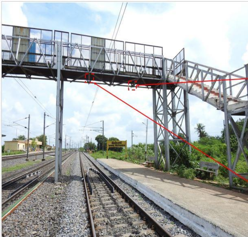
a) Corrosion of floor beams at Span-1
