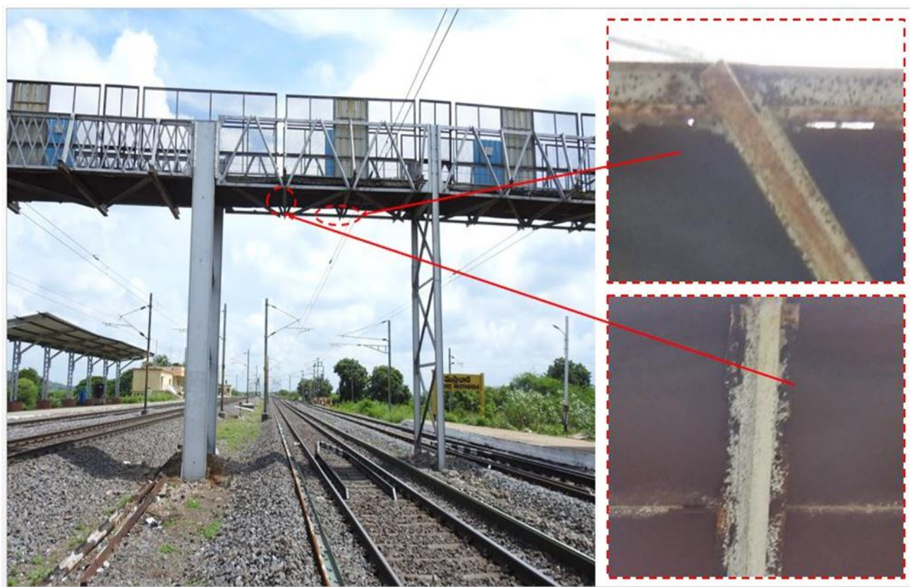
Fig.2.6 Corrosion of floor beams at span-3
