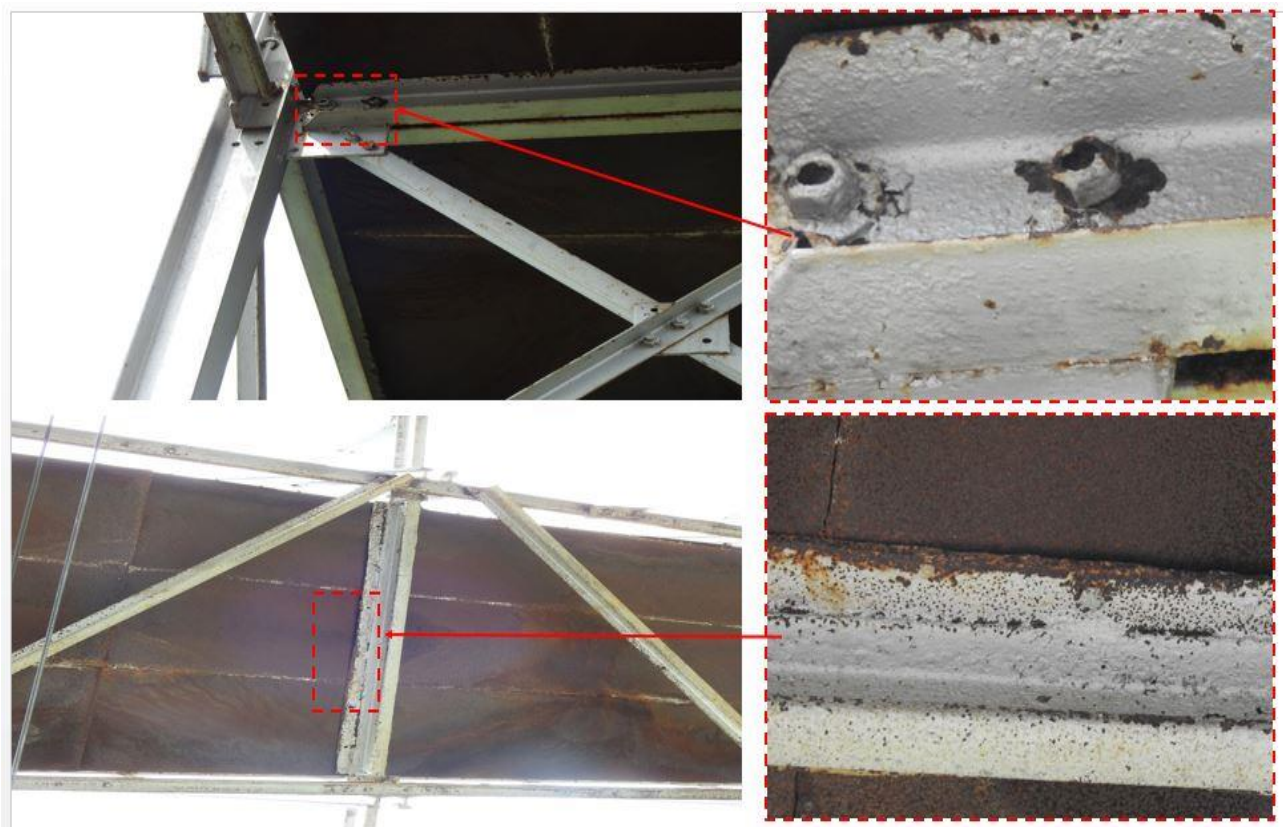
f) Corrosion at Floor Beam
