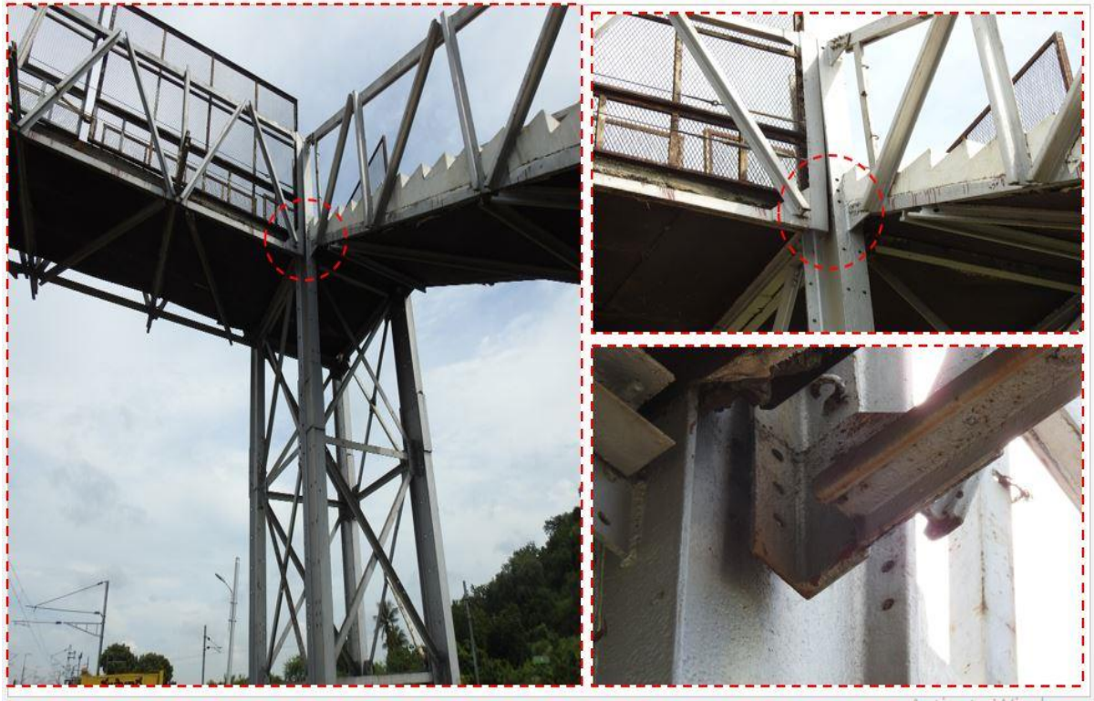
Fig.2.9 Connection failure at Stair Case-2
