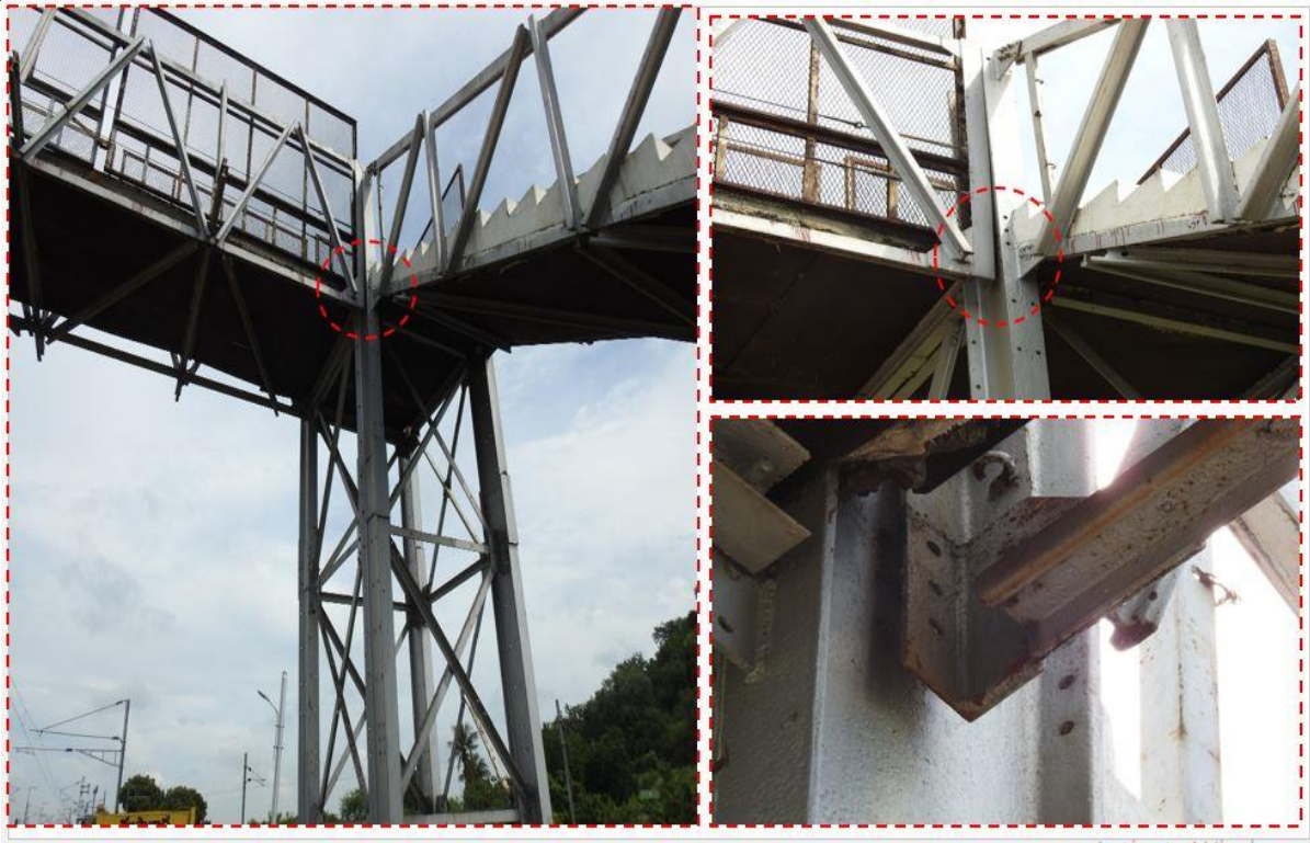
Connection failure at Stair Case-2
