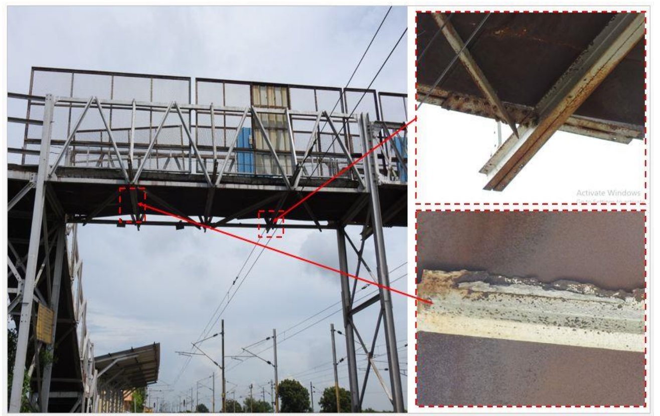
d) Corrosion in floor beams at Span-4
