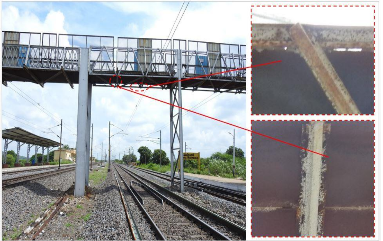
c) Corrosion in floor beams at Span-3
