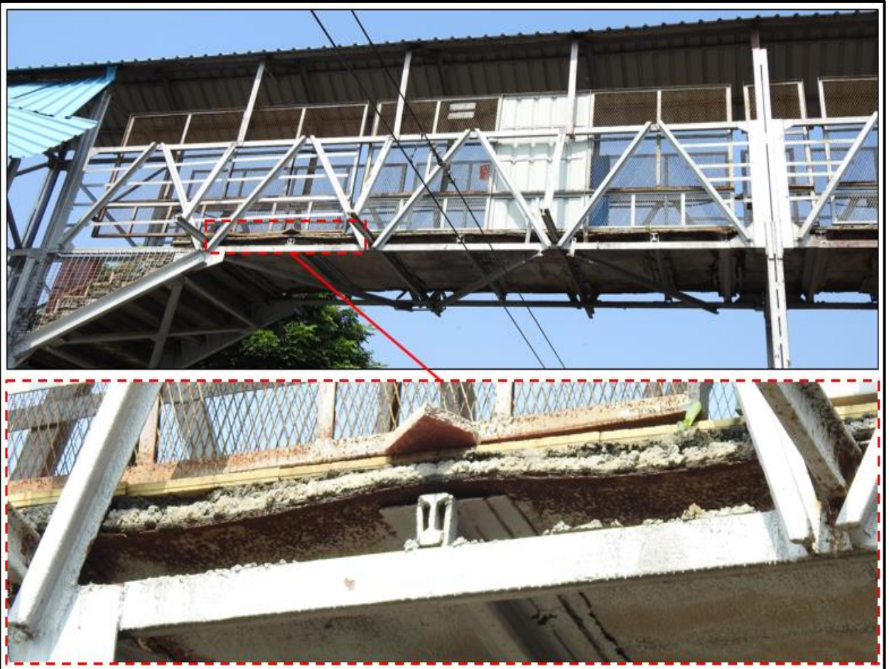
VI. Deformation at slab panels on Span-2
