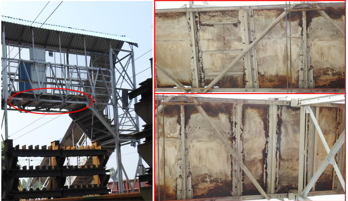
Fig 2.5: Corrosion of floor beams in span 2
