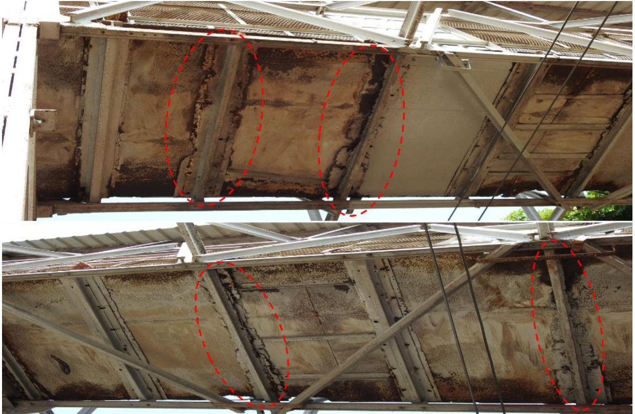
Fig: 1.8 Corrosion of floor beams in Span 1 and Span 2
