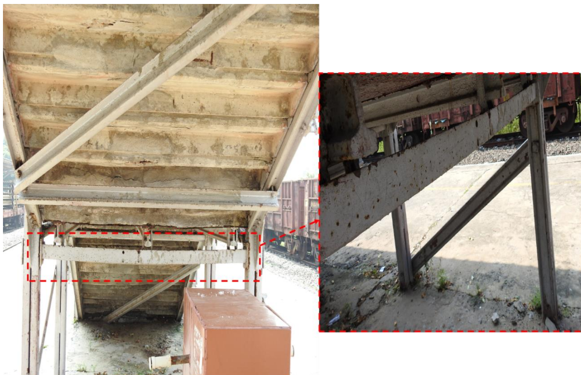
VII. Deformation of Tie beam at Staircase 2
