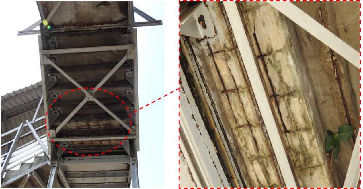
Fig 2.6: reinforcement exposure of pathway stair case
