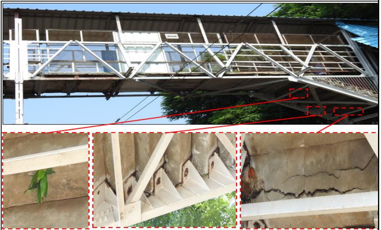
b) Vegetation, corrosion at cleat angles and cracks observed at pathway staircase Span 1
