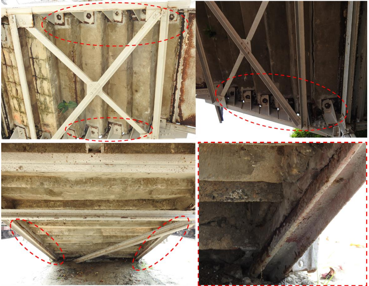
Fig: 1.9 Corrosion of Cleat angles and Stringer beam
