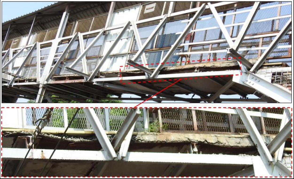
V. Deformation at slab panels on Span-1
