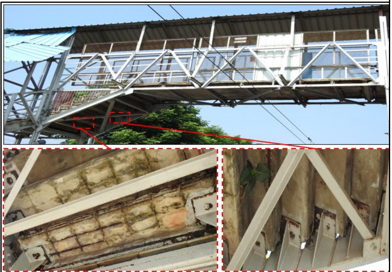
c) Vegetation , Reinforcement exposed and corrosion at cleat angles observed at pathway staircase Span 2
