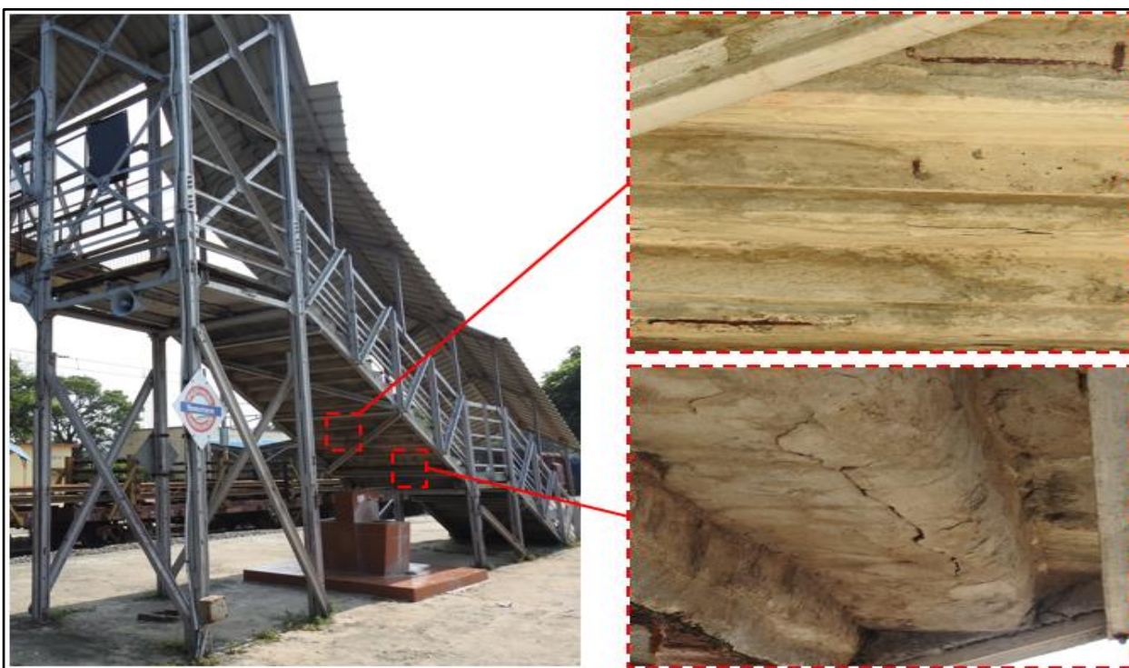
a) Cracks and reinforcement observed at Staircase 2 bottom
