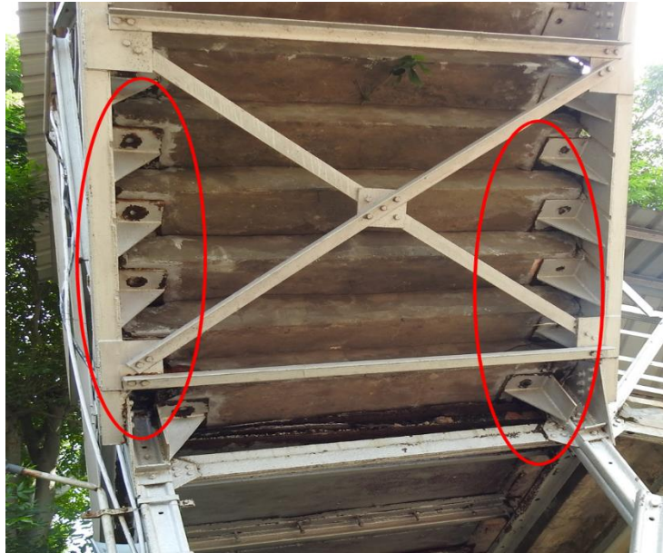
Fig 2.3: Corrosion of Cleat angles along the staircase
