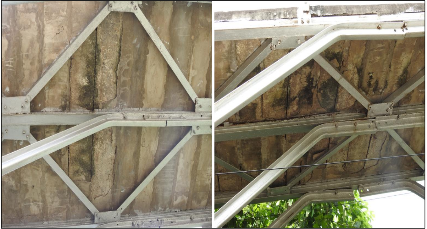
b) Spalling observed in ramp on both sides
