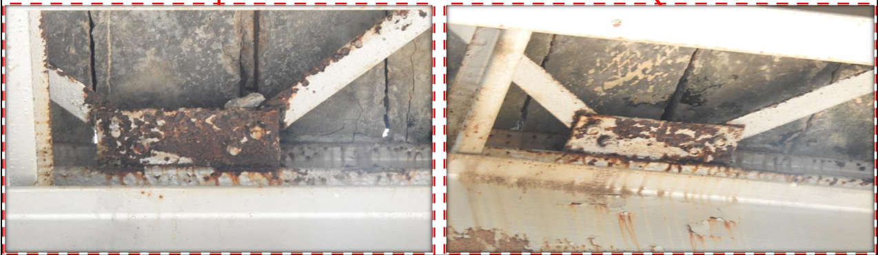
a) Corrosion of Gusset plate in 2 nd Span of FOB
