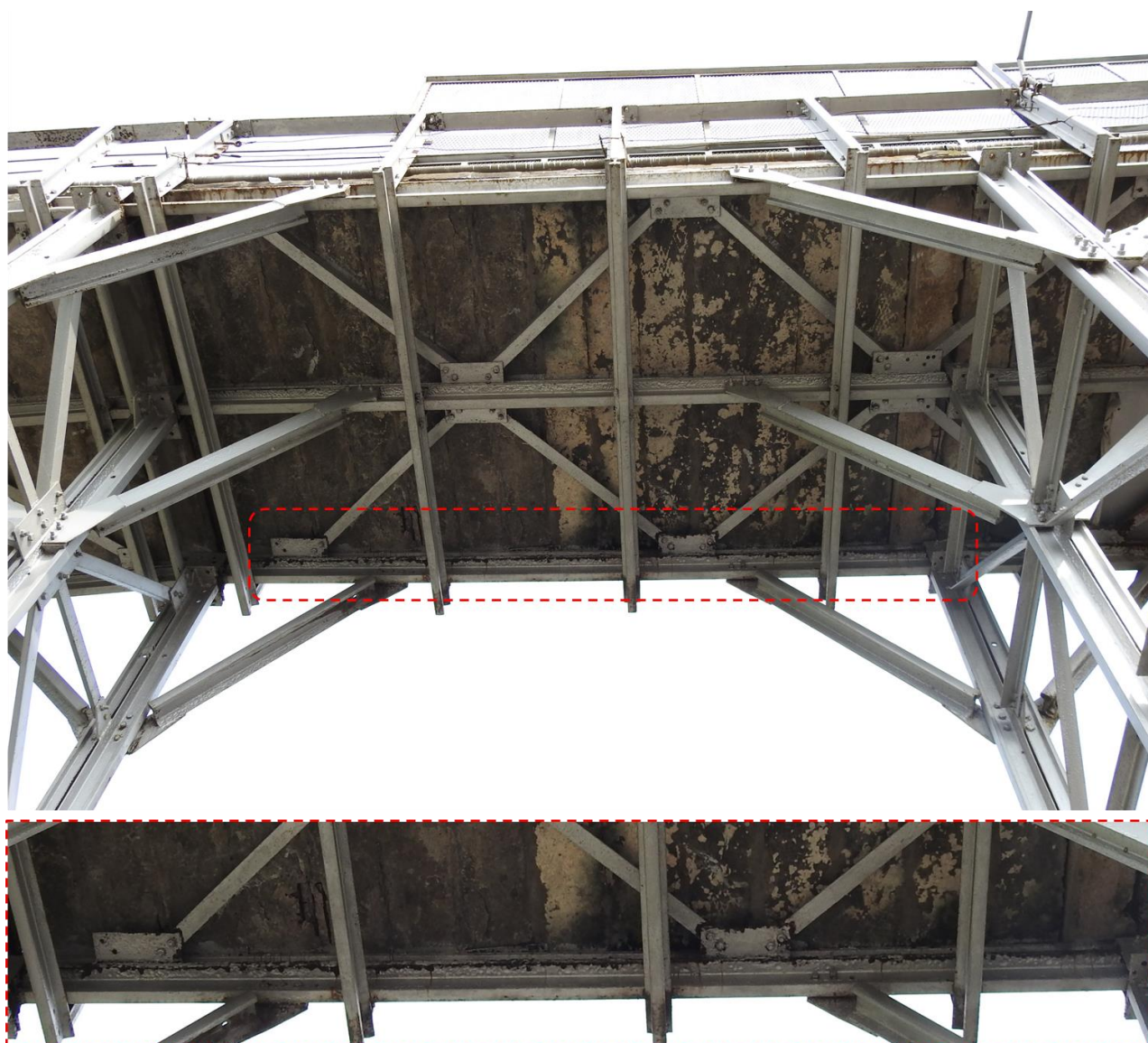
Fig 2.18: Corrosion of bottom chord members
