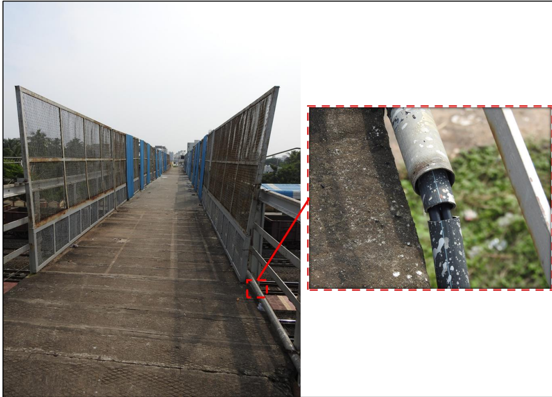
Fig 1.2: FOB pathway, protective screen, and cables on floor of pathway
