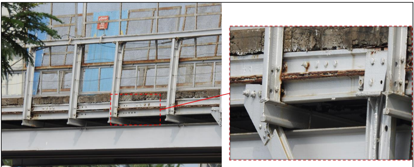
e) Corrosion observed in bottom chord
