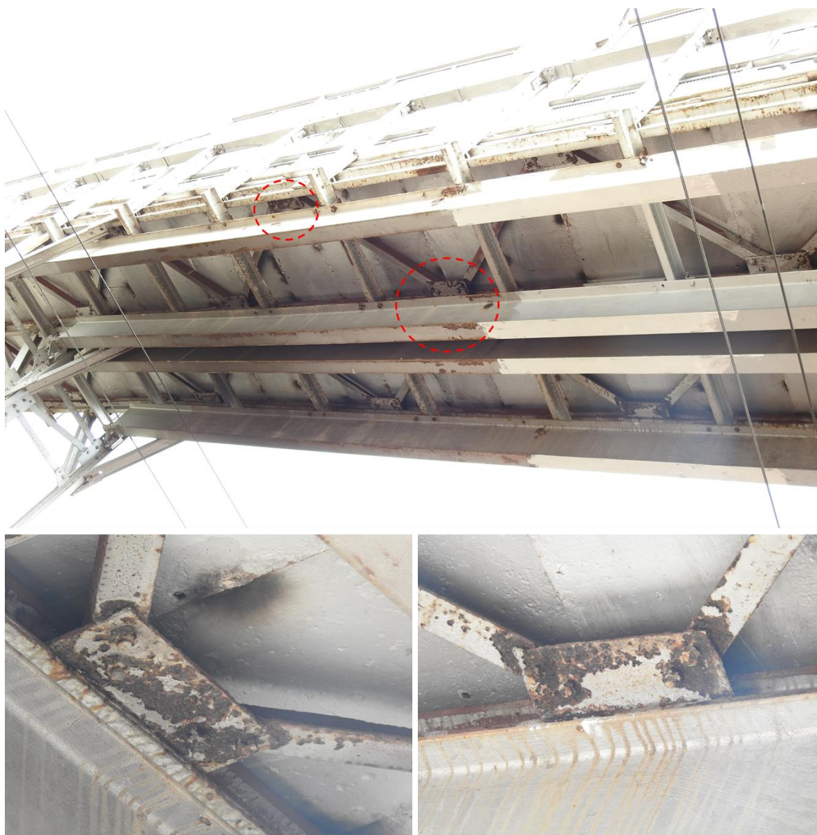
Fig 2.14: Corrosion of gusset plate and bottom chord members
