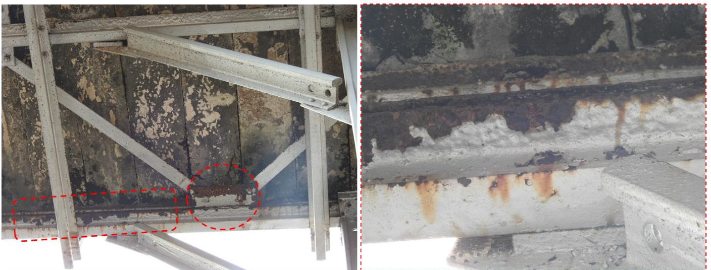
Fig 2.10: Sever corrosion of gusset plate and bottom chord member at steel concrete joint
