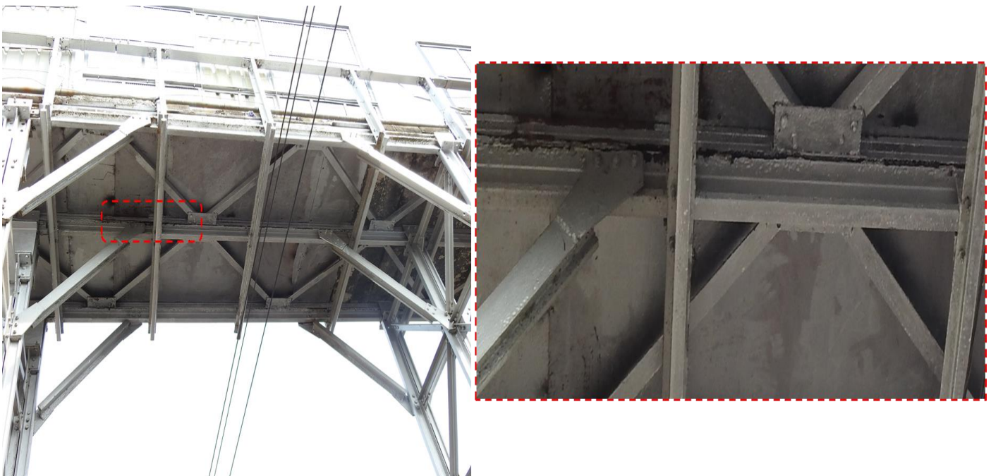
Fig 2.12: Moderate corrosion of floor beam in span 4
