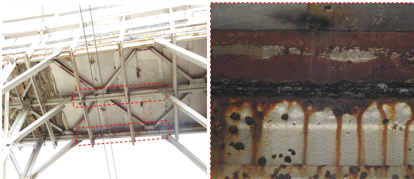
Fig 2.16: Corrosion of bottom chord members
