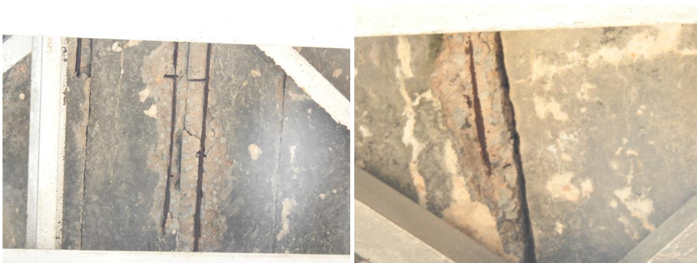
Fig 2.8: Exposed reinforcement in precast slab panels in span 2
