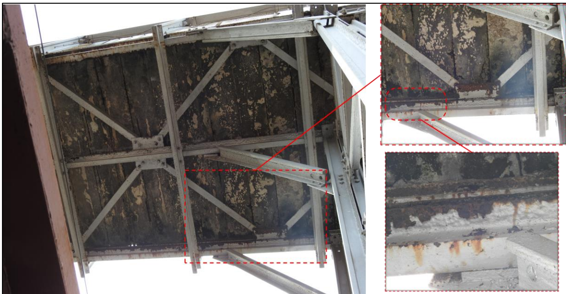
b) Corrosion of Gusset plate and bottom chord member in 3 rd span of FOB
