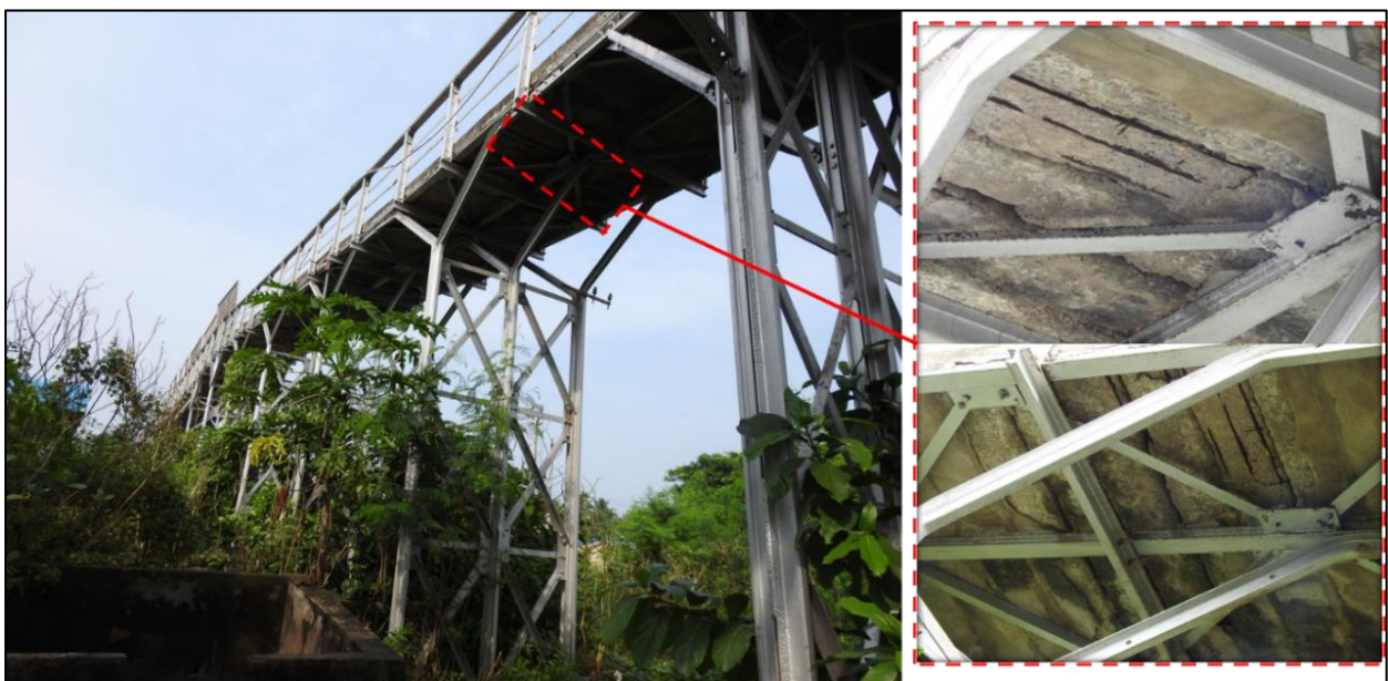
a) Reinforcement exposed slab panels
