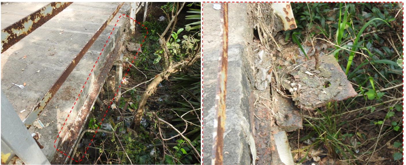
Fig 2.21: Severe corrosion in floor beam supporting flight of ramp
