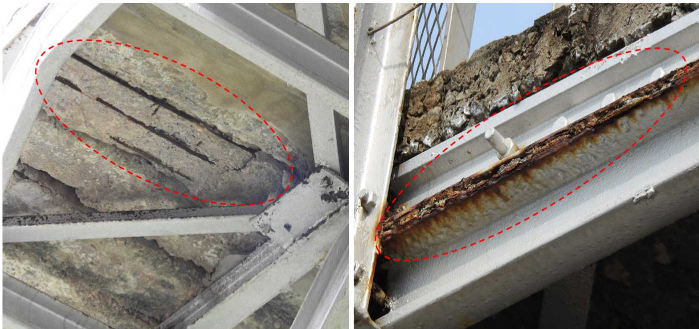
Fig 2.3: Exposed Reinforcement and moderate corrosion in bottom chord member
