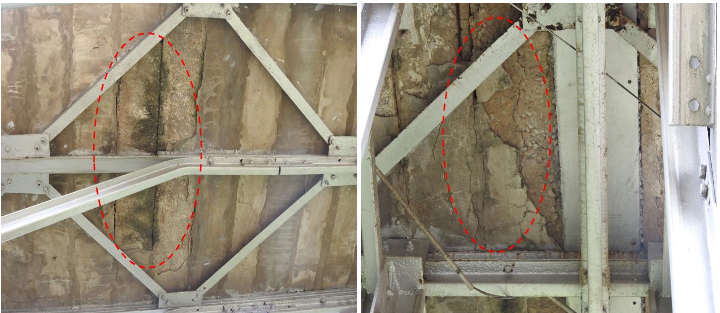
Fig 2.2: Algae and cracks in Ramp -1 pre-cast slab panels
