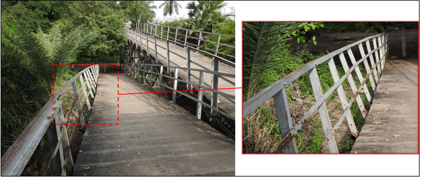
Fig 1.6: Damaged ramp railing
