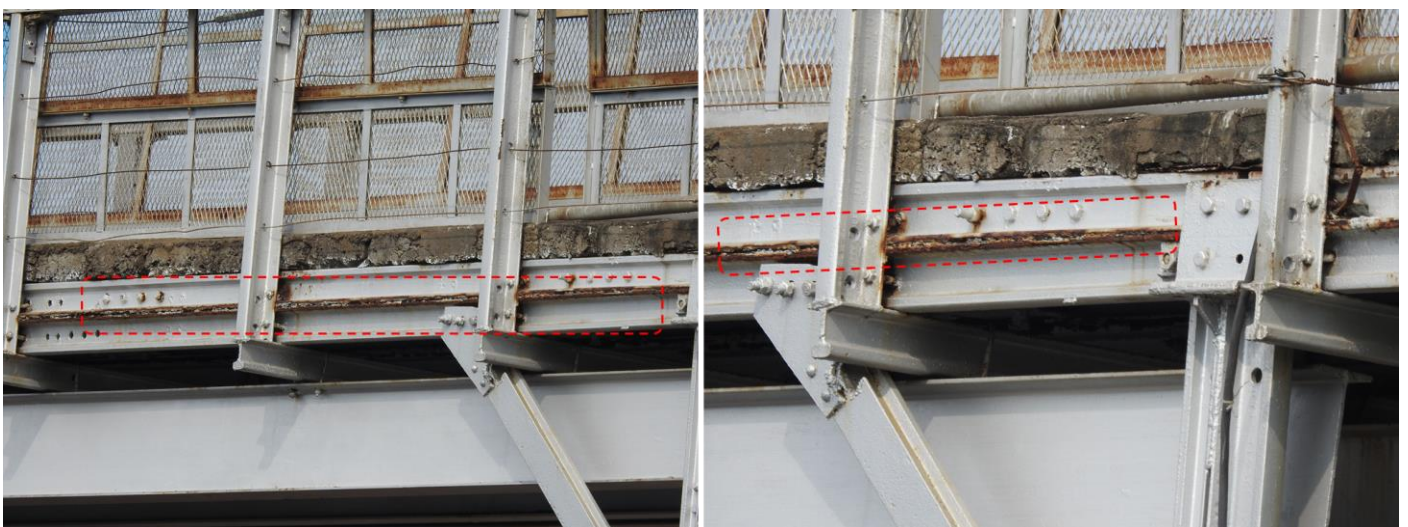
Fig 2.22: Moderate Corrosion in bottom chord member
