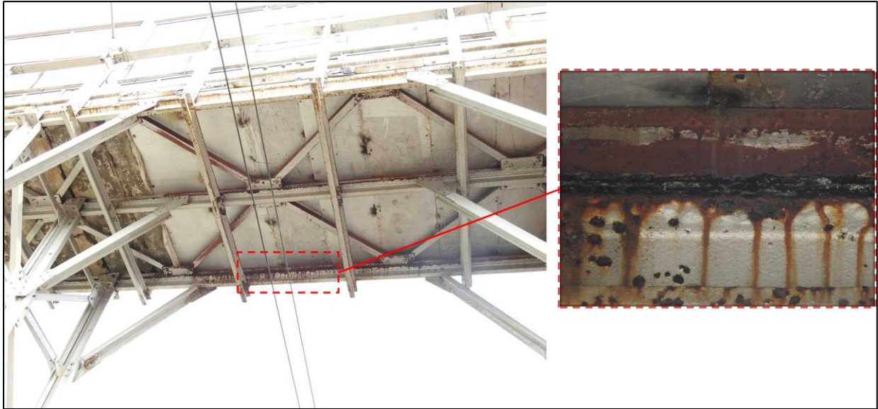
c) Corrosion of bottom chord member in 5 th span of FOB
