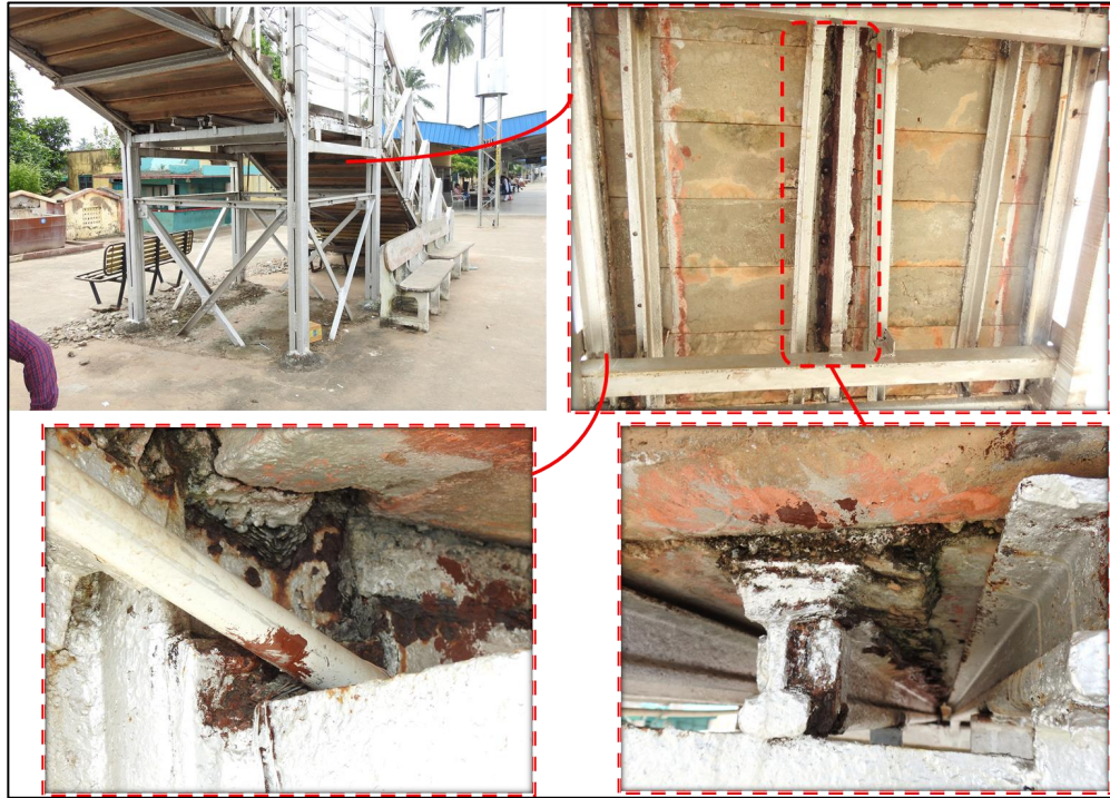
Fig 2.4: Corrosion of floor beam and stringer beam in staircase-1
