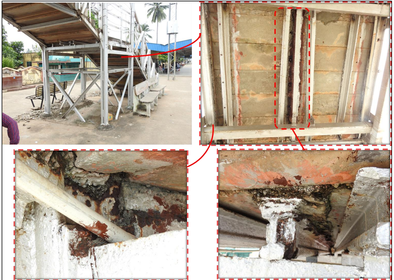
(a) Corrosion of floor beam and stringer beam in staircase-1
