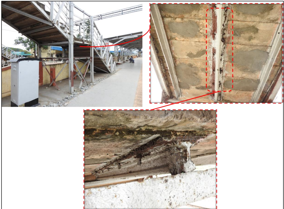
Fig 2.5: Corrosion of floor beam in staircase-2
