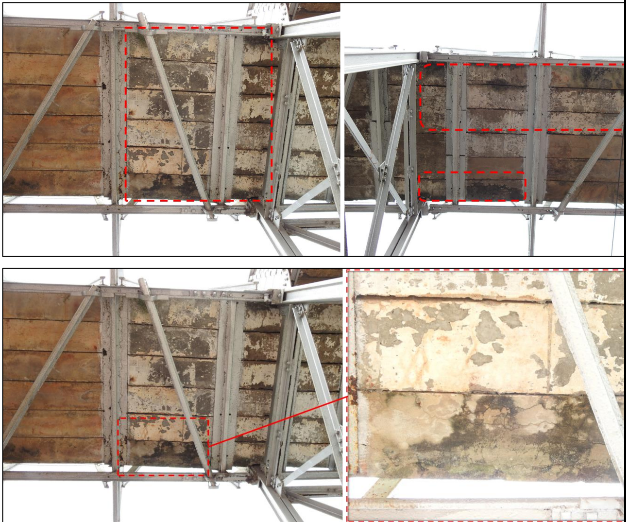
(a) Leaching and cracks in slab panels
