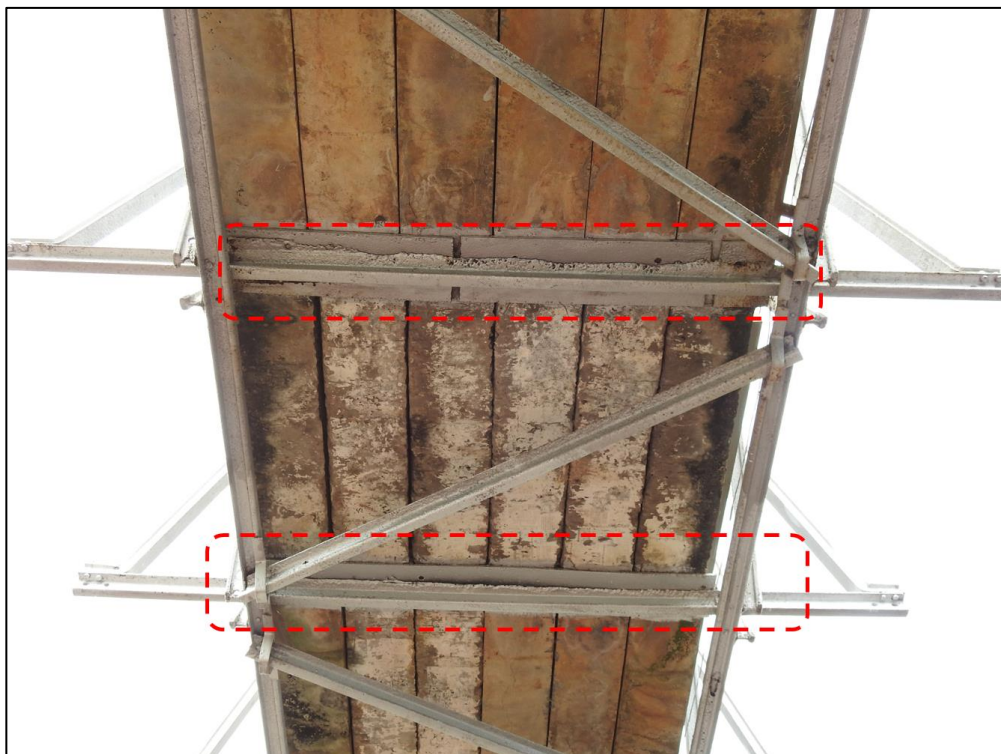
Corrosion of Floor beam coated with silver oxide paint
