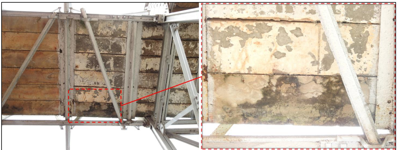
Fig 2.7: cracks in slab panels
