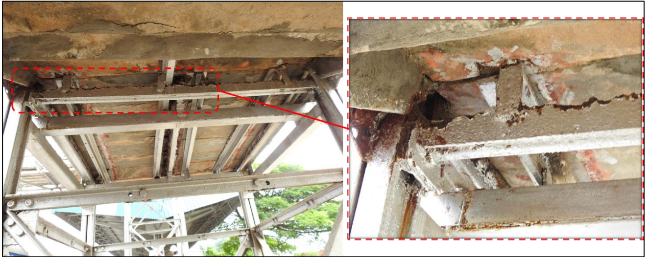
Fig 2.6: Corroded angle section in staircase -1
