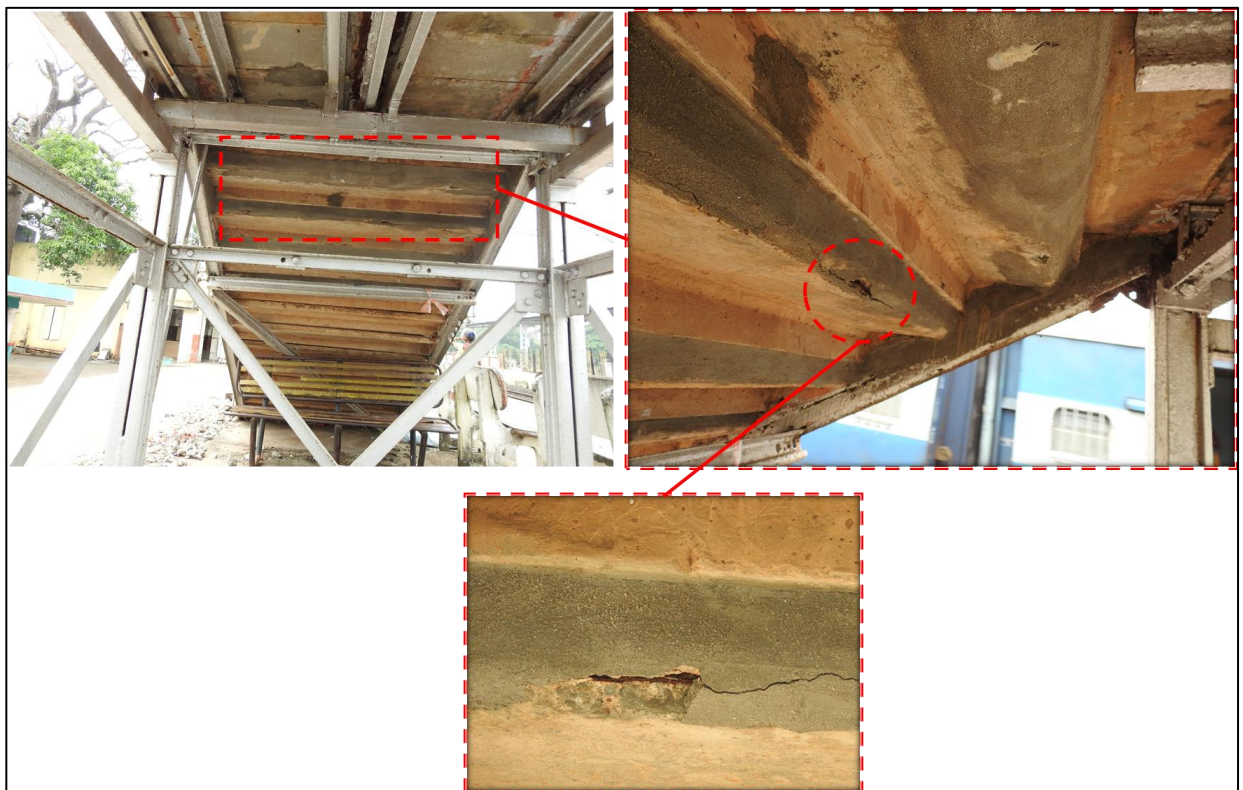
Fig 1.7: Patch work and reinforcement exposed in staircase -1
