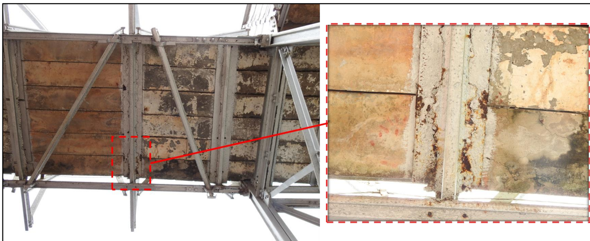
Fig 2.3: Corrosion of Floor beam
