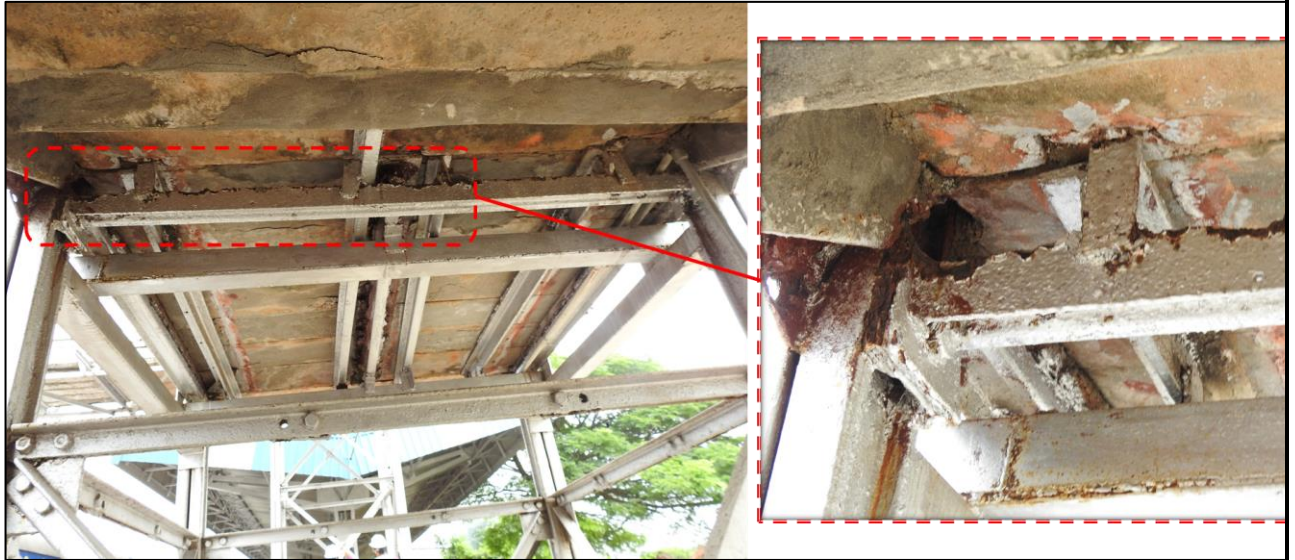
(c) Corroded angle section in staircase -1
