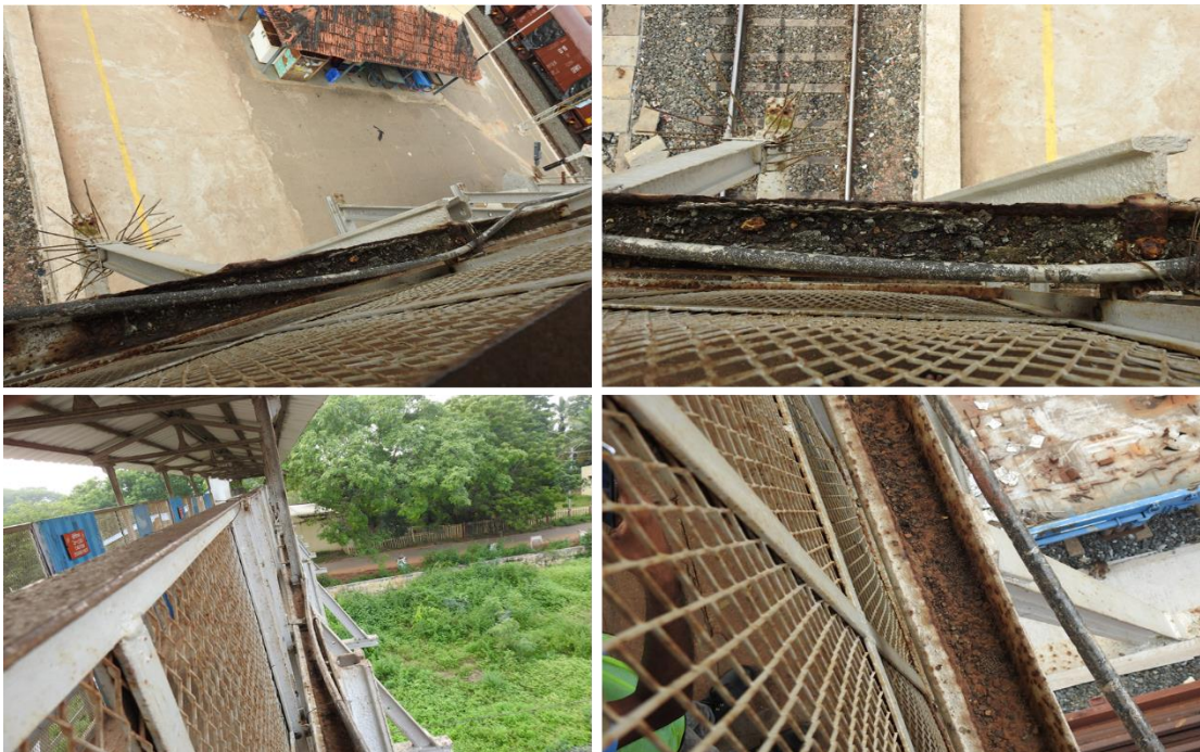
Fig 2.13: Locations of Corrosion observed at top chord members
