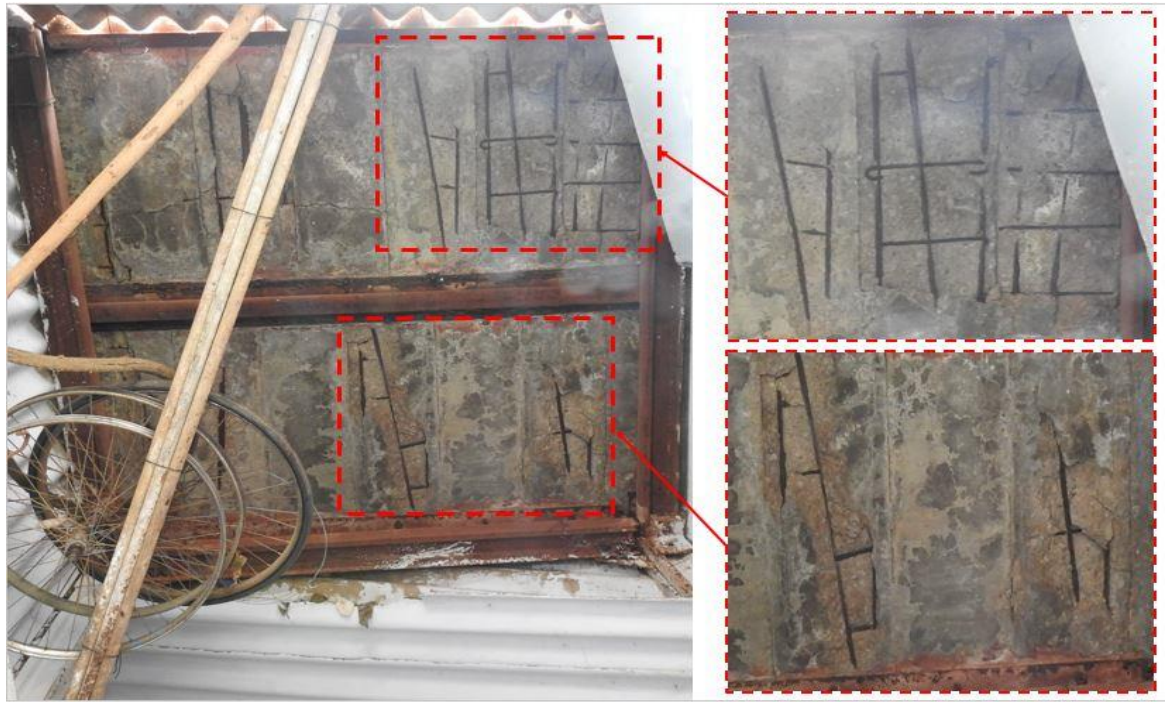
c) Spalling observed at Mid landing of Staircase-2
