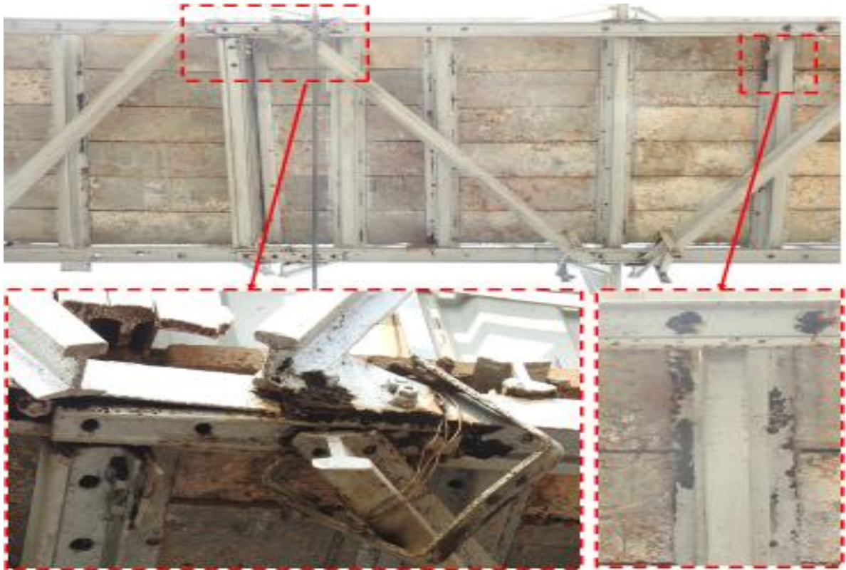
Fig: 1.14 Corroded joints and floor beam
