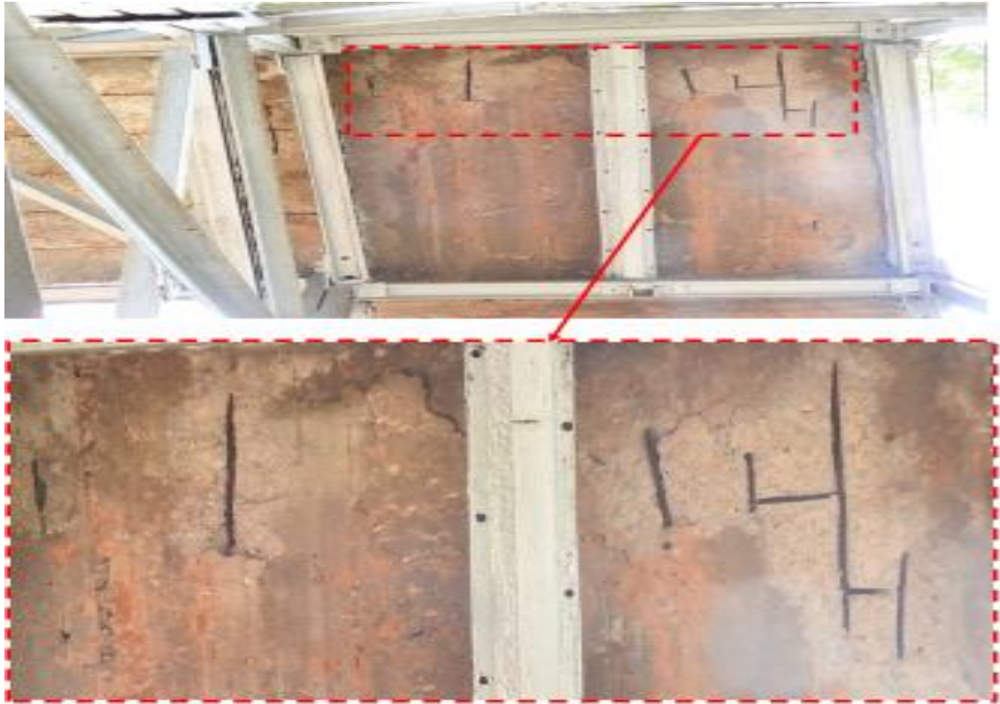
Fig: 1.16 Damaged panels observed at mid – landing of Staircase-1
