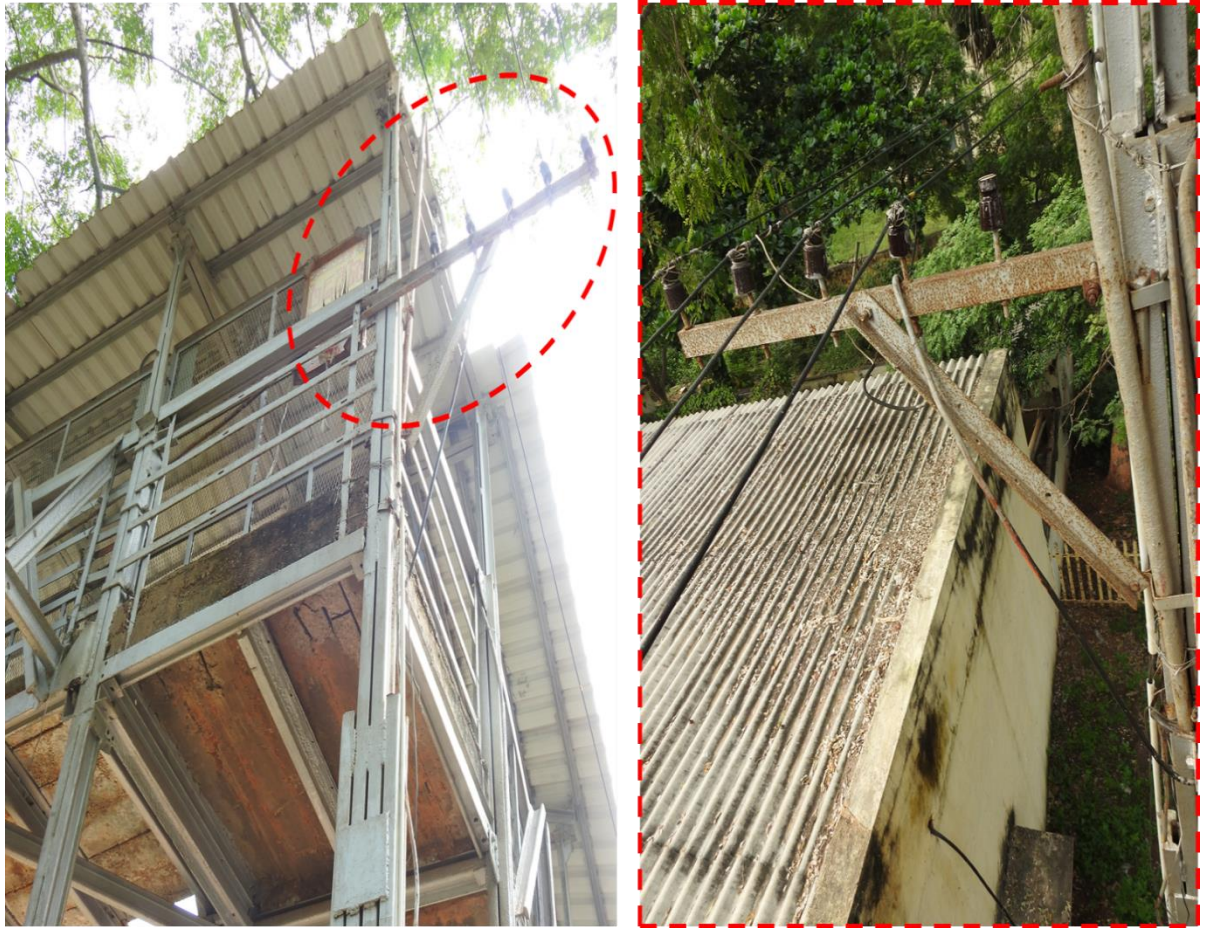
Fig 1.12: Electrical lines supported at Trestle 1
