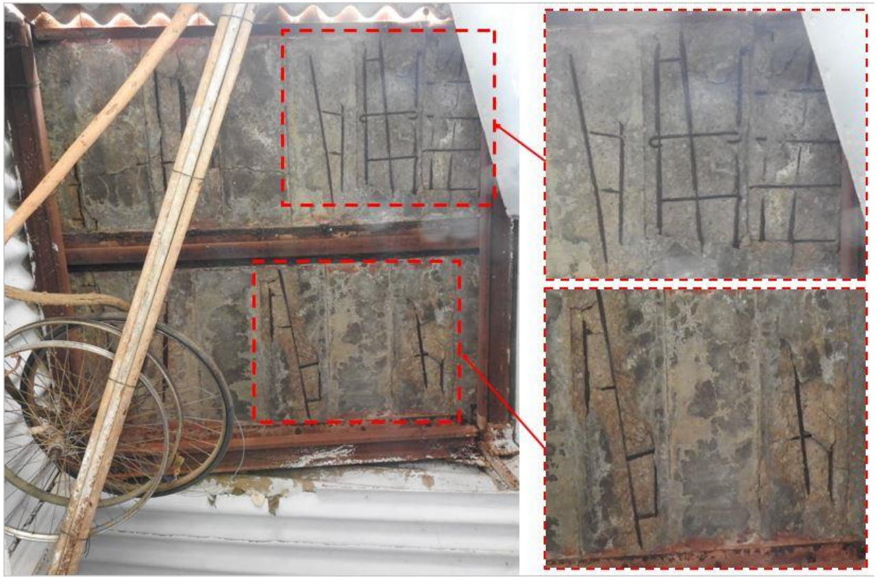
Fig 2.14: Locations of Deteriorations in Staircase 2
