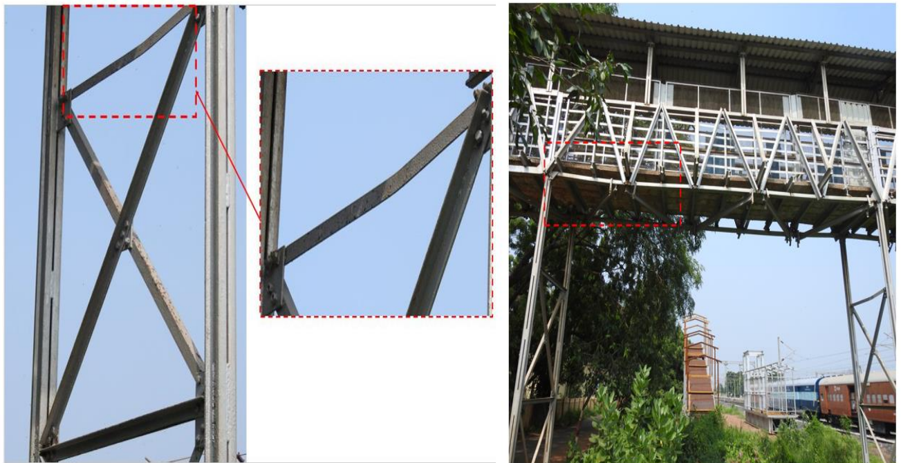
Fig 2.5: Deterioration locations of Horizontal bracing of stanchion 2 and Bottom chord of Span-2.
