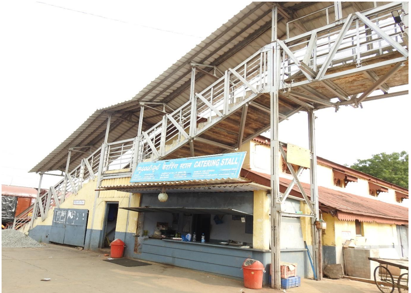
Fig 1.10: Unable to inspect under stair case-2 due to existing rooms (P.W Trolley shed)
