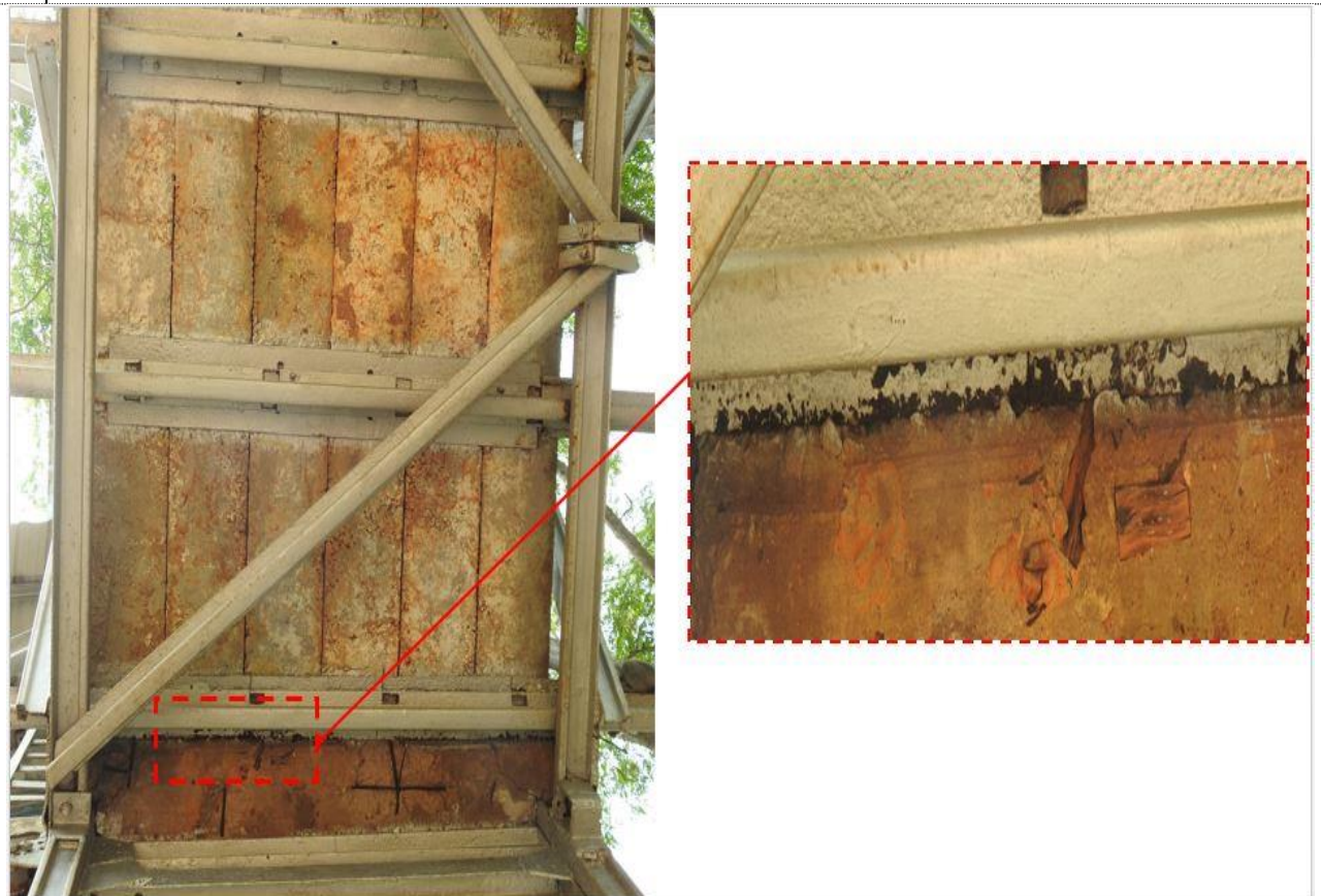
a) Corrosion observed at floor beams in Span-1
