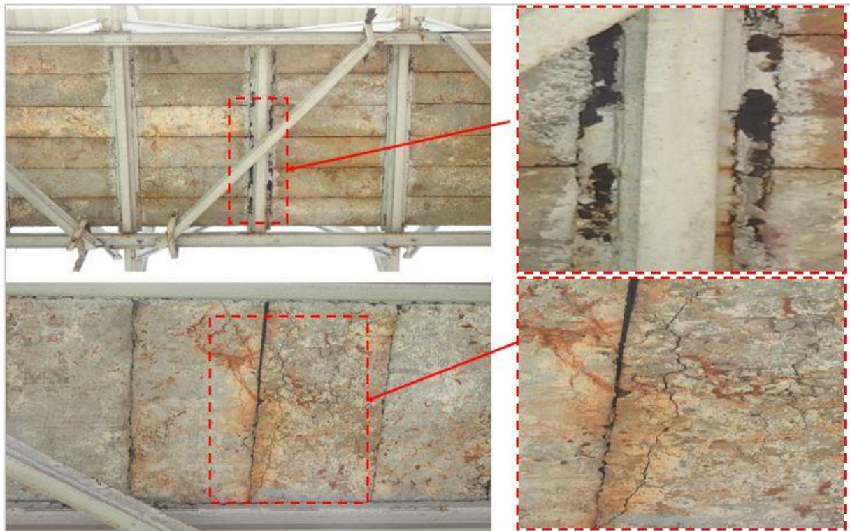
Fig 2.9: Floor beam corrosion and cracks in slab panels
