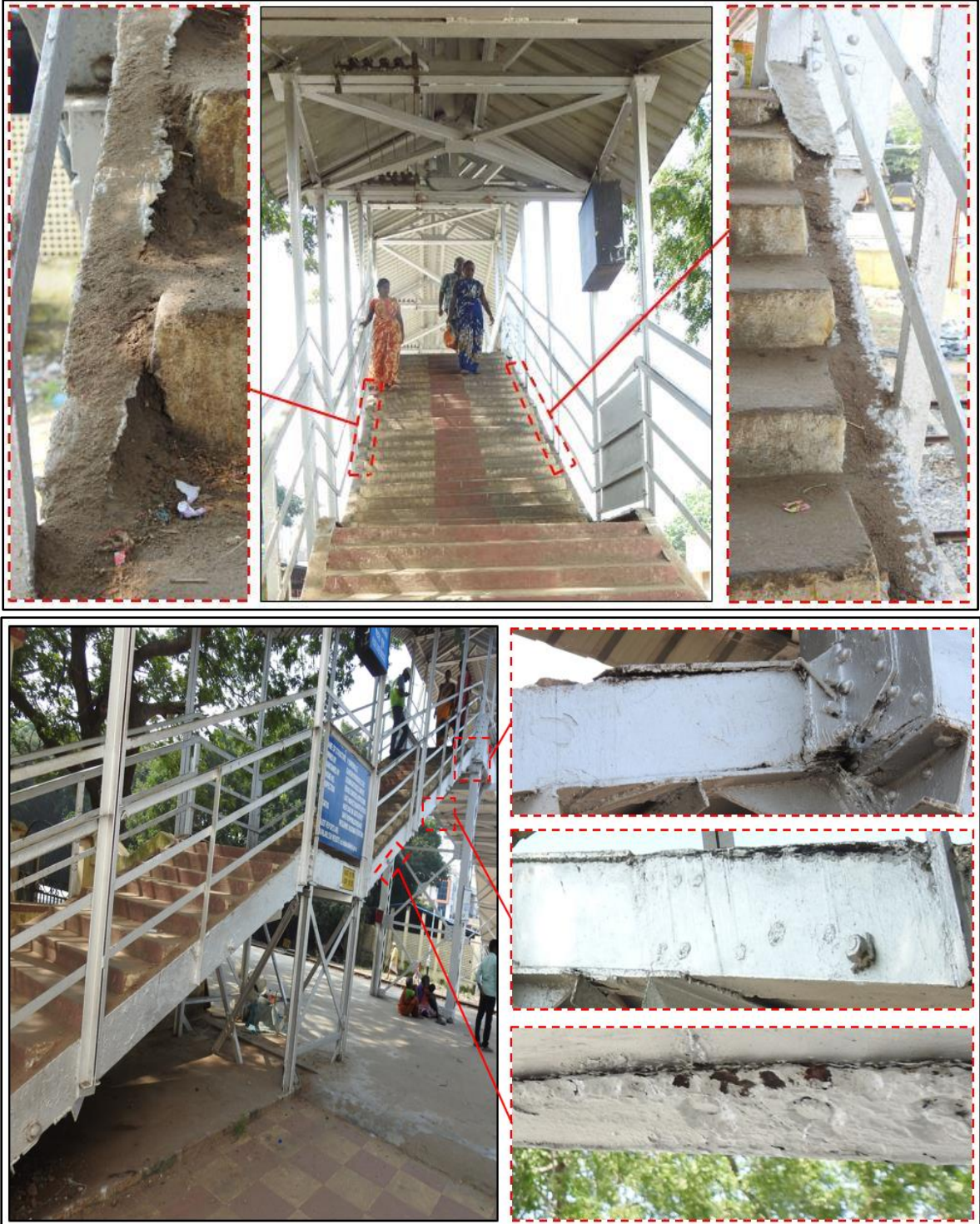
a) Corrosion observed at Staircase 1 Stringer beam
