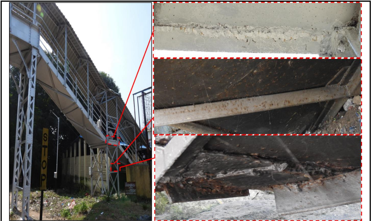
b) Corrosion observed at Staircase 2 Stringer beam and Corrosion of cross bracing
