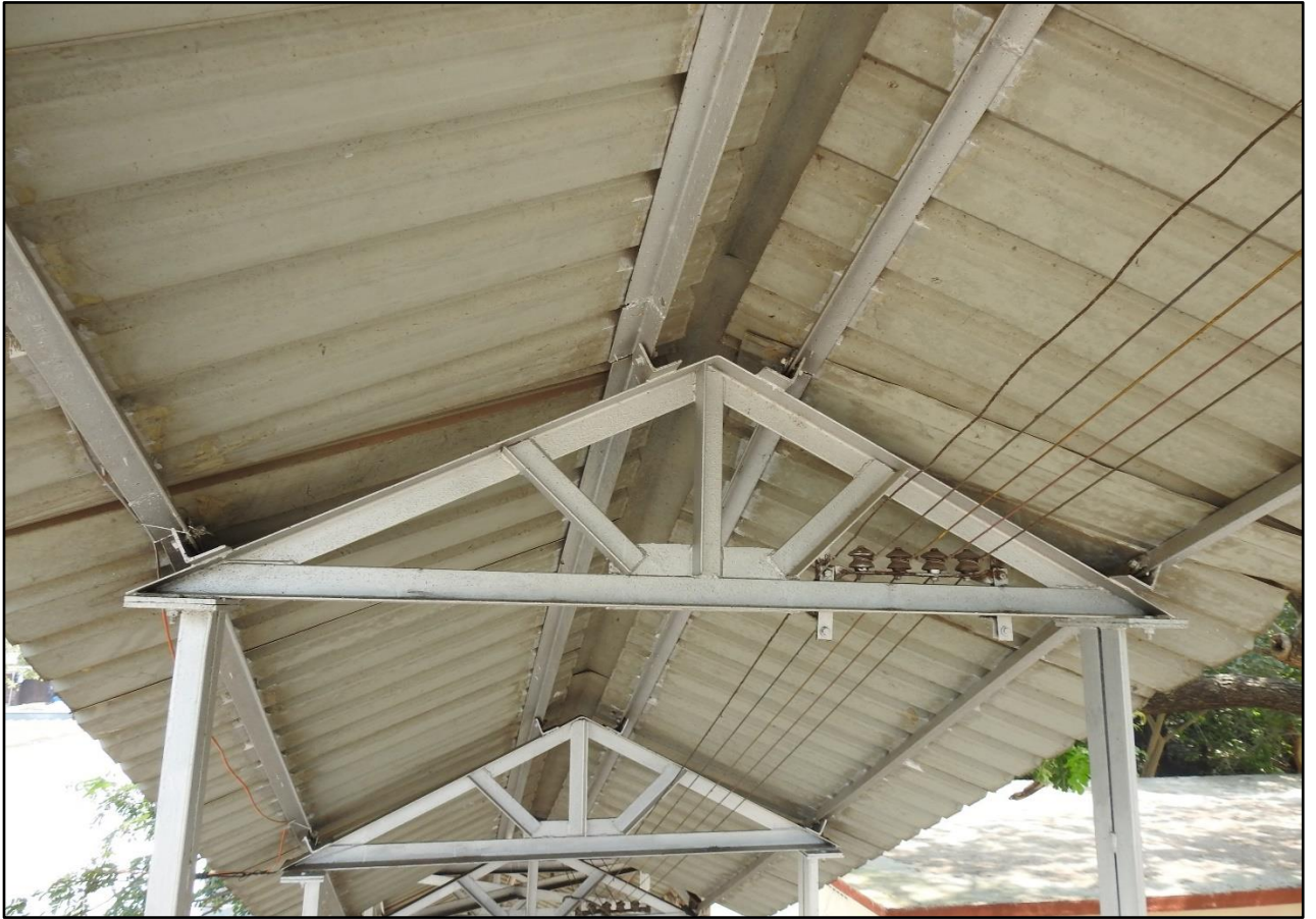
Fig 1.9: Insulated Electrical lines on Roof truss
