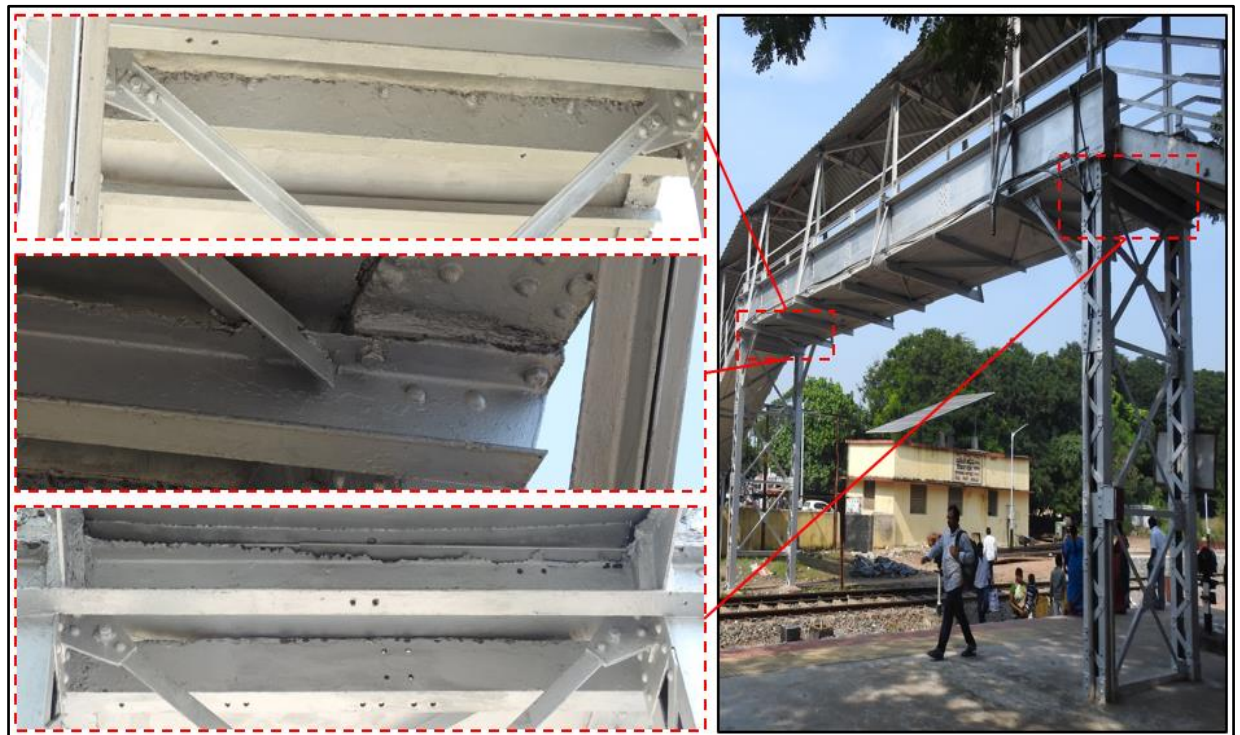
a) Corrosion observed at floor beams of FOB
