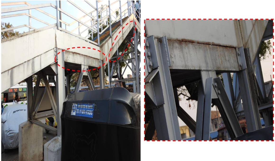
Fig: 3.17 Corrosion of Stinger beam at staircase-2
