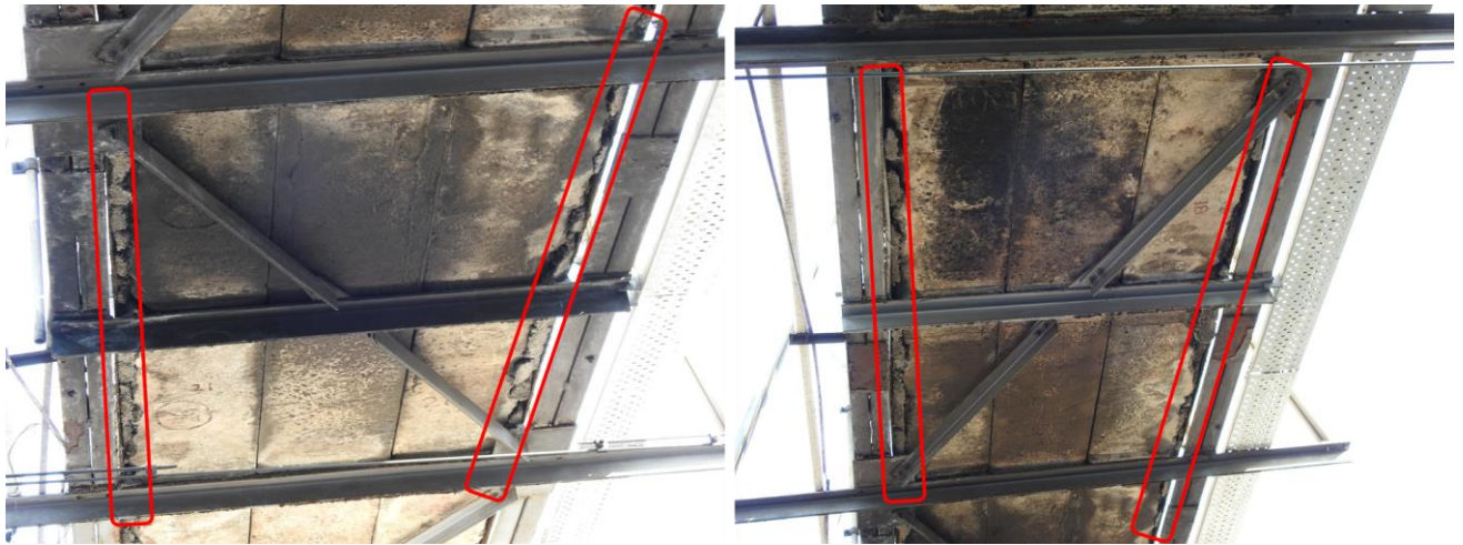
Fig 3.6: Exposed reinforcement in slab panels at span-2
