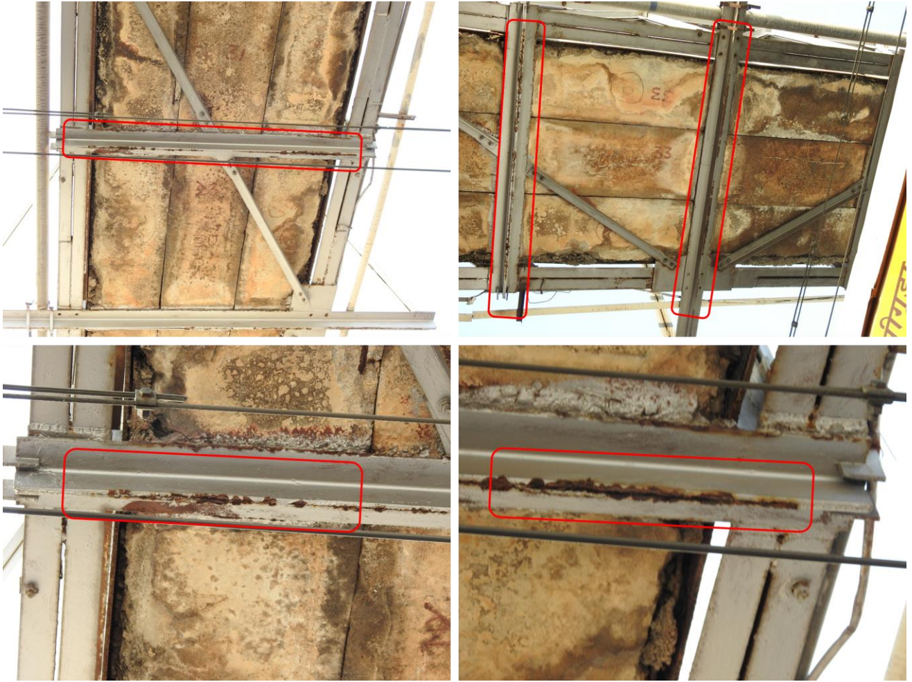
Fig 3.10: corrosion of floor beam in span-3
