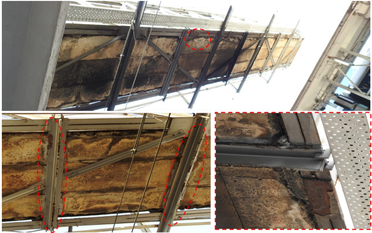
(c) Corrosion of floor beams and Bottom chord members in span 2.
