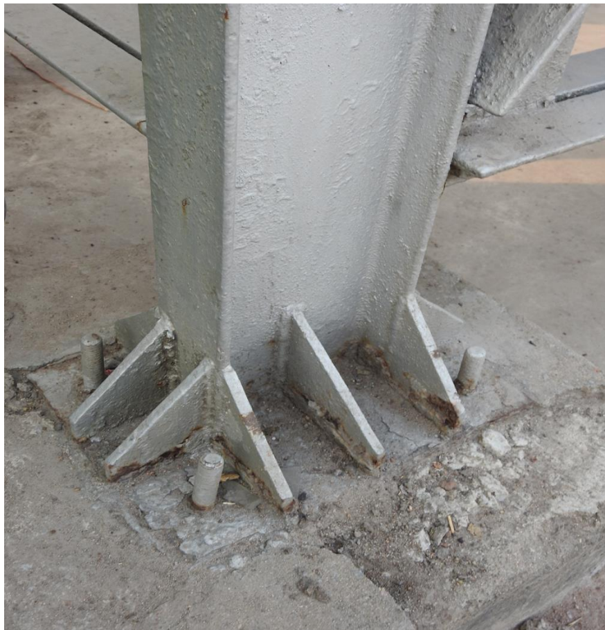
(b) Corrosion of Base plate at Trestle 1
