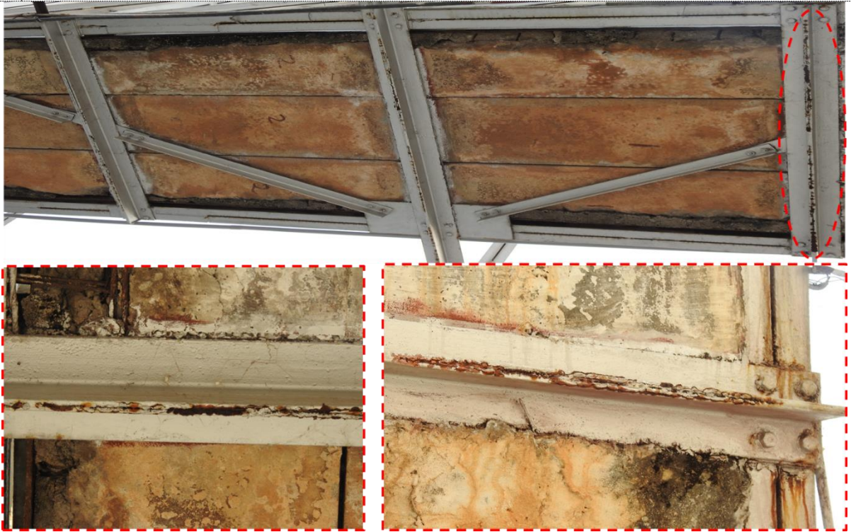
(a) Corrosion of Floor and bottom chord beams at span 1
