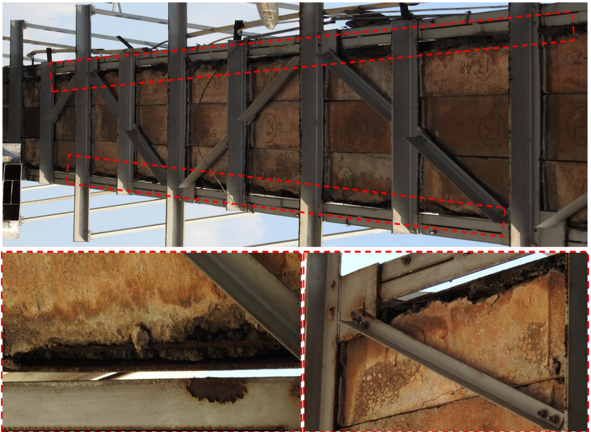
(b) Spalling at bottom chord and slab panels connecting joint along the length of FOB
