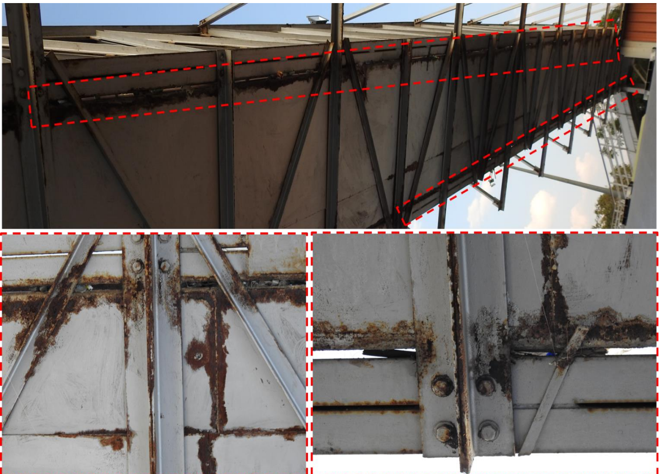
Fig: 3.16 corrosion of floor beam, joints and sacrificial plate and bottom chord joints
