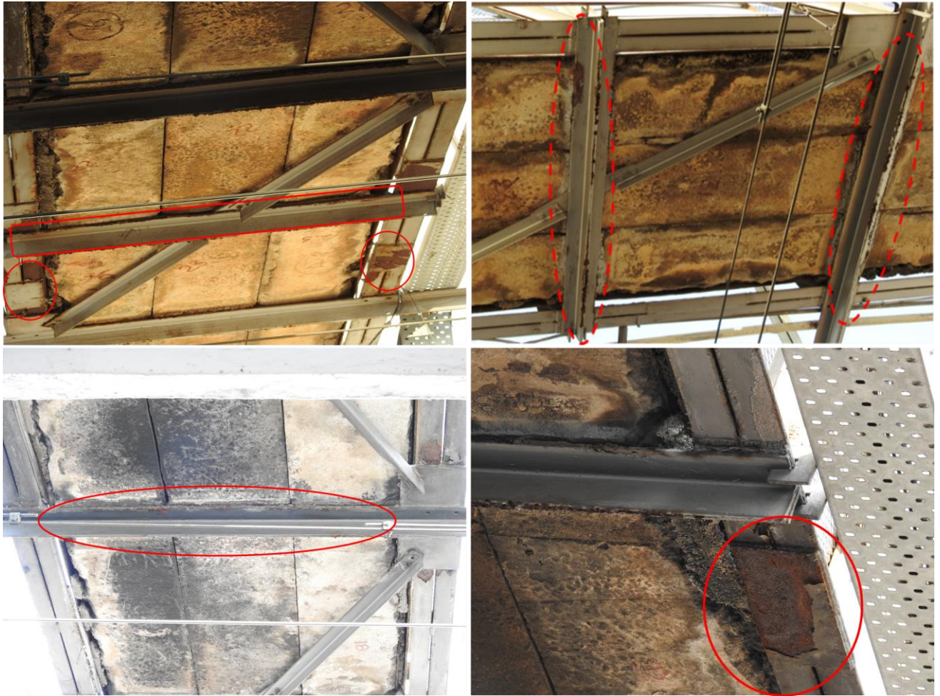
Fig 3.7: corrosion of floor beam, bottom chord and splice joint in span-2
