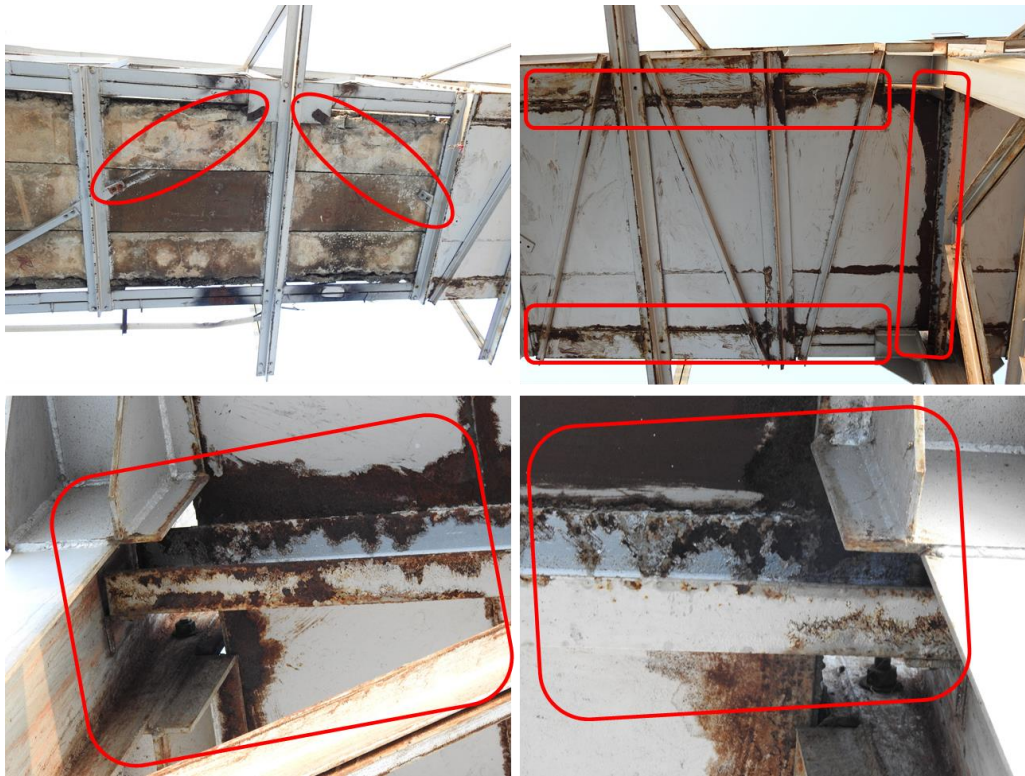
Fig 3.13: corrosion of floor beam and sacrificial plate and missing diagonal
