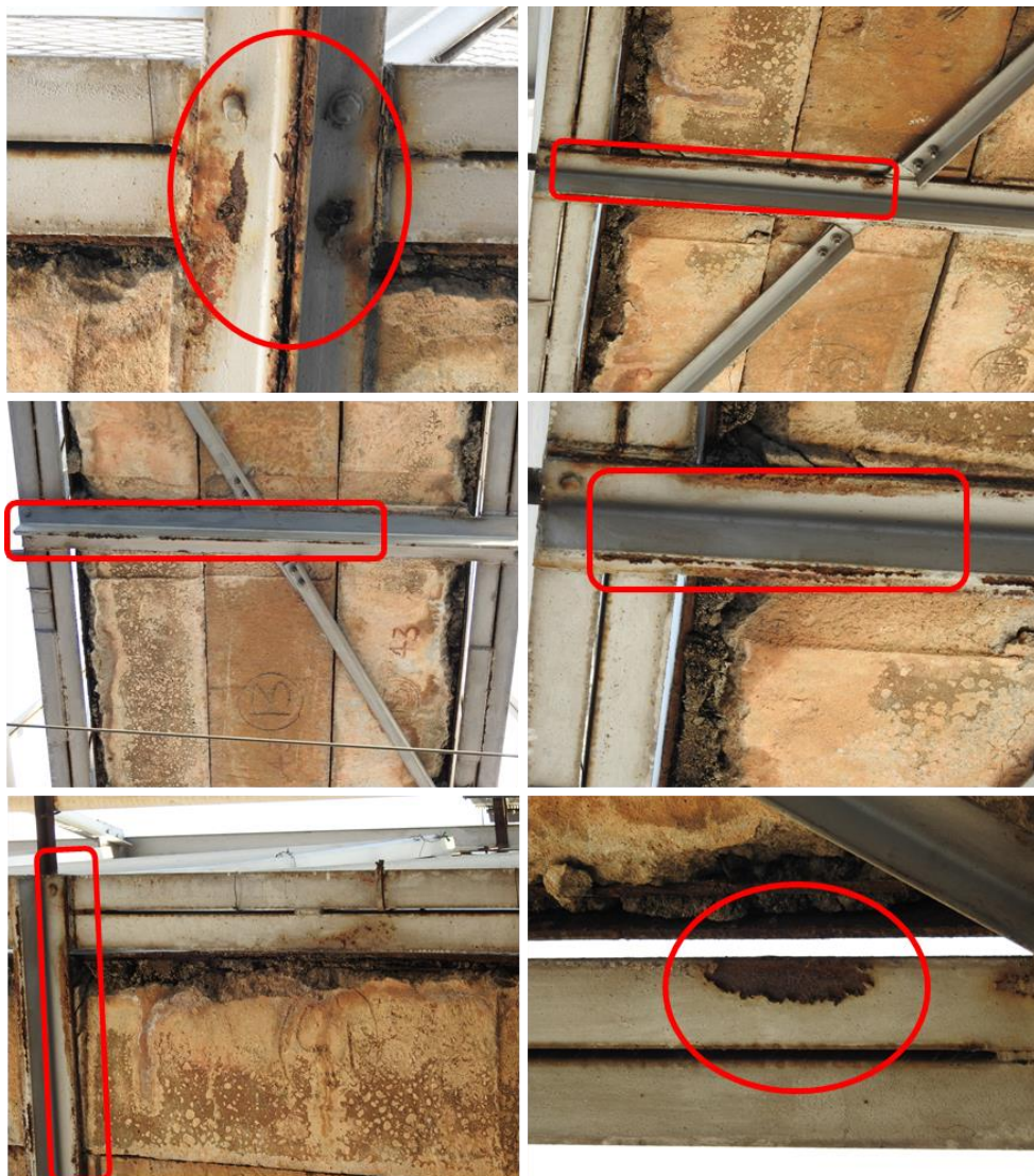
Fig 3.14: Corrosion of floor beams and bottom chord in span-4
