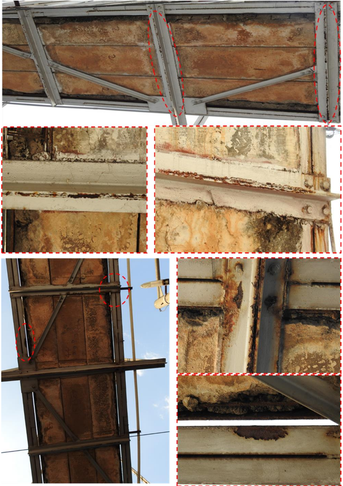
Fig 3.4: corrosion of floor beams in span-1
