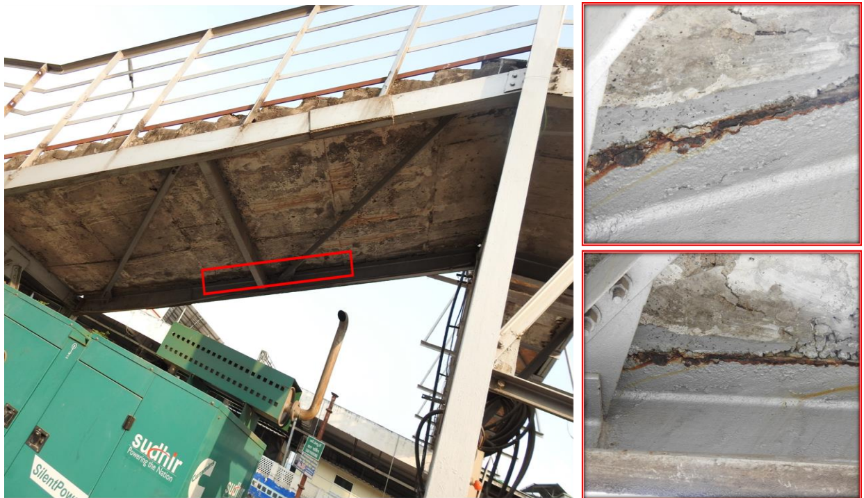
Fig 3.2: Corrosion of stinger beam near steel concrete joint at span-1
