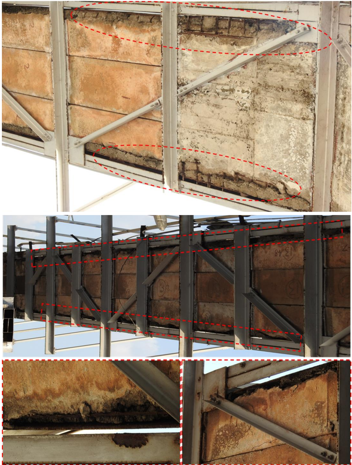
Fig 3.3: Exposed reinforcement in slab panels at span-1
