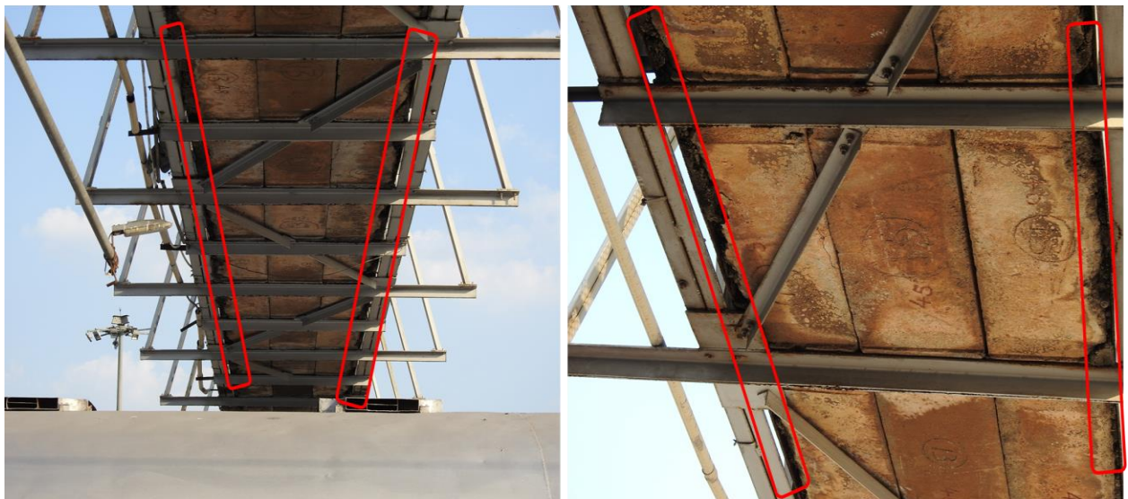
Fig 3.12: Exposed reinforcement in slab panels at span-4
