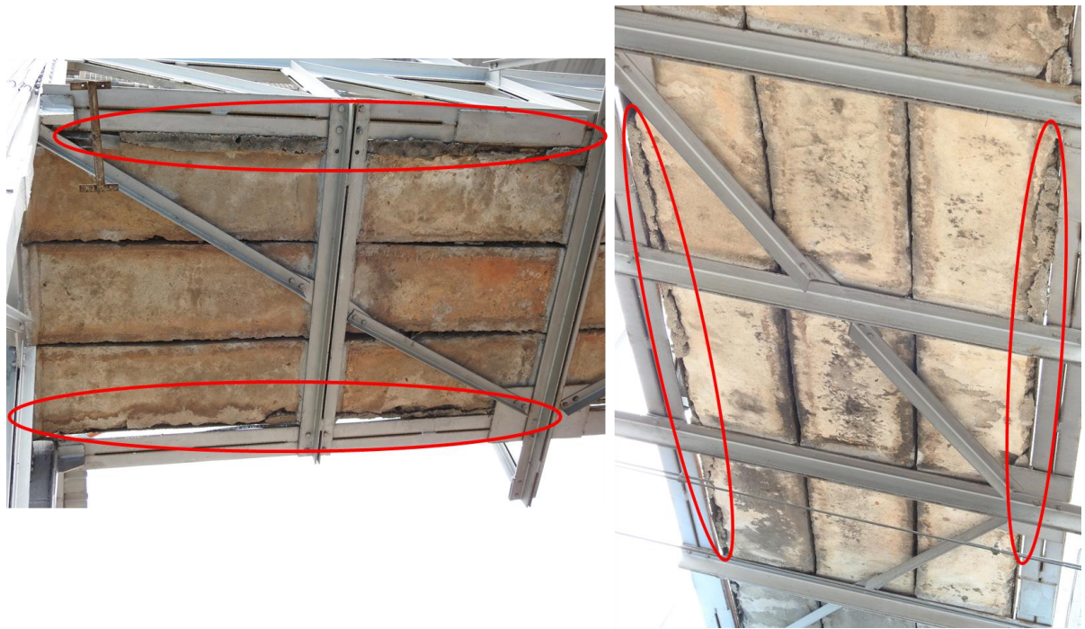
Fig 3.2: Exposed reinforcement and patchwork in slab panels at span-1
