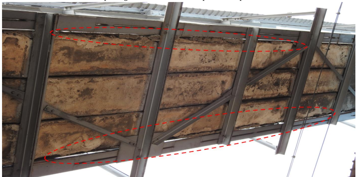
Spalling at bottom chord and slab panels connecting joint
