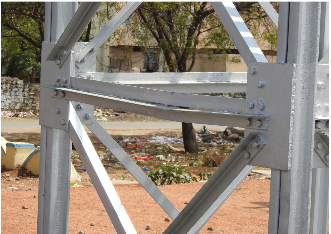
Fig 1.8: Deformation of bracings at trestle 4
