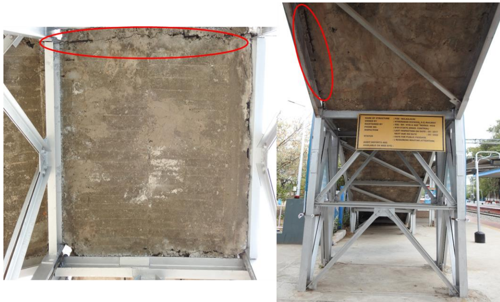
Fig: 3.3 Exposed reinforcement in mid landing and flight of staircase-1
