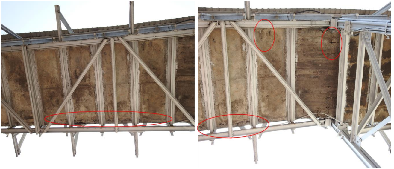
Fig: 3.8 Exposed reinforcement in pathway of span-3
