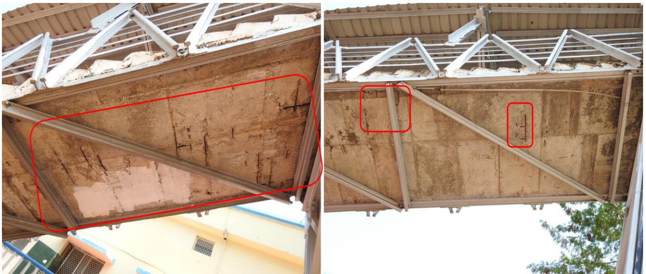
Fig: 3.10 Exposed reinforcement in staircase-3
