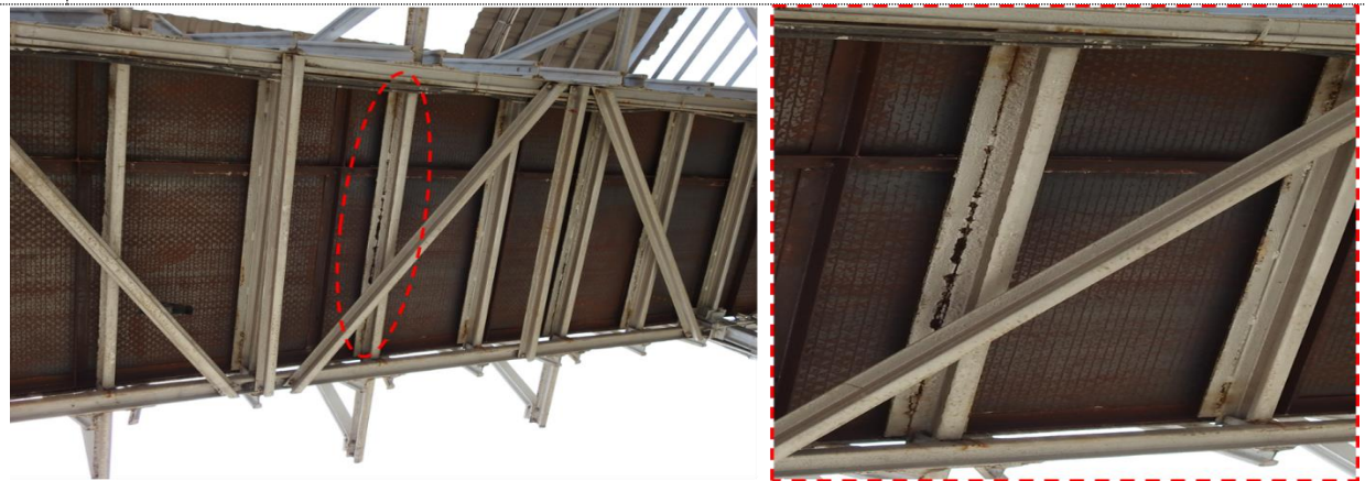
Corrosion of Floor beams
