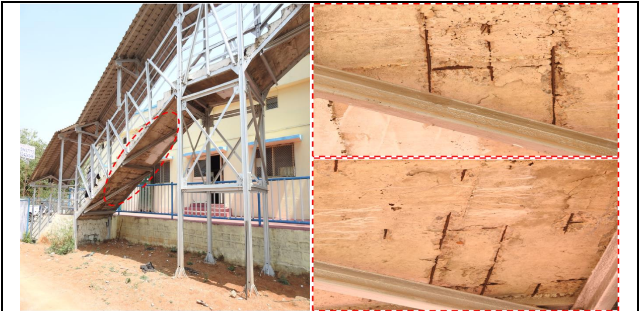
Spalling at stair case 3
