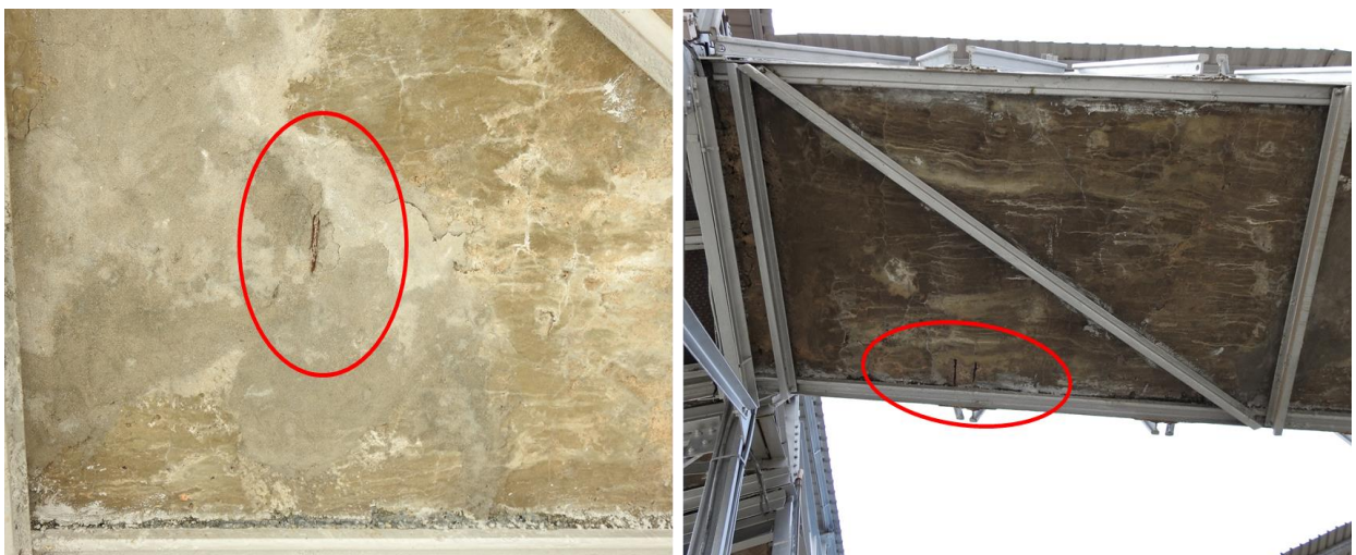
Fig: 3.6 Exposed reinforcement in flight of staircase-2
