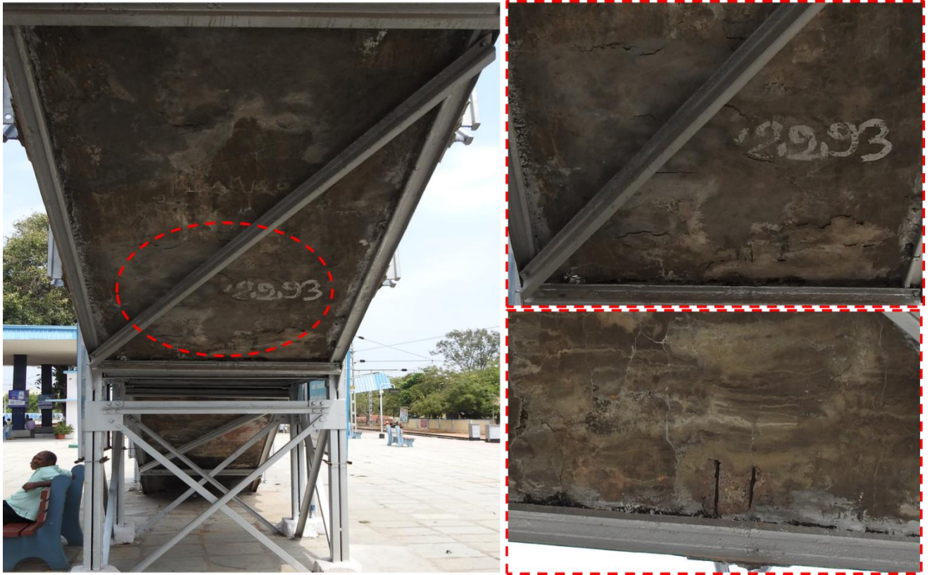
Fig 1.9: Patch work observed at staircase 2
