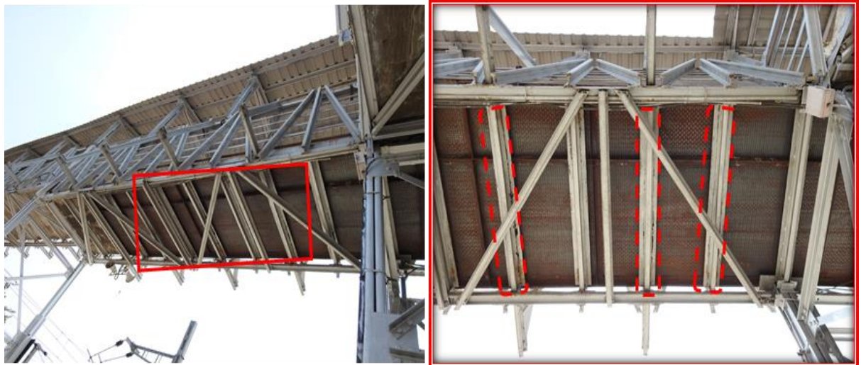
Fig: 2.5 Corrosion of floor beams in span-2
