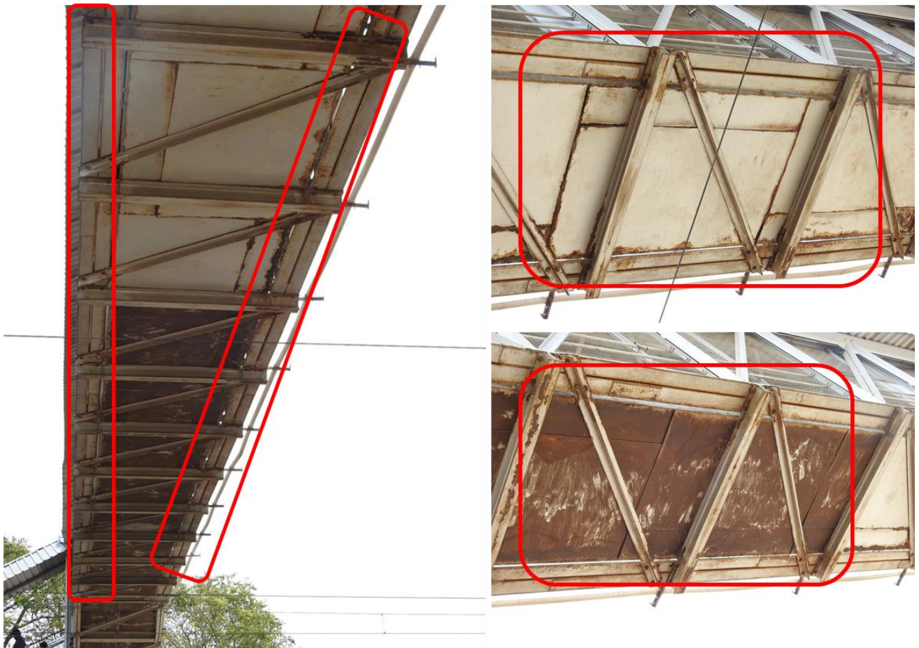
Fig: 3.6 corrosion of bottom chord and sacrificial plate at span-2
