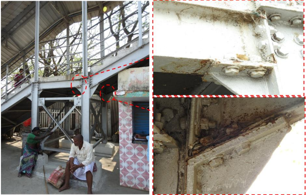
Fig: 3.3 Corrosion of bolts near beam column joint at span-1
