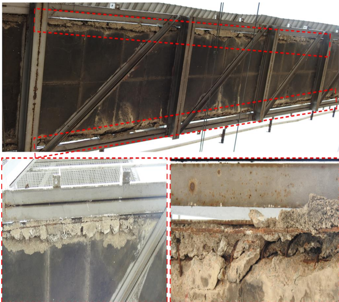
Fig: 3.2 Exposed reinforcement in slab at pathway of span-1
