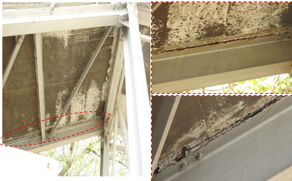
corrosion observed at Stringer beam (steel concrete joint)
