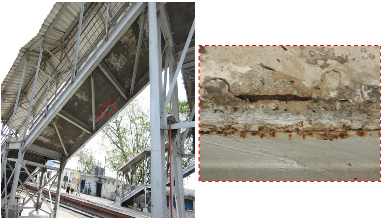
Fig: 3.4 spalling and exposed reinforcement at staircase-2
