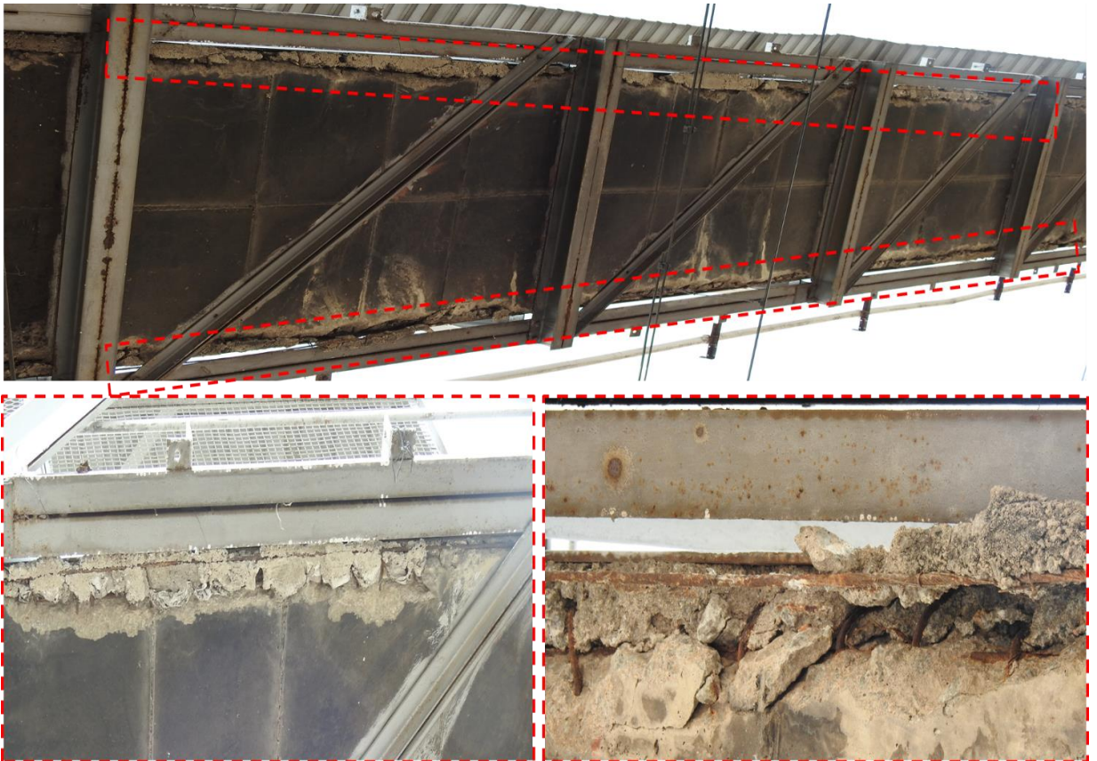
Spalling and reinforcement exposure
