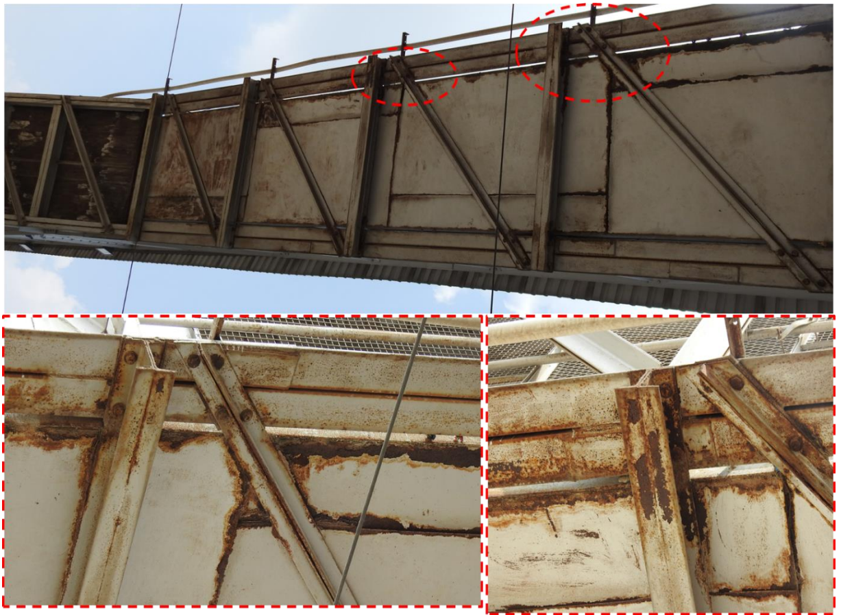
Corrosion of floor beam joints of span 3
