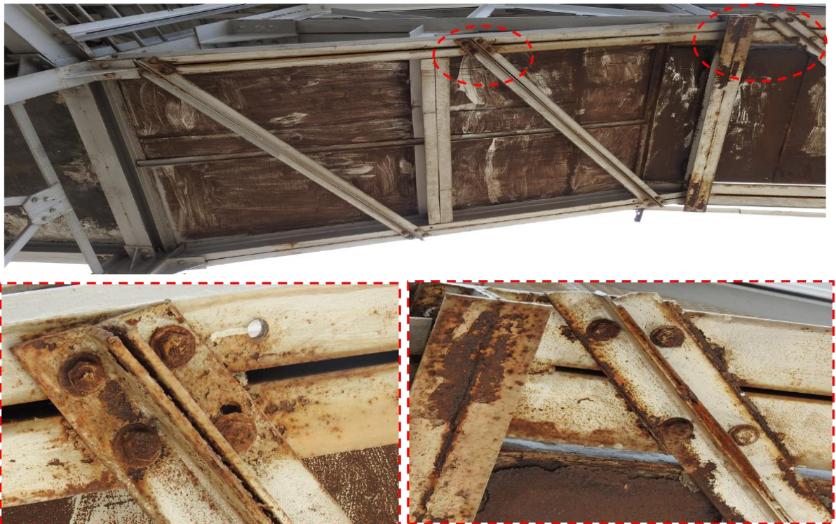
Corrosion observed in Floor beams joints of span 2
