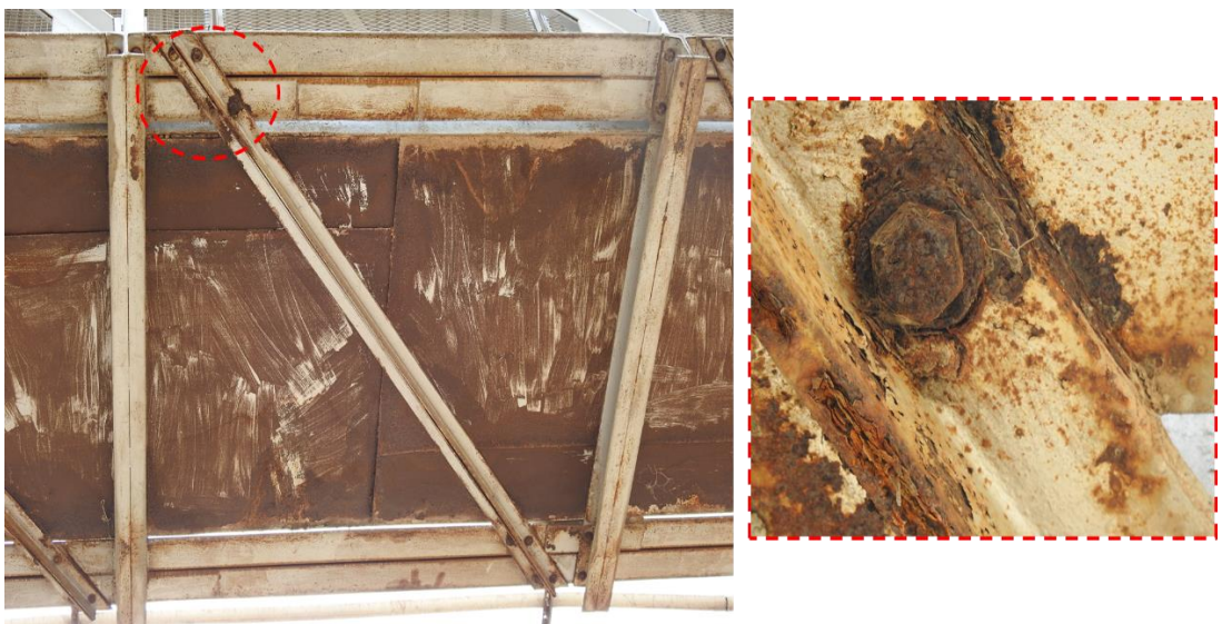
Fig: 3.8 corrosion of bolts at span 2
