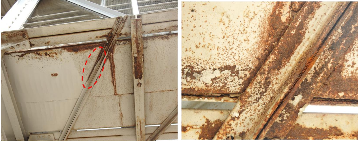
Fig: 3.11 Corrosion of diagonal and sacrificial plate at span-3
