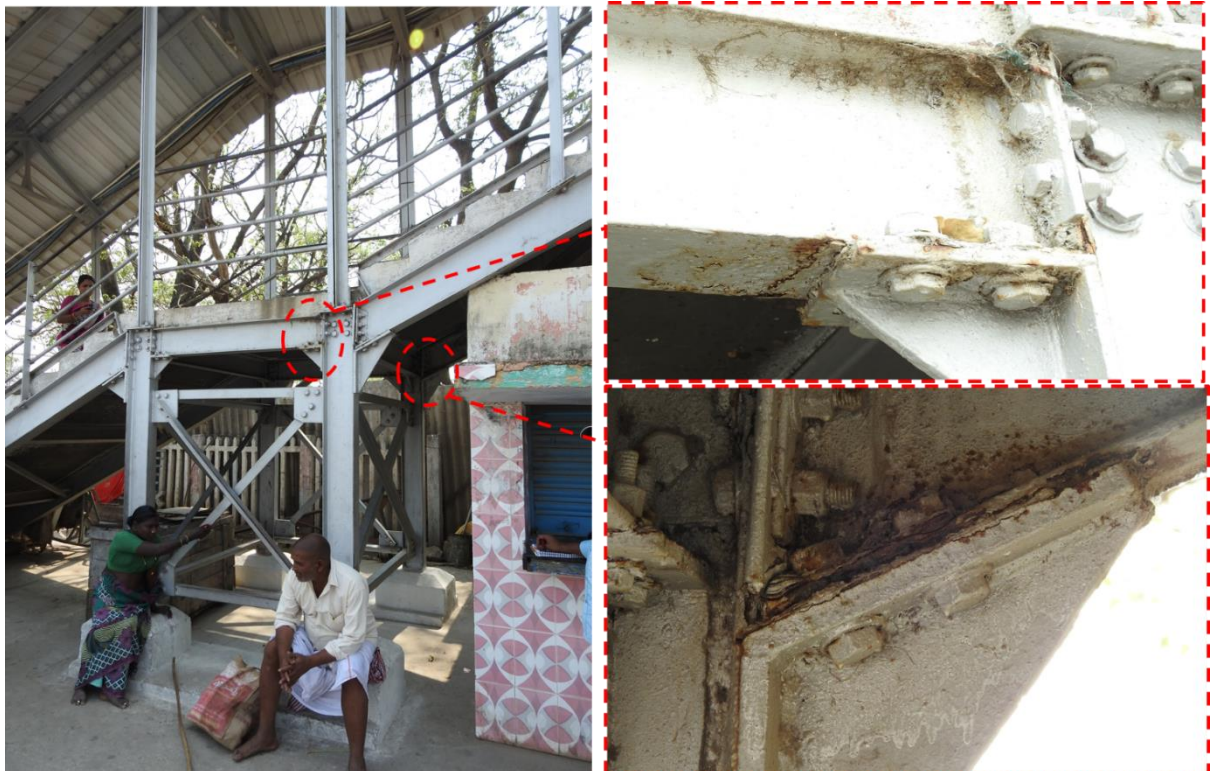
Corrosion at mid landing beam column joint.
