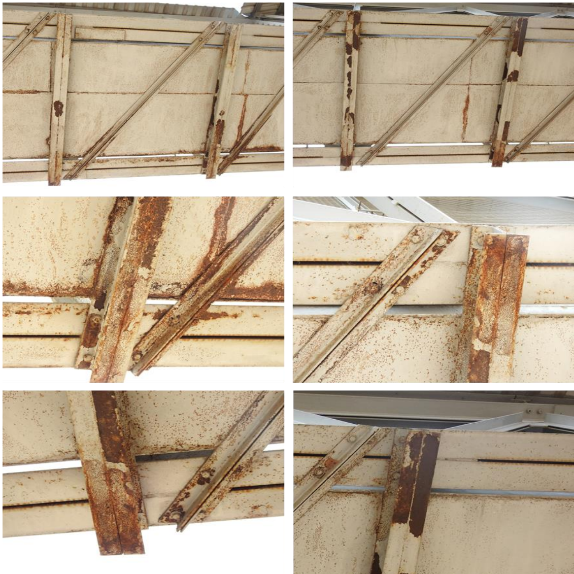
Fig: 3.10 Corrosion of floor beams, diagonals and bolts at span-3
