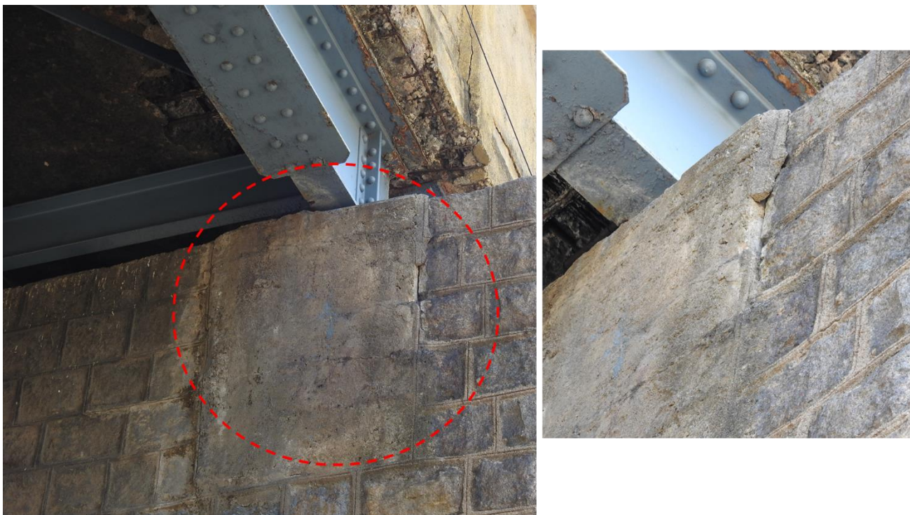
Fig: 1.12 pointing failure observed at the bed block
