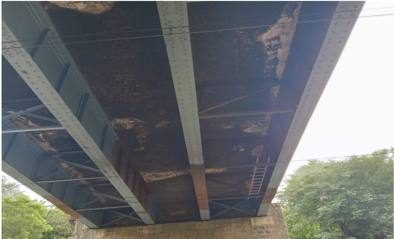
Fig:1.2 Bottom view of Slab
