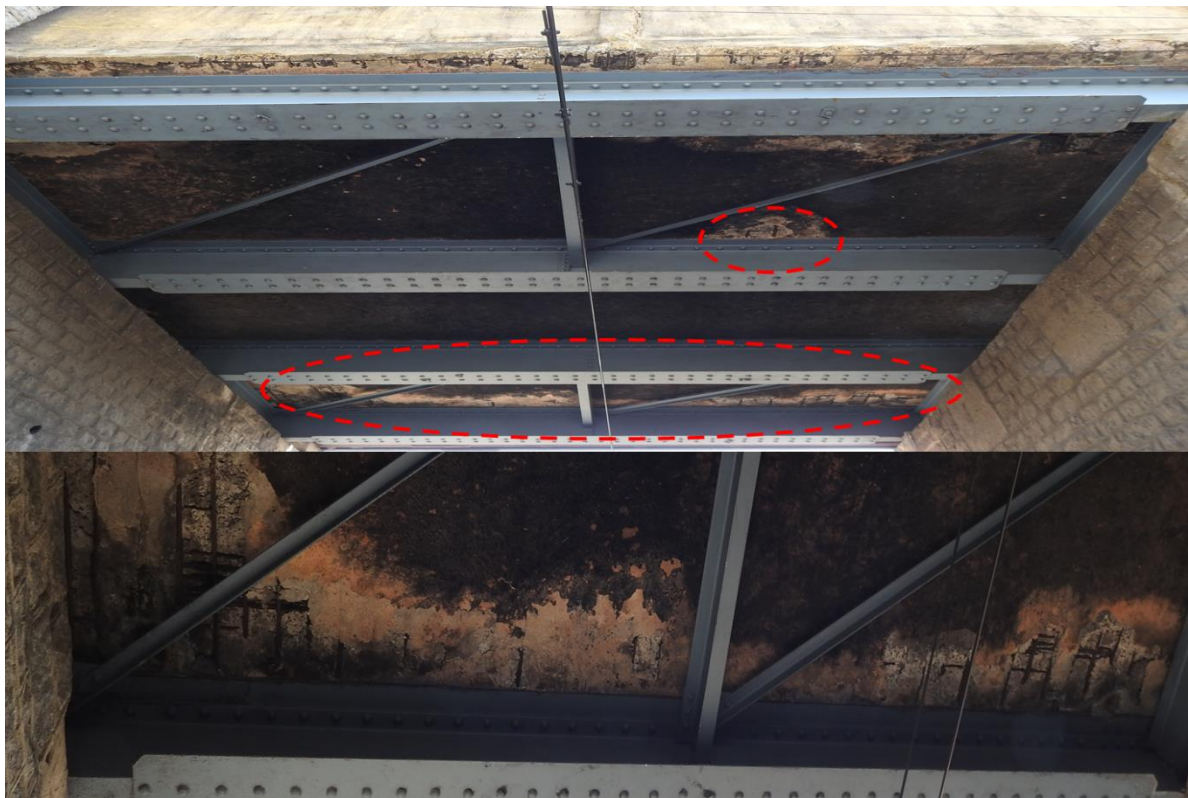
Fig: 1.8 Spalling and reinforcement exposed at span 1
