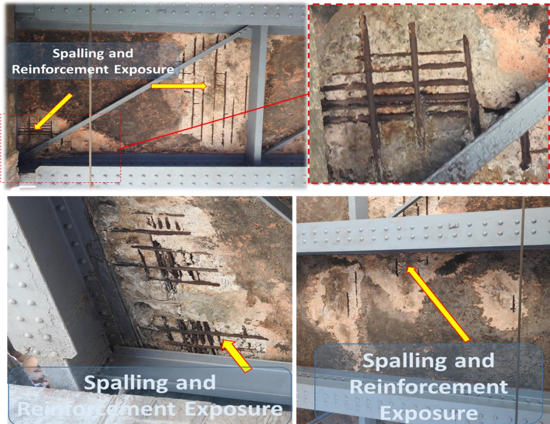
Fig 3.2: Damage locations identified in span 1 at “a, b, c & d”
