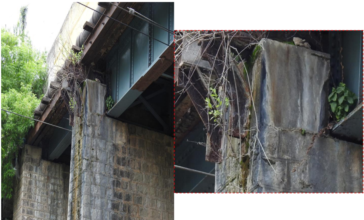
Fig: 1.3 Vegetation, algae growth, leaching, and cracks observed at Piers
