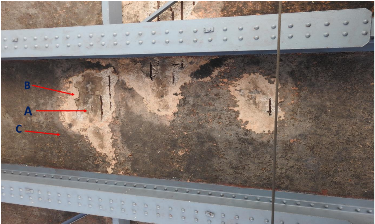
Fig:1.10 Patch work observed (A- original concrete, B-old patch work, C-new patch work)
