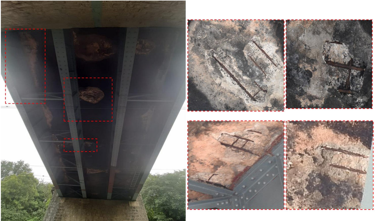
Fig:1.4 Exposed reinforcement observed in span 2
