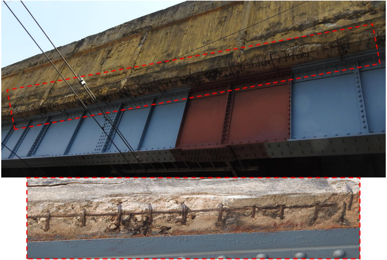
Fig: 1.7 Spalling and reinforcement exposed at overhang portion of slab due to less cover
