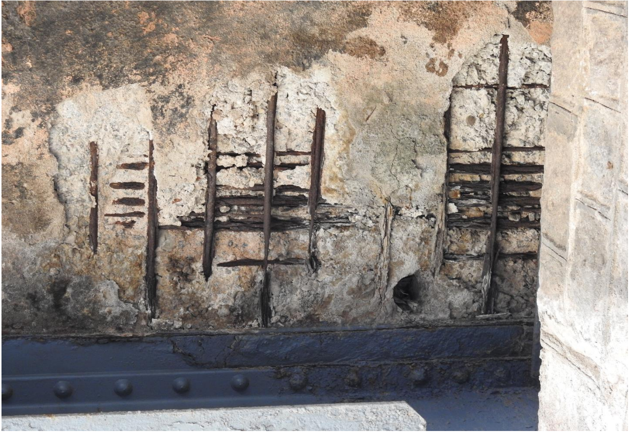
Fig: 1.11 Exposed reinforcement due to improper drain
