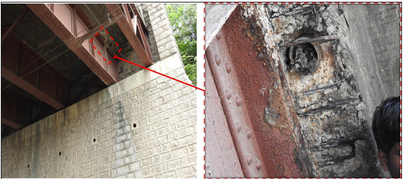
Fig 2.5: Corrosion and steel flaking at top flange of beam
