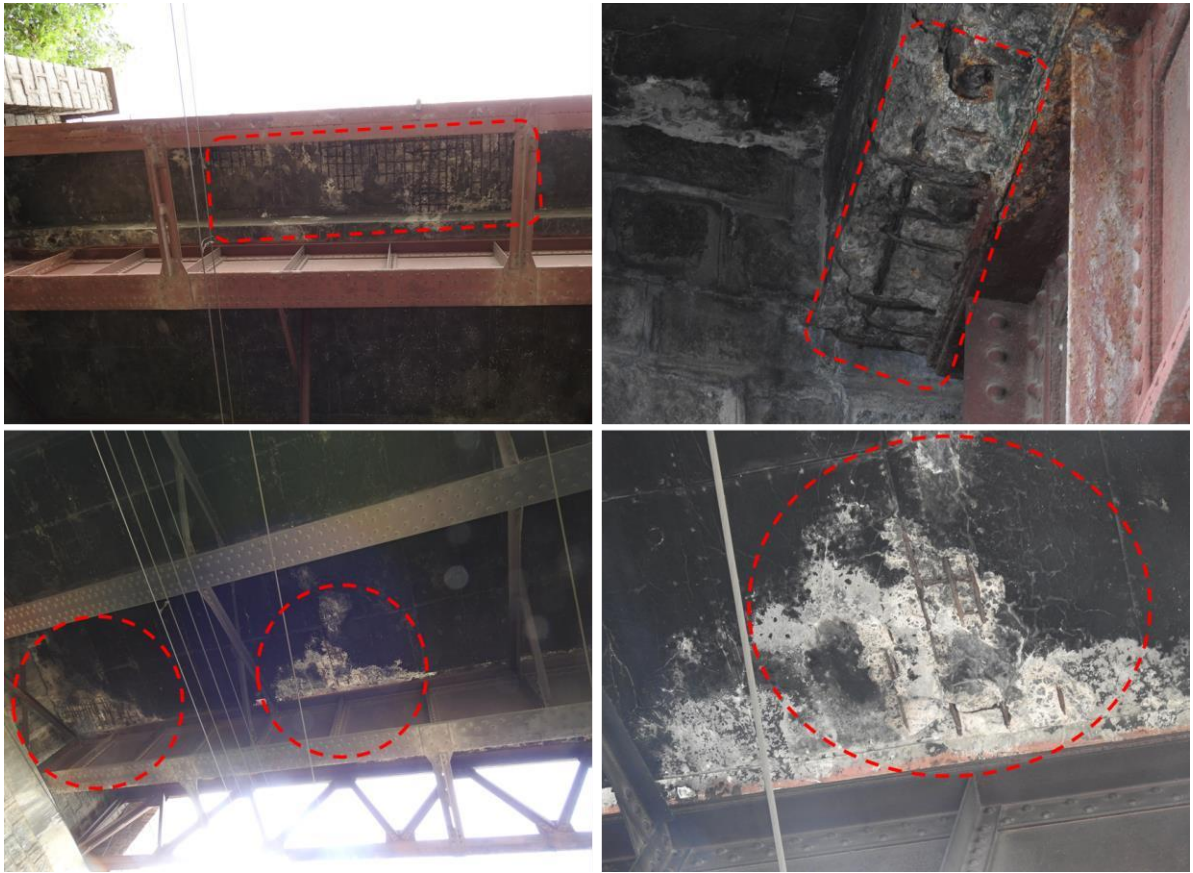
Fig 2.2: Damage locations identified in deck slab
