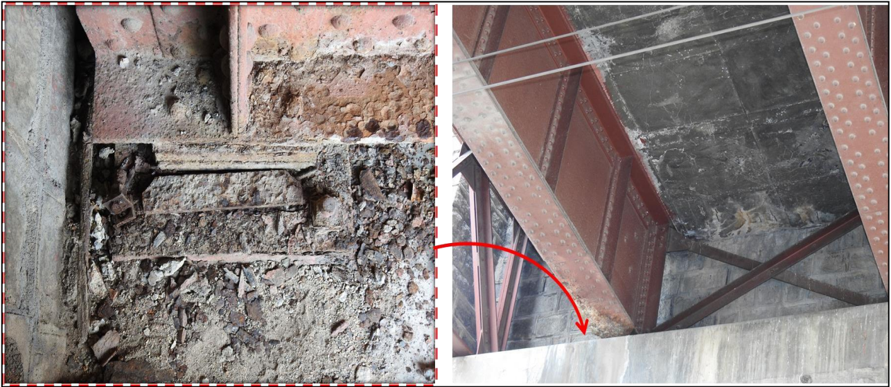
Fig 2.4: corrosion of bearing plate
