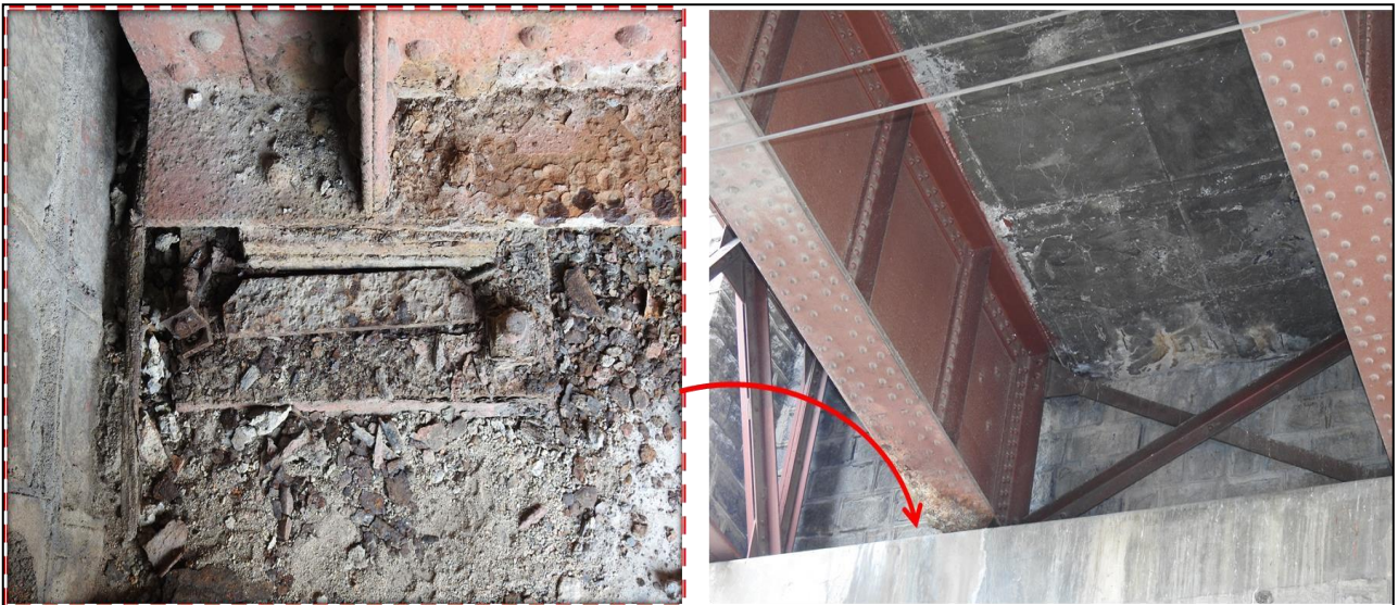
Fig 1.5: Base plate corrosion
