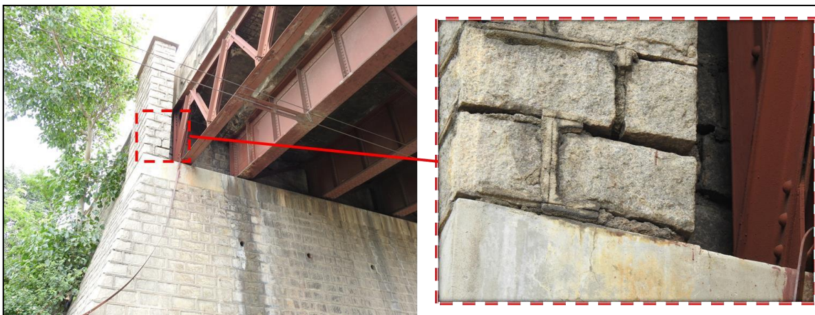
Fig 1.2: failure of pointing near abutments
