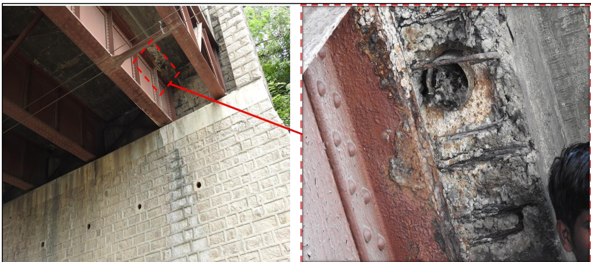
Fig 1.3: Reinforcement exposed and corrosion of main girder
