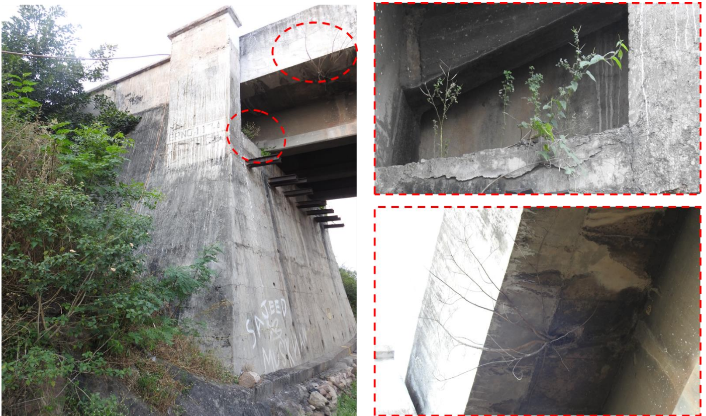
Fig 12: Vegetation observed at abutment and Drainage spouts
