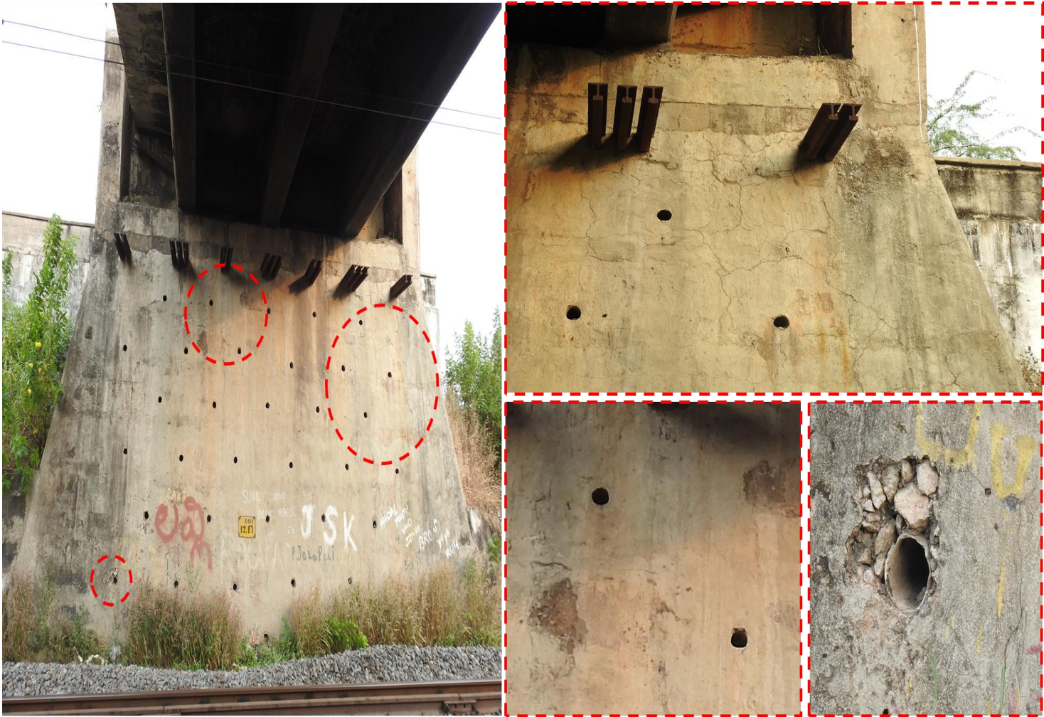
Fig 11: Shrinkage cracks and minor spalling at Abutment 1
