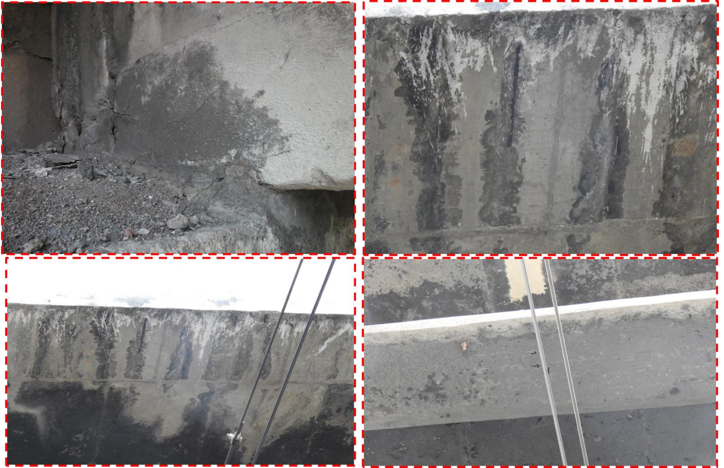
Fig: 15 Spalling of concrete at girders and overhang slab portion
