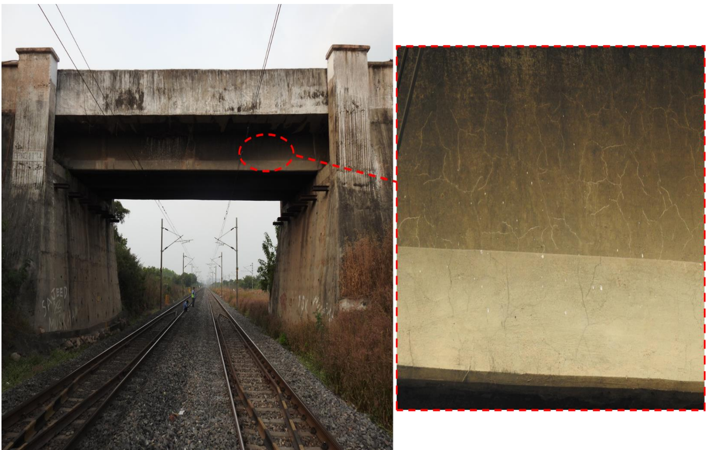
Fig 8: shrinkage cracks at main girders
