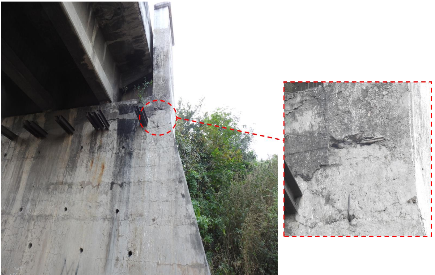
Fig 7: Minor Spalling, leaching at Abutment
