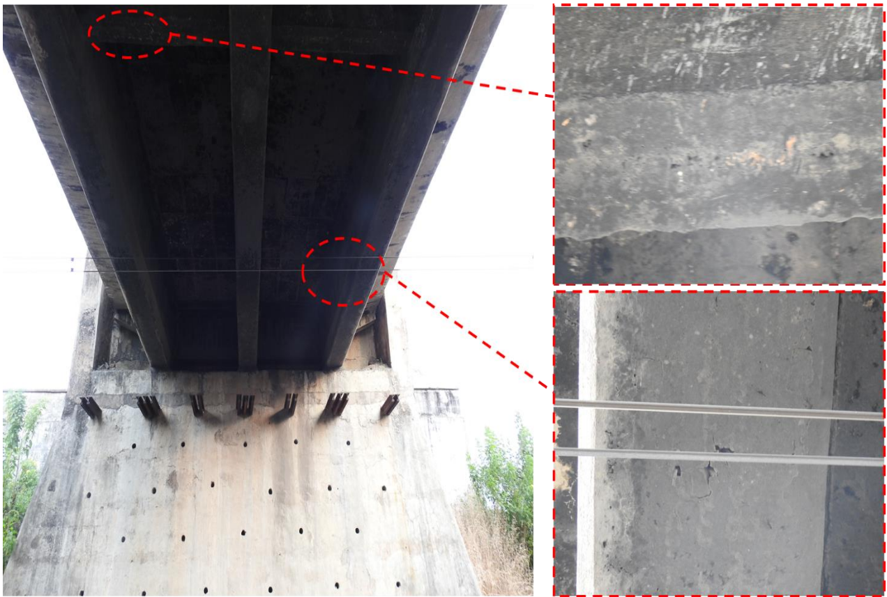
Fig 9: Minor spalling at secondary and main girder
