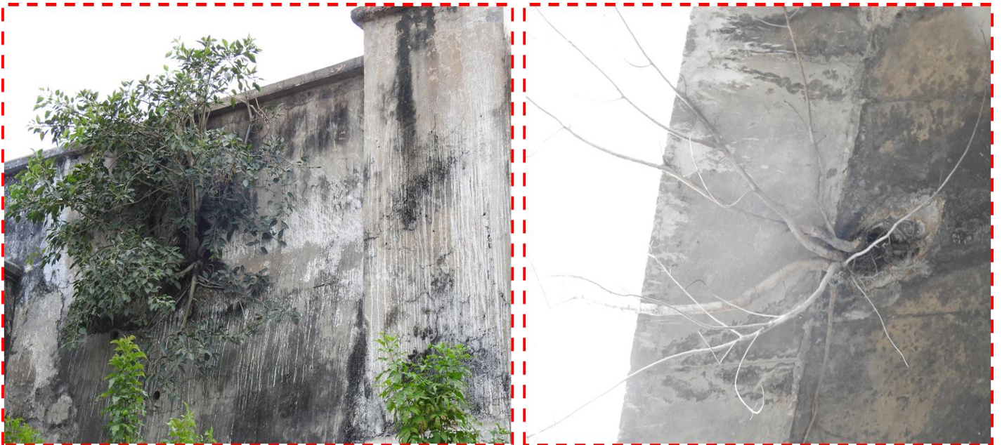
Fig: 16 Vegetation growth at abutments and slab
