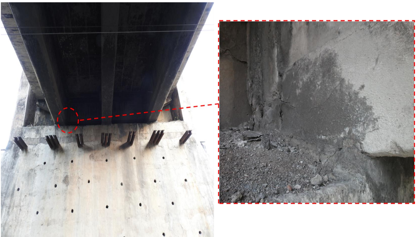
Fig 6: Spalling and crack at main girder resting location
