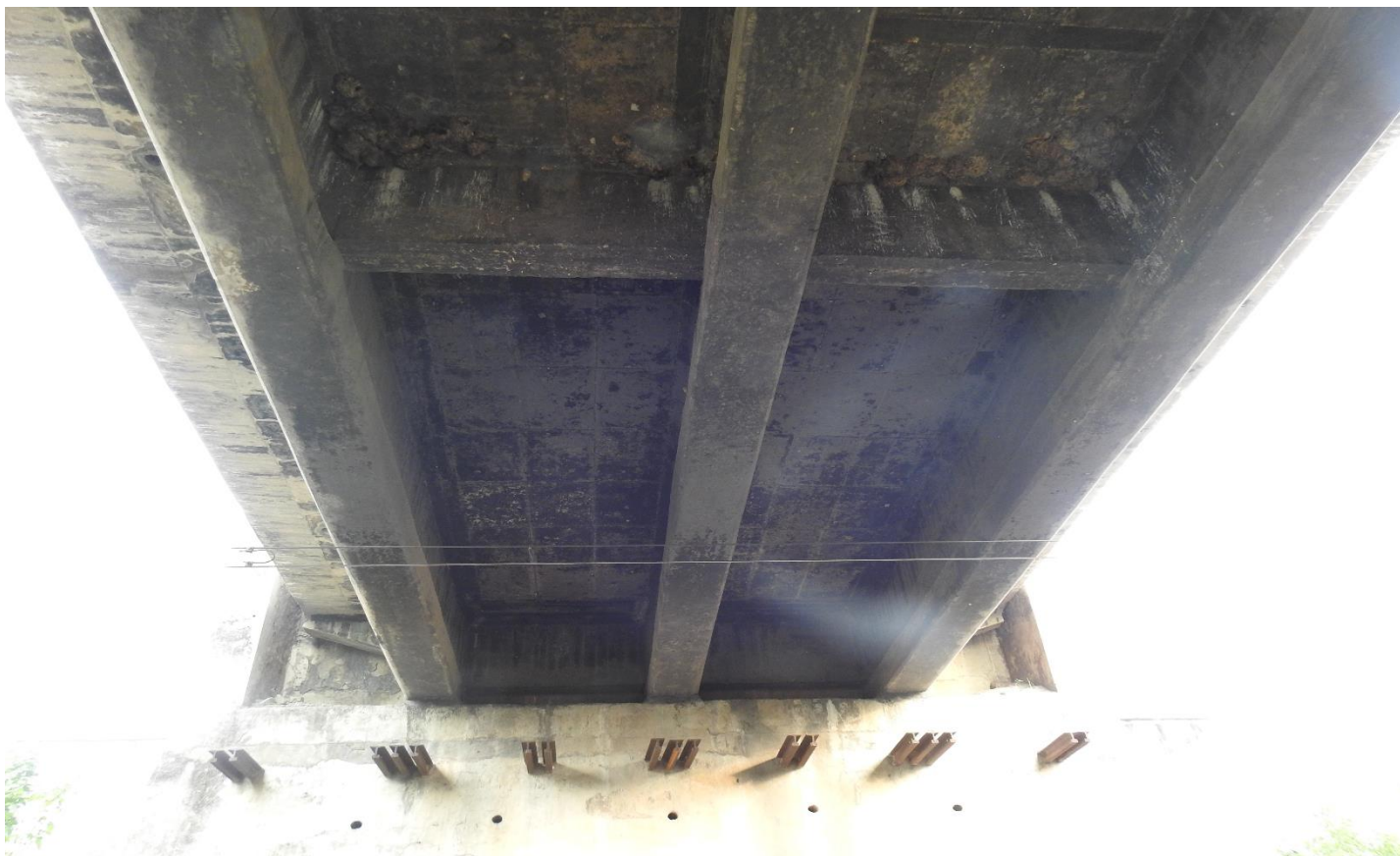
Fig: 3 Bottom view, Leaching observed
