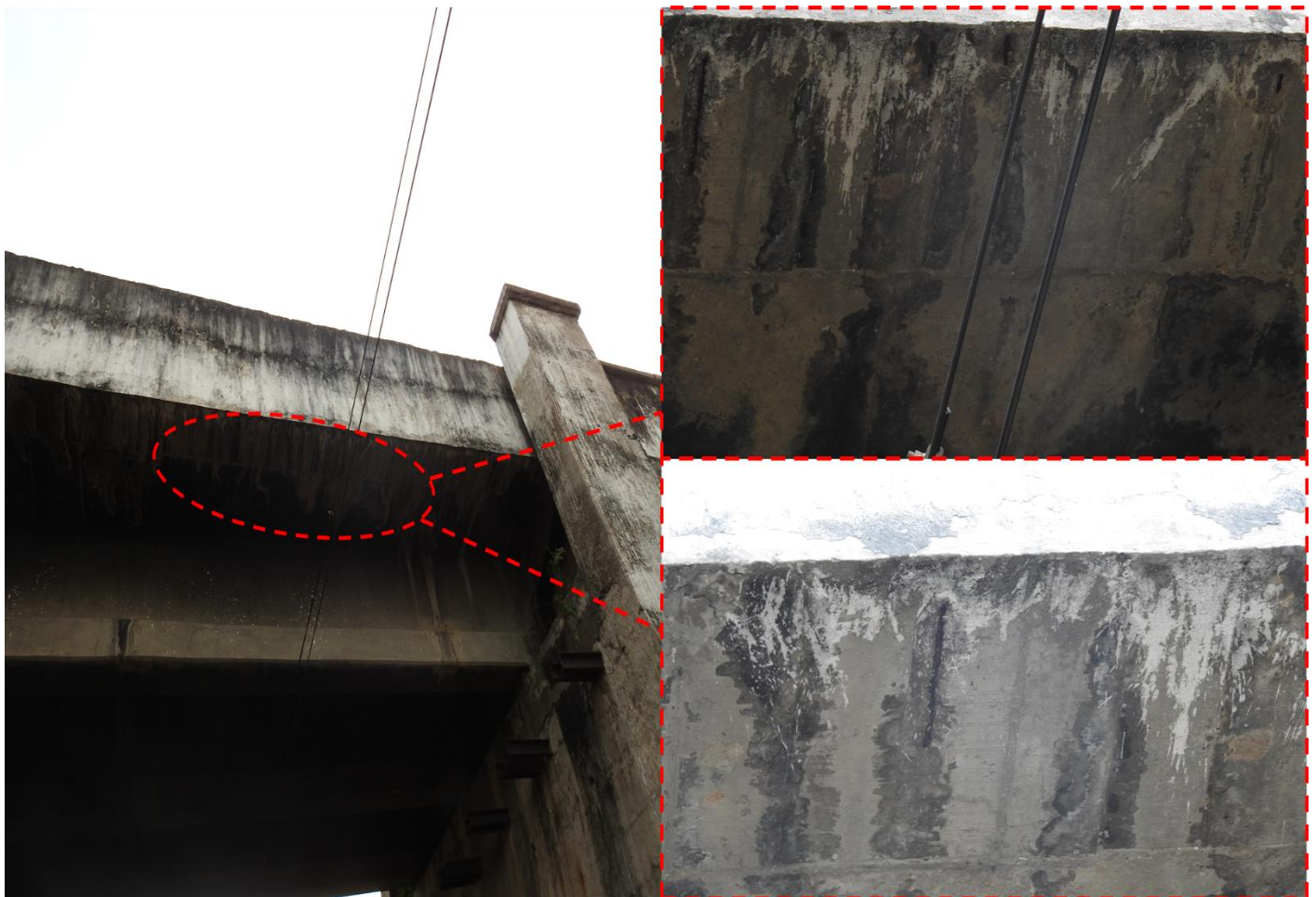
Fig 10: Spalling at Overhang Slab portion
