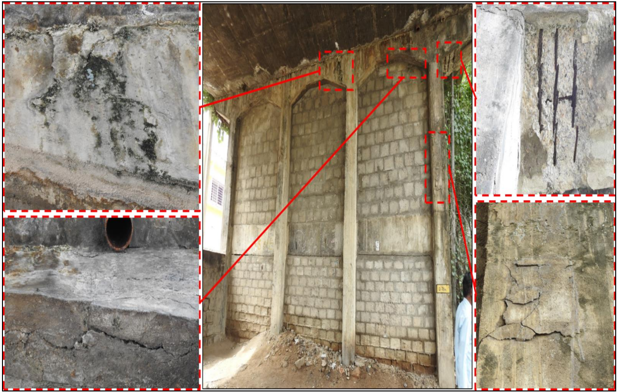
Fig 4: Cracks, Spalling & Reinforcement exposure observed in Pier-1
