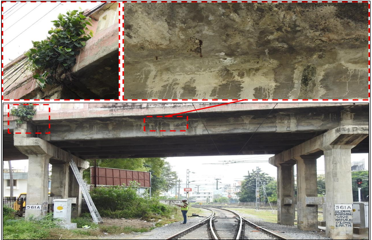
Fig 10: Vegetation at Expansion joint & Spalling at Girder and Slab of Span-3
