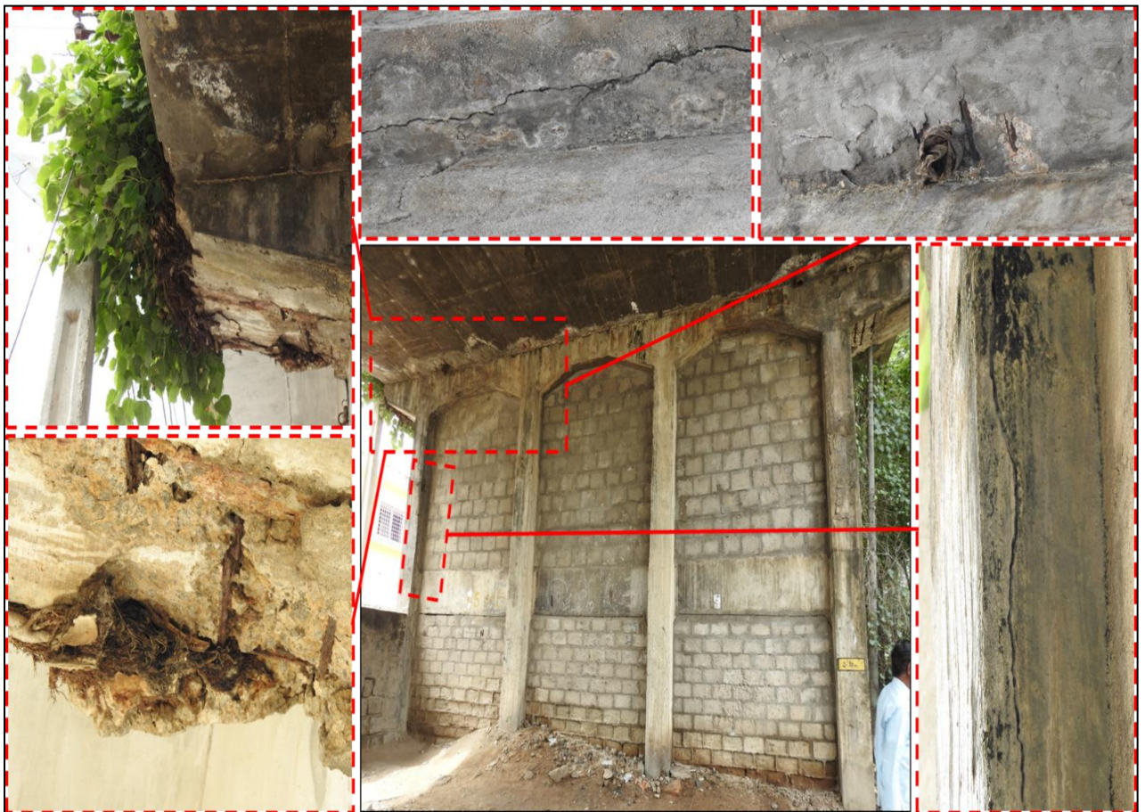
Fig 5: Cracks, Vegetation & leaching observed on Pier-1
