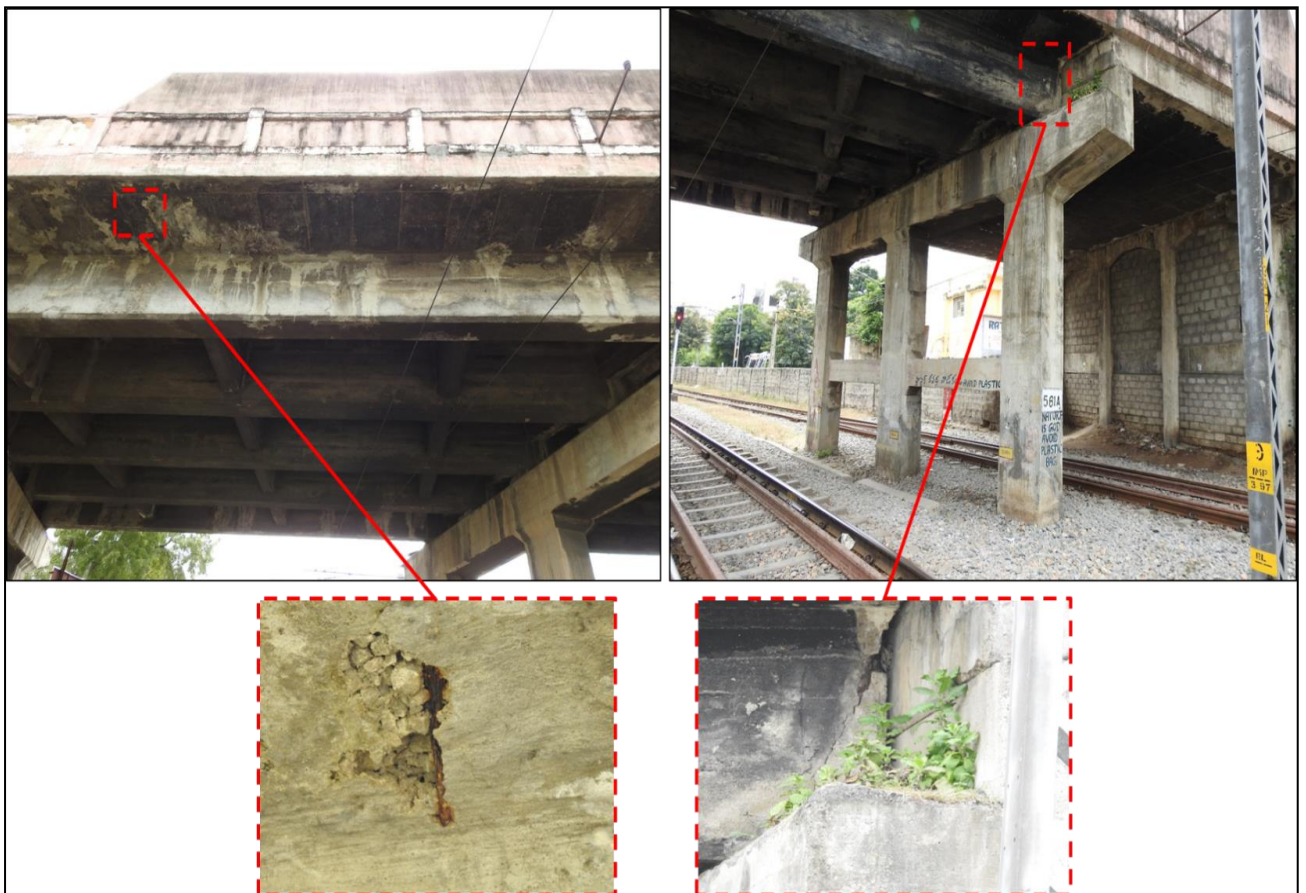
Fig 13: Spalling, Vegetation & Reinforcement exposure at Girder & Slab
