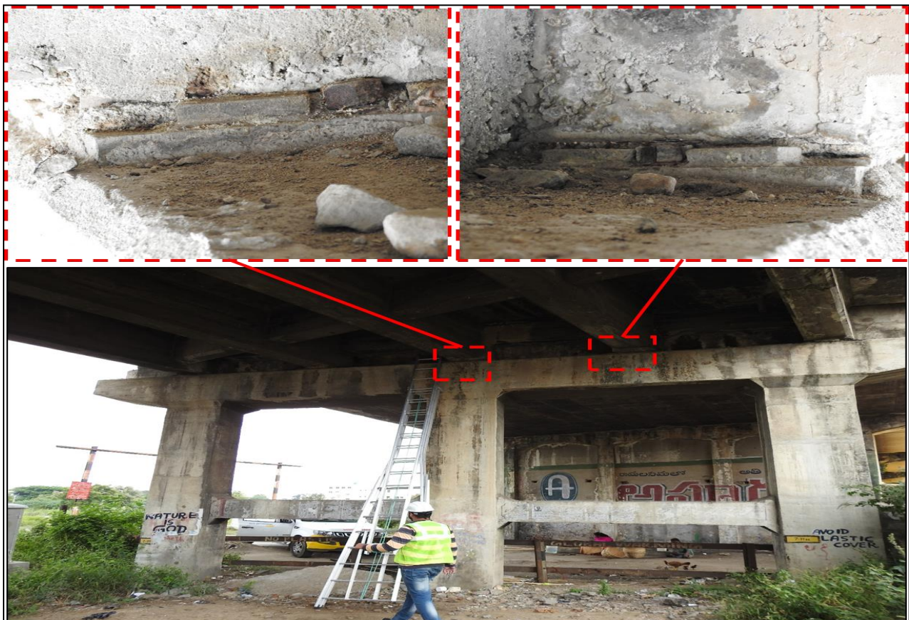
Fig 11: Debris accumulated at Bearings
