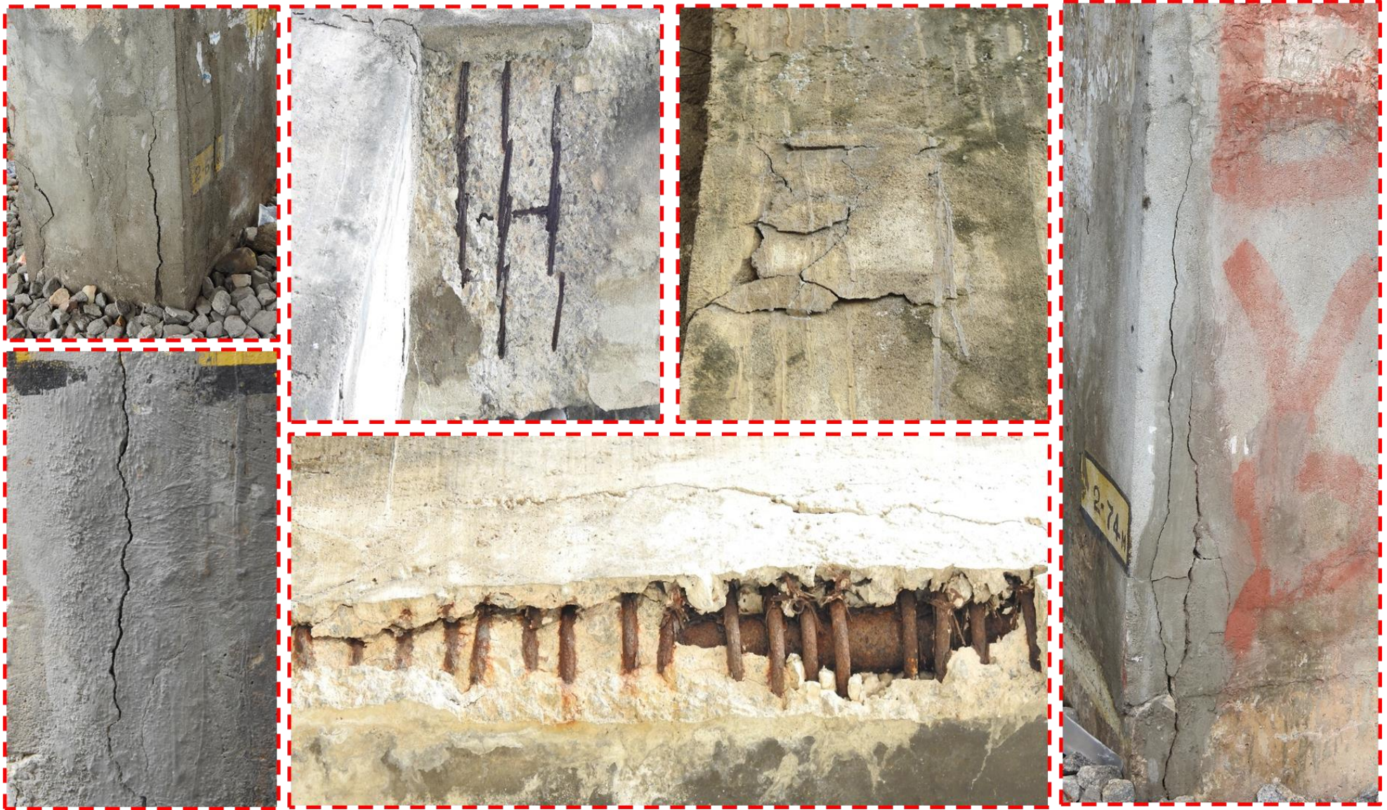
Fig: 19 Major Cracks at Columns and Reinforcement exposure.
