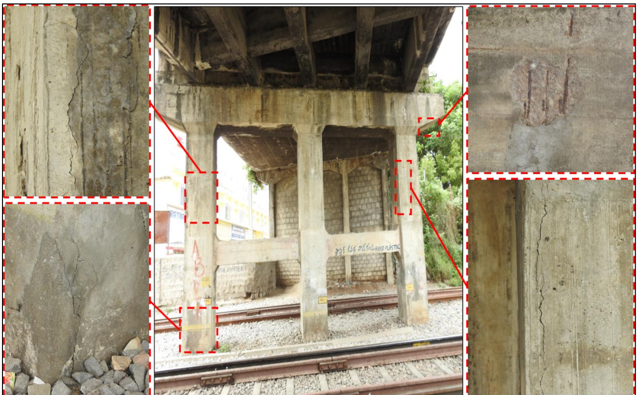
Fig 7: Cracks, Spalling & Reinforcement exposure observed in Pier-2
