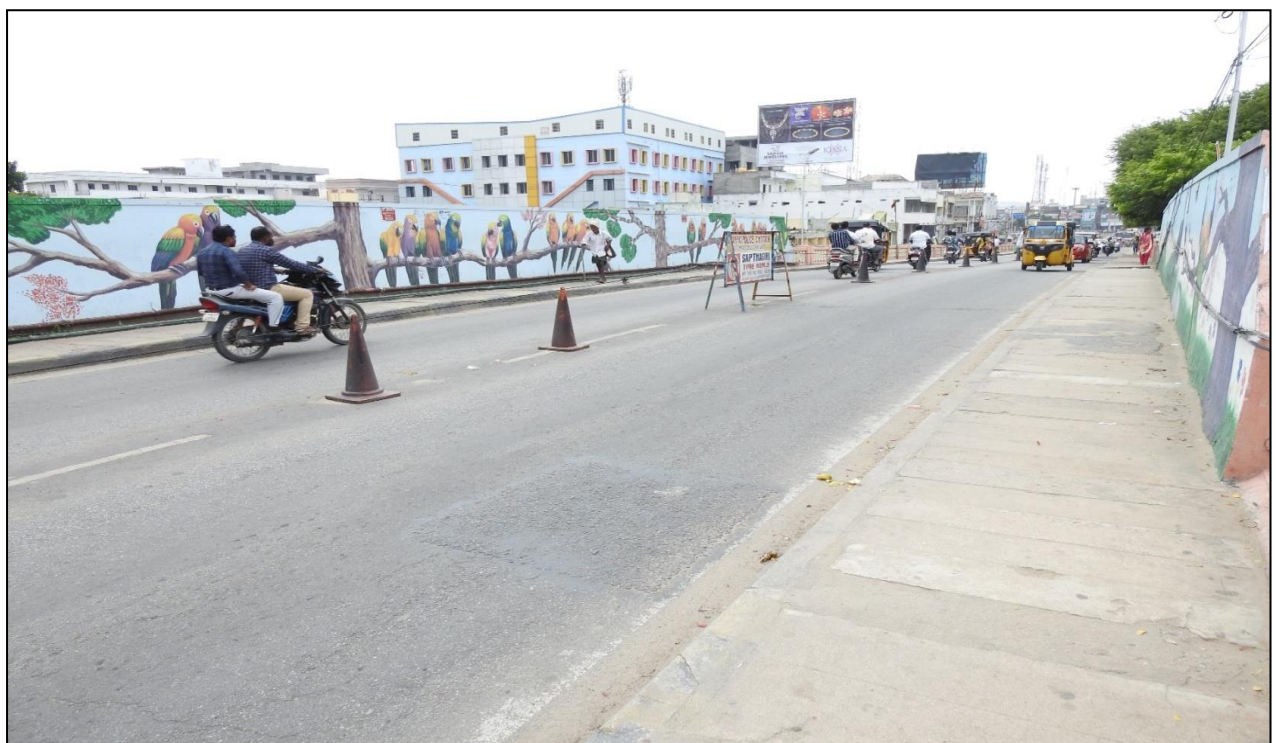
Fig 3: Top View of the bridge / Condition of wearing course
