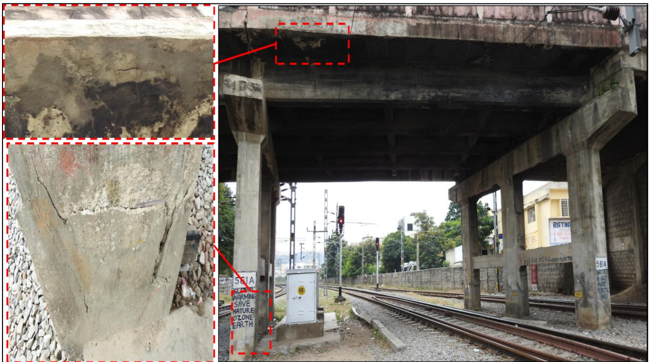
Fig 9: Cracks at overhang portion of slab and spalling at Pier-3 column
