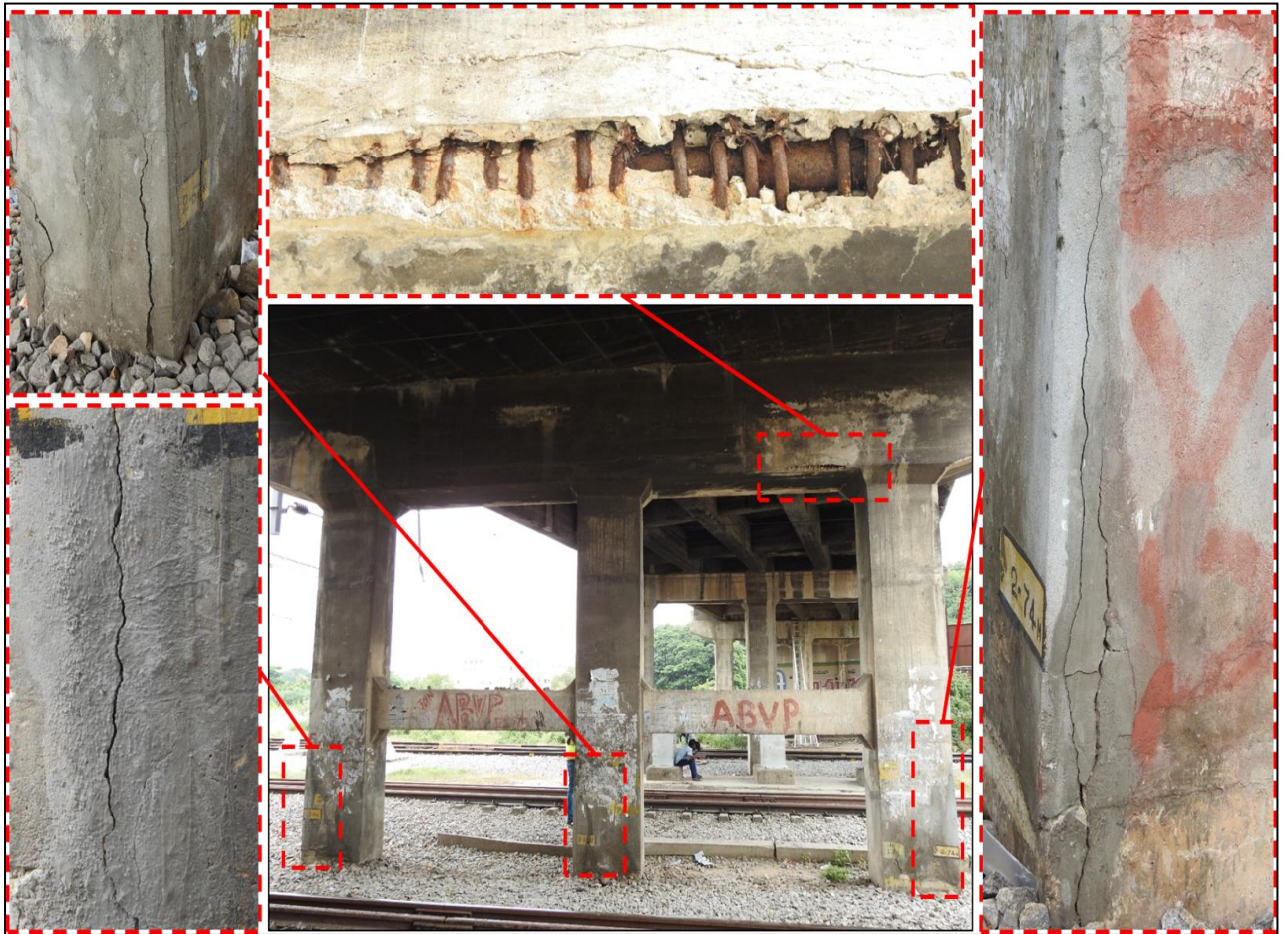
Fig 6: Cracks, Spalling & Reinforcement exposure observed in Pier-2
