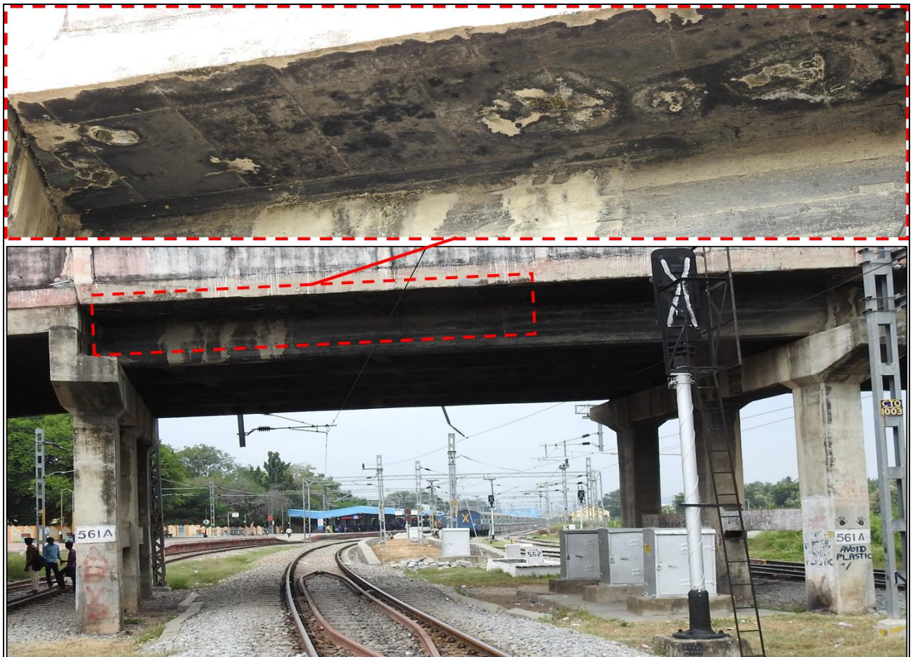
Fig 8: Leaching at overhang portion of Slab of Span-2
