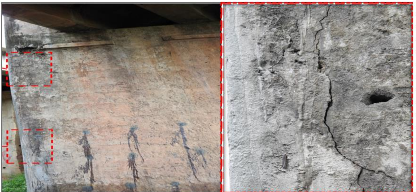
Fig 14: cracks observed at Abutment.
