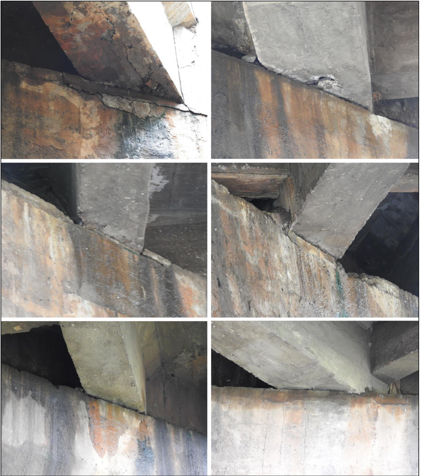
Fig 8: Distresses observed at Bearings
