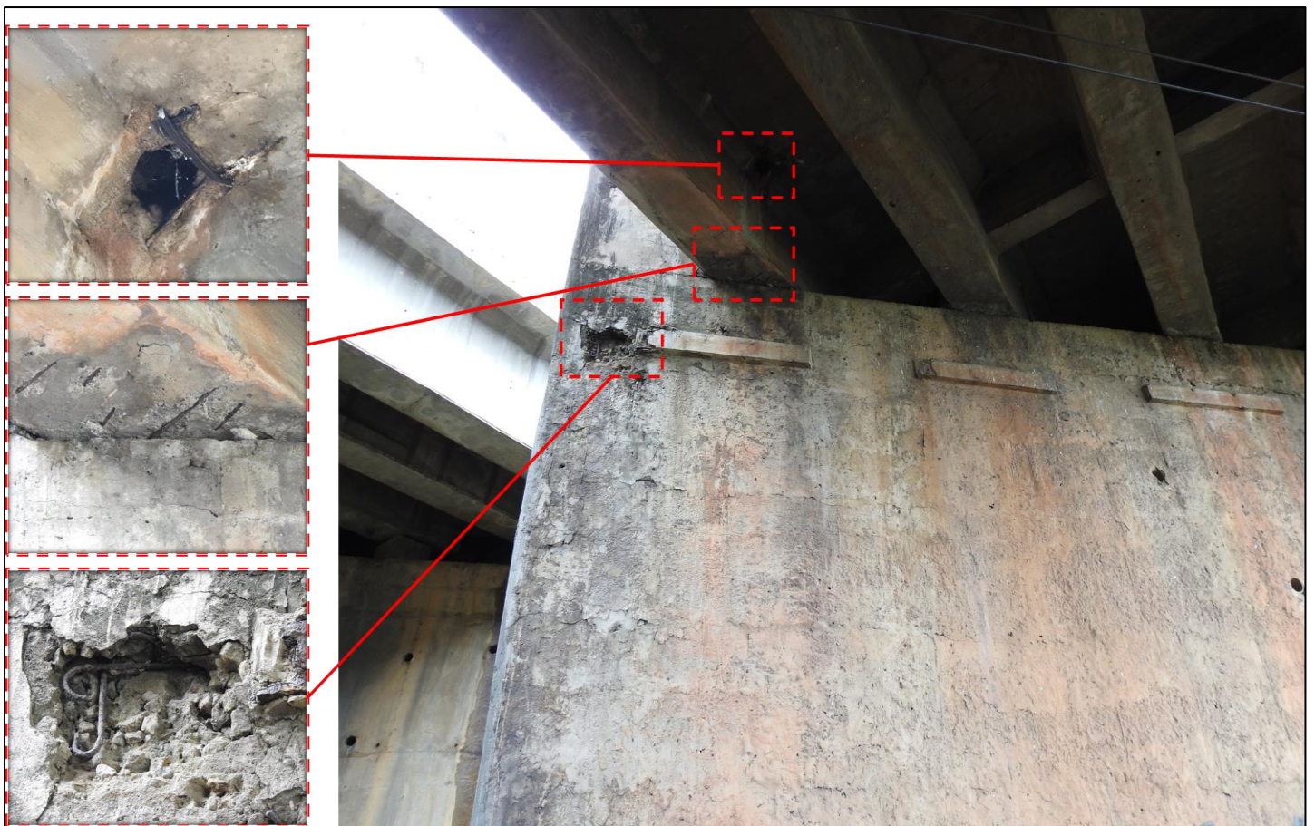
Fig 6: Reinforcement exposed in exterior girder, pier and slab at drainage spout
