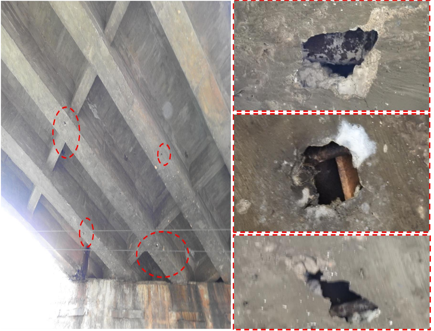
Fig 16: Minor spalled concrete holes on main girder.
