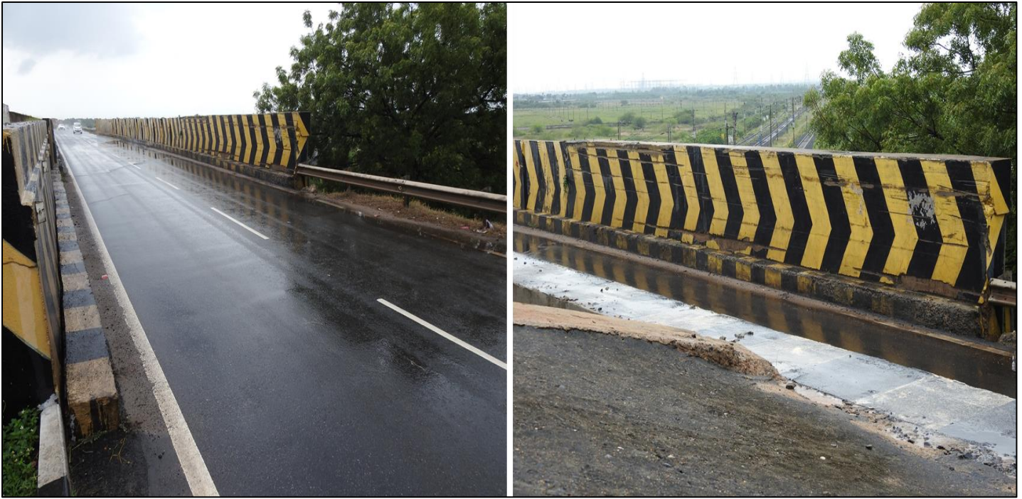
Fig 11: Wearing Coat condition & Accidental hitting marks on Crash Barrier.
