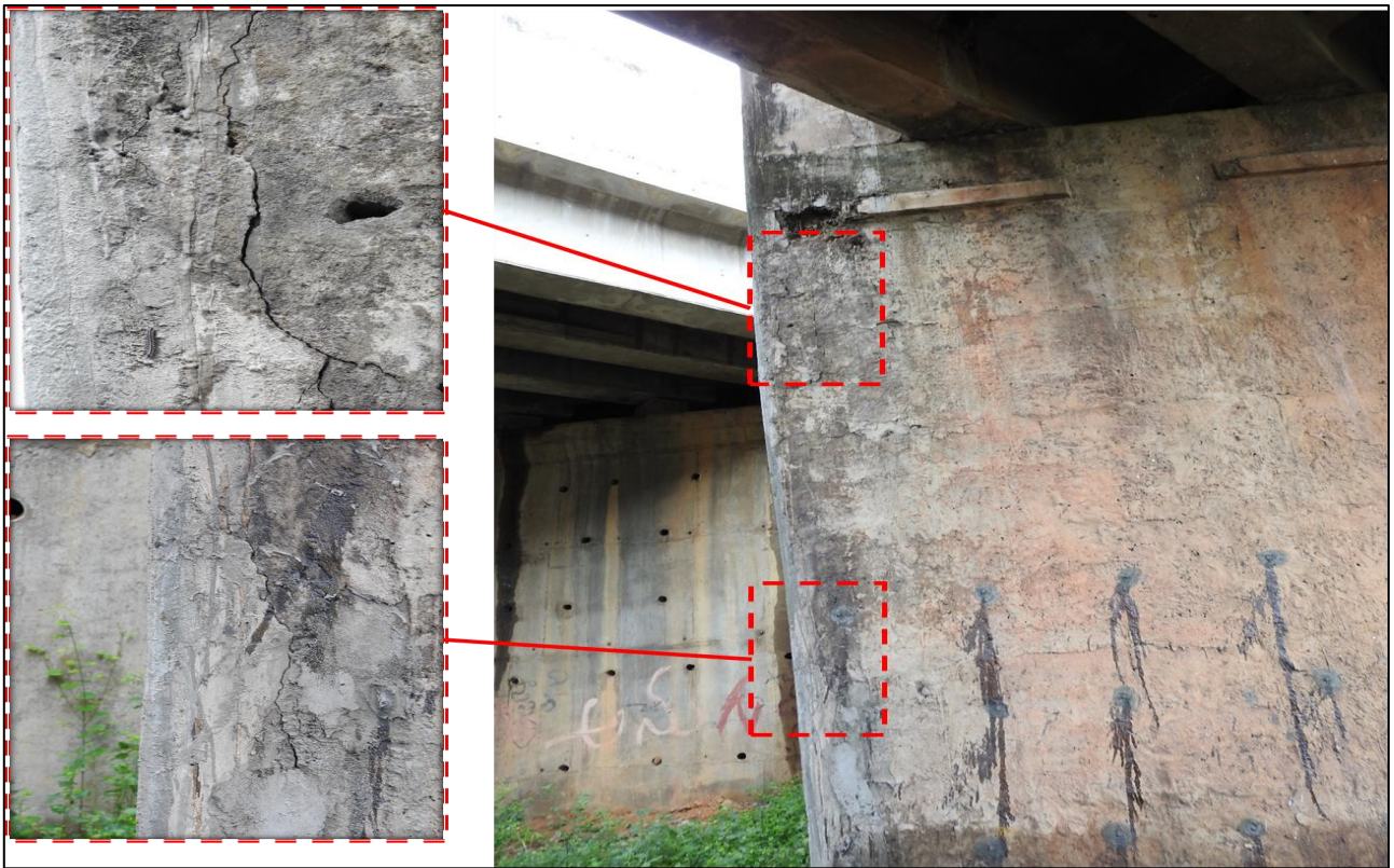
Fig 9: Cracks observed on pier
