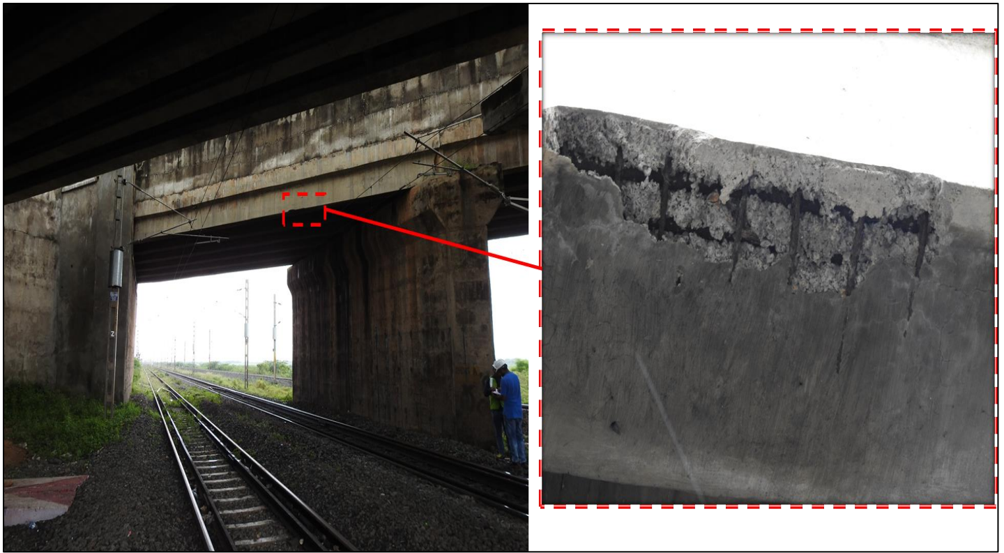
Fig 5: Reinforcement exposed in exterior girder
