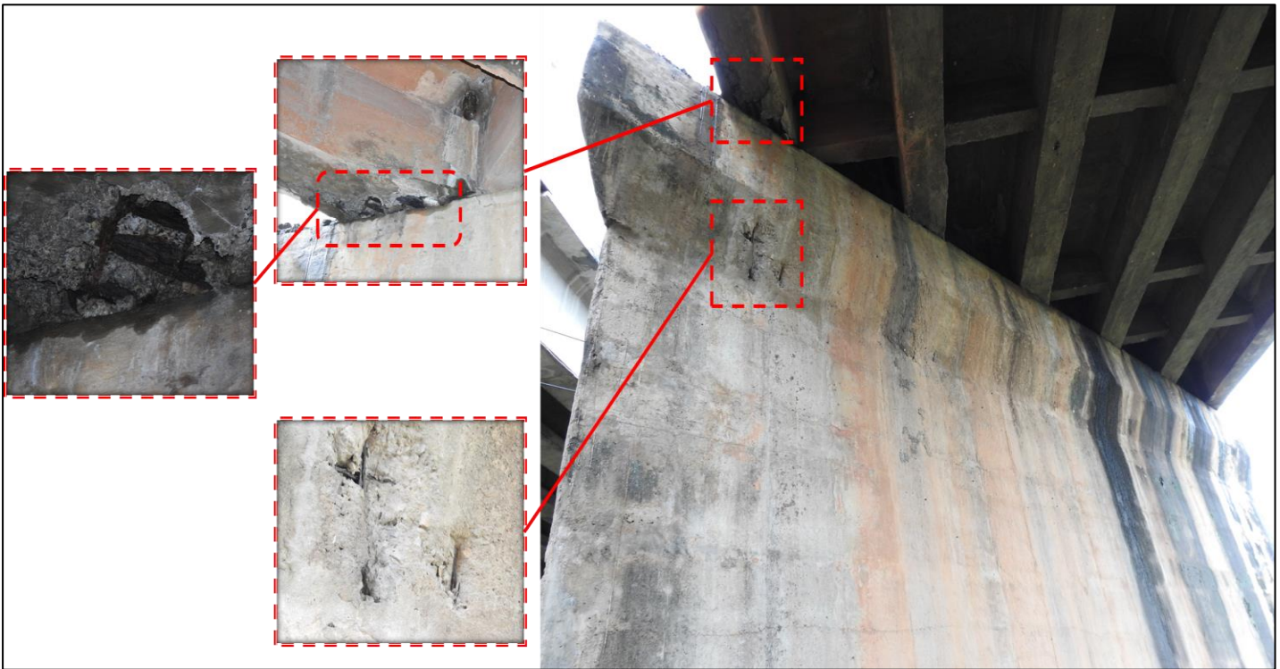
Fig 7: Reinforcement exposed, Leaching and cracks at girder end and Pier haunch
