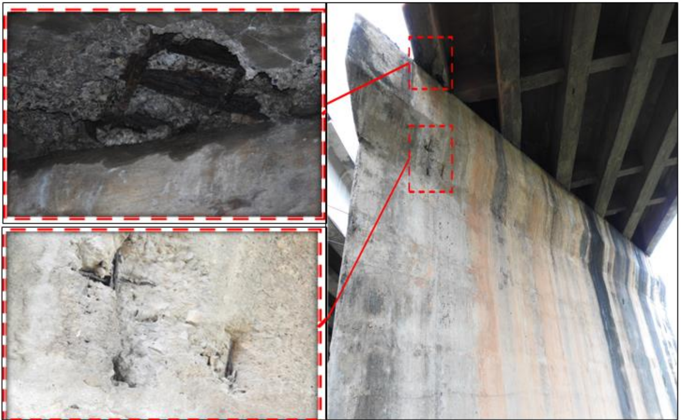
Fig 13: Reinforcement exposed at girder end and Pier haunch
