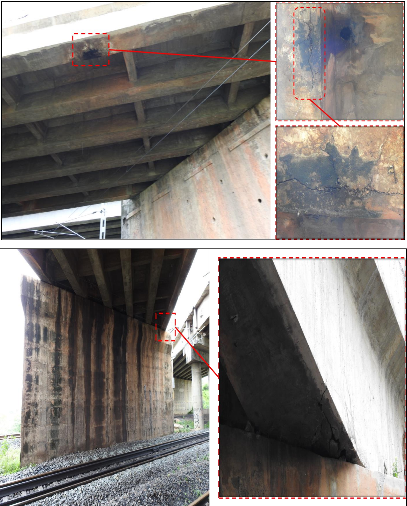
Fig 4: Cracks observed in Exterior girder
