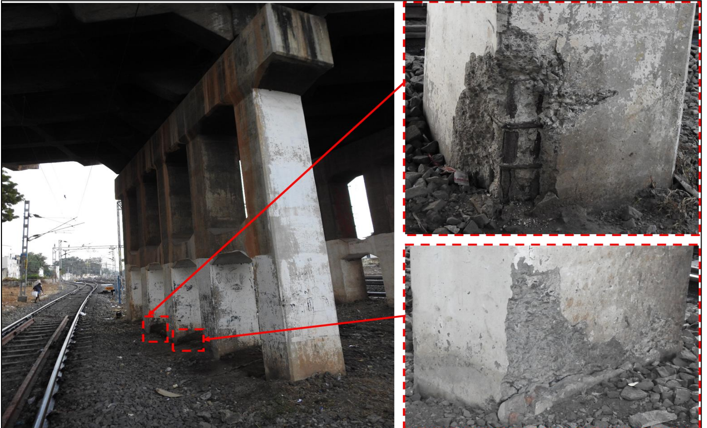
Fig 13: Reinforcement exposure & Spalling observed at columns of Pier-3
