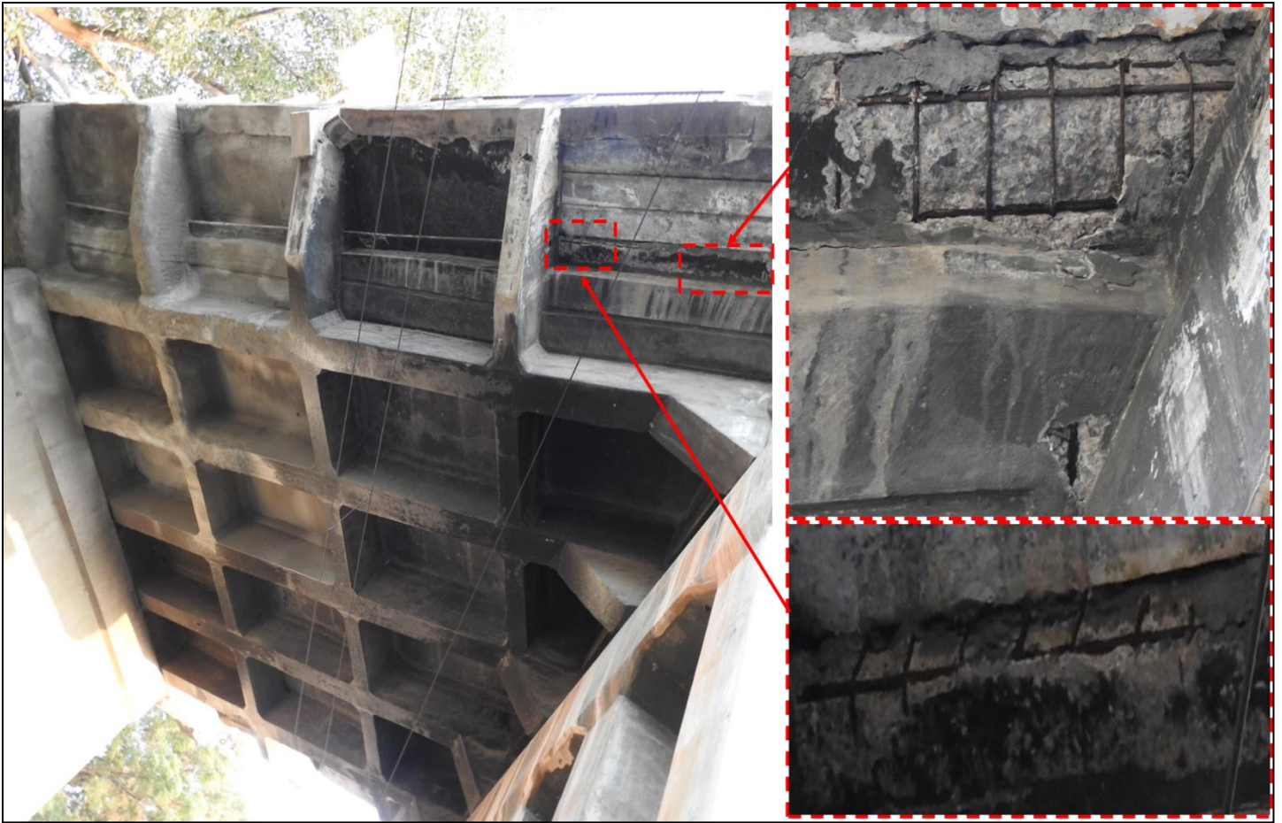
Fig 12: Reinforcement exposure observed at Slab of Span-3
