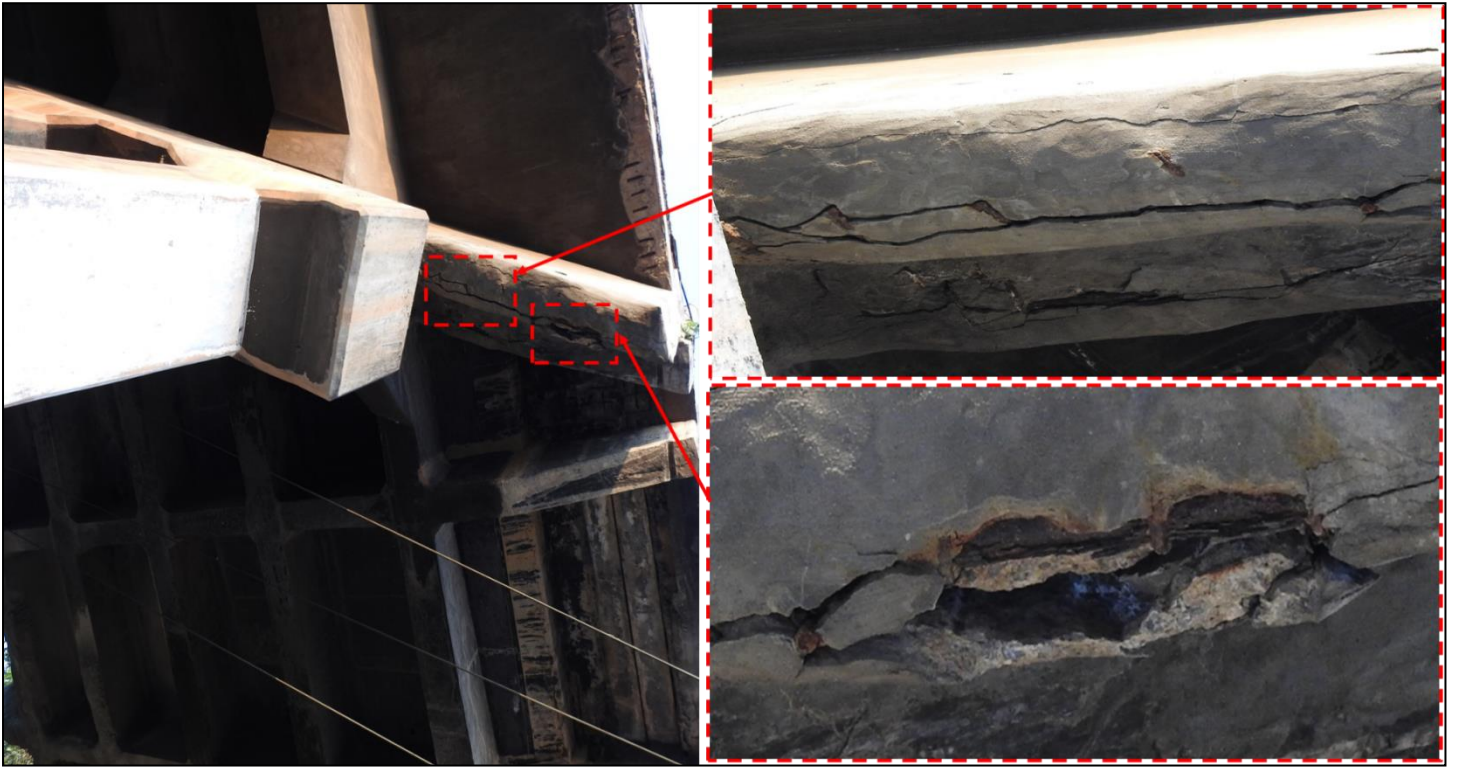
Fig 10: Severe Spalling & Reinforcement exposure observed at over hanging portion of cross girder in pier 2
