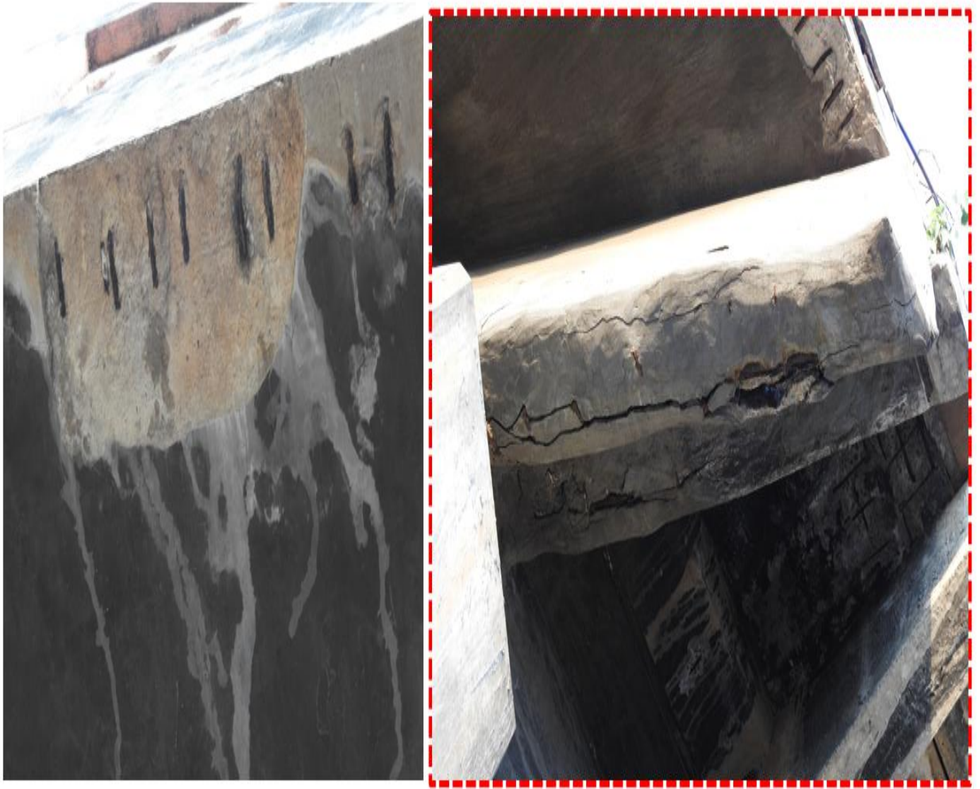
Fig: 20 Deterioration of Reinforcement and Major spalling of Deck slab.
