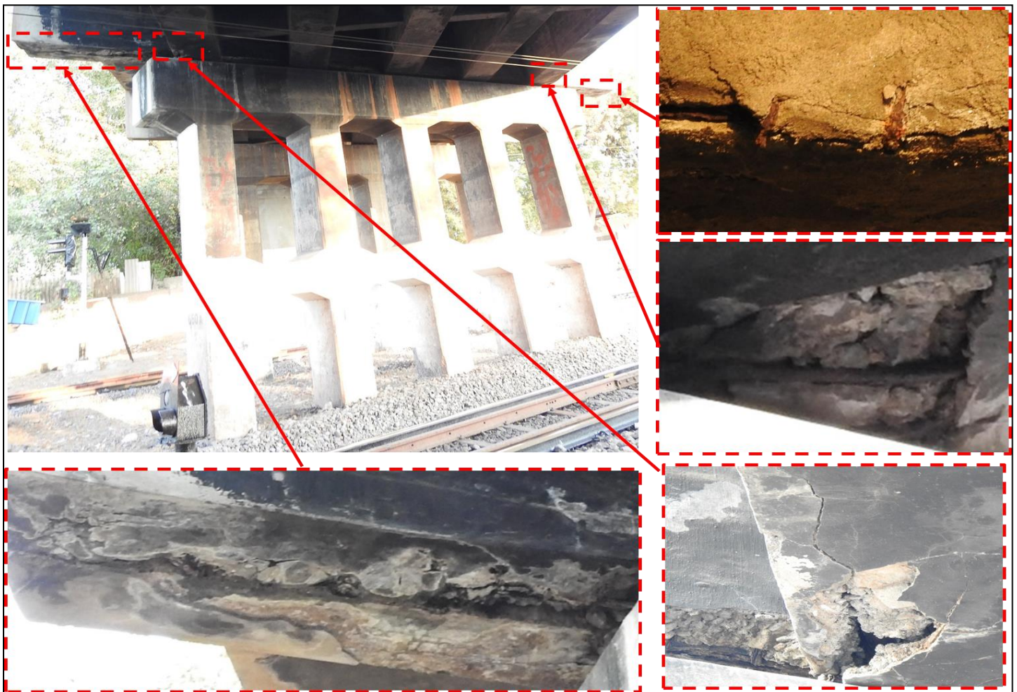
Fig 7: Reinforcement exposure & Spalling observed on Longitudinal & Cross girders of Span-1
