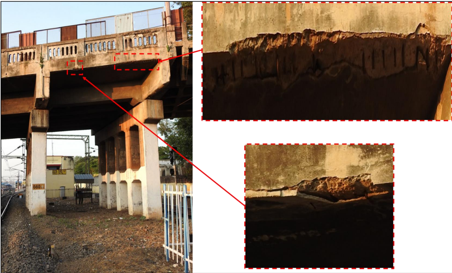
Fig 11: Spalling & Reinforcement exposure observed at over hanging portion of slab in Span-2
