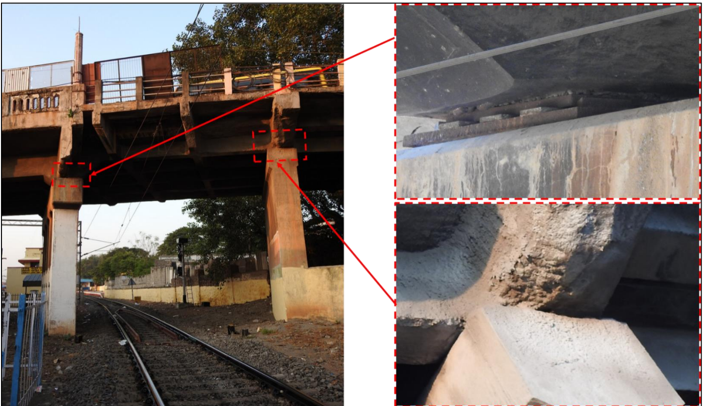
Fig 15: Debris accumulated at bearings of Span-2 and filled with Mortar at Span-3
