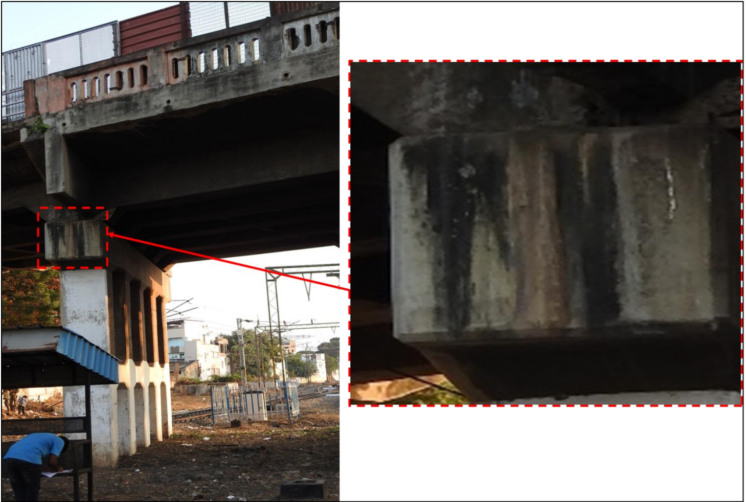
Fig 14: Leaching observed at Pier-3 cap
