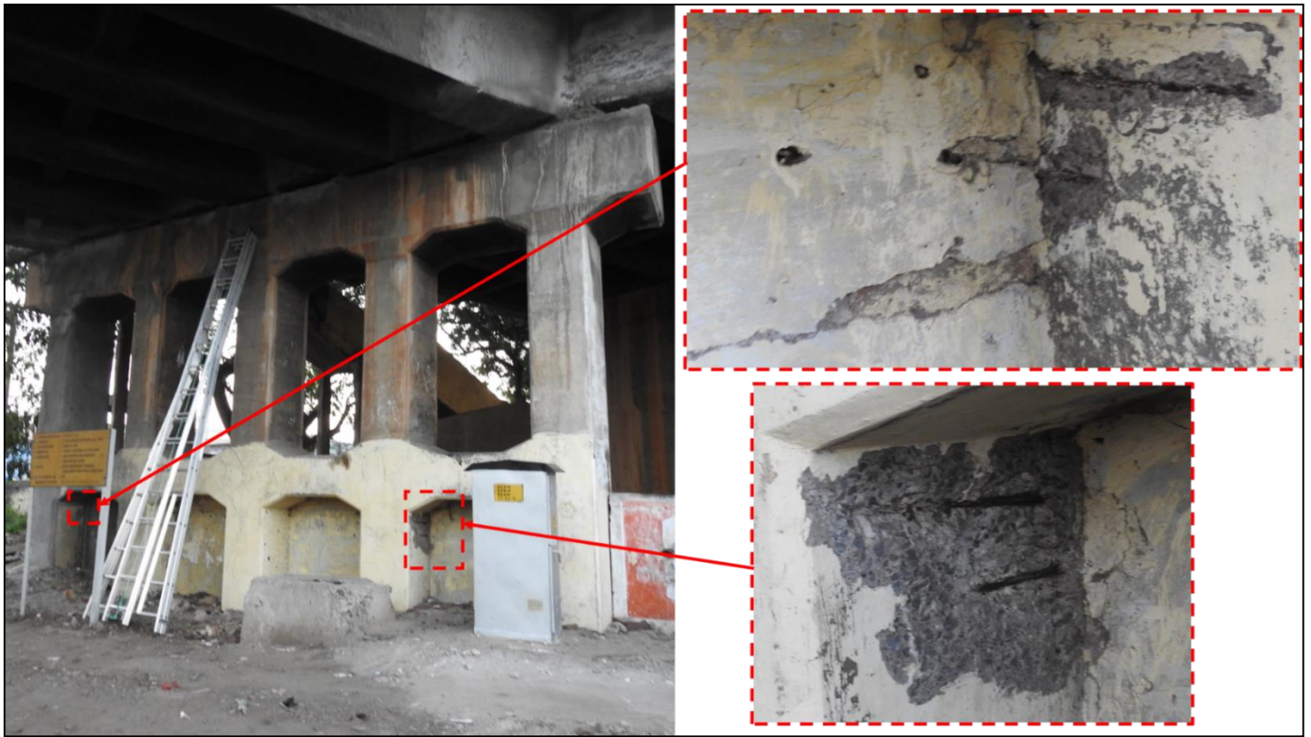
Fig 6: Reinforcement exposure observed in pier-1 columns
