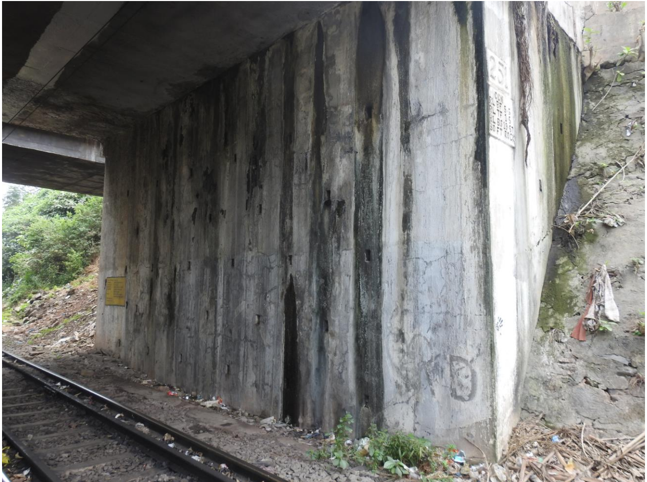
Fig: 4 Water seepage at abutment
