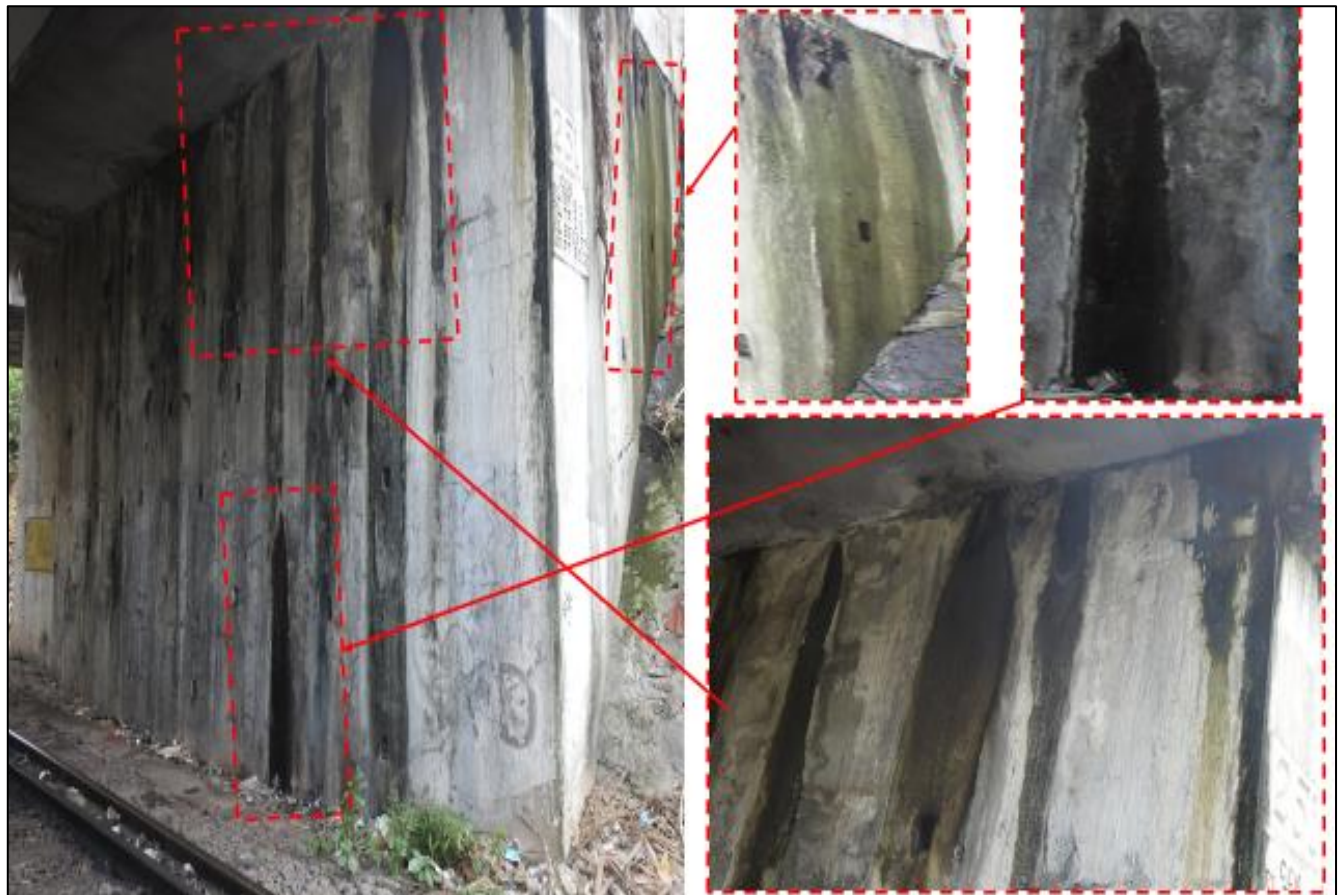
Fig 14: Algae observed on Abutment-2
