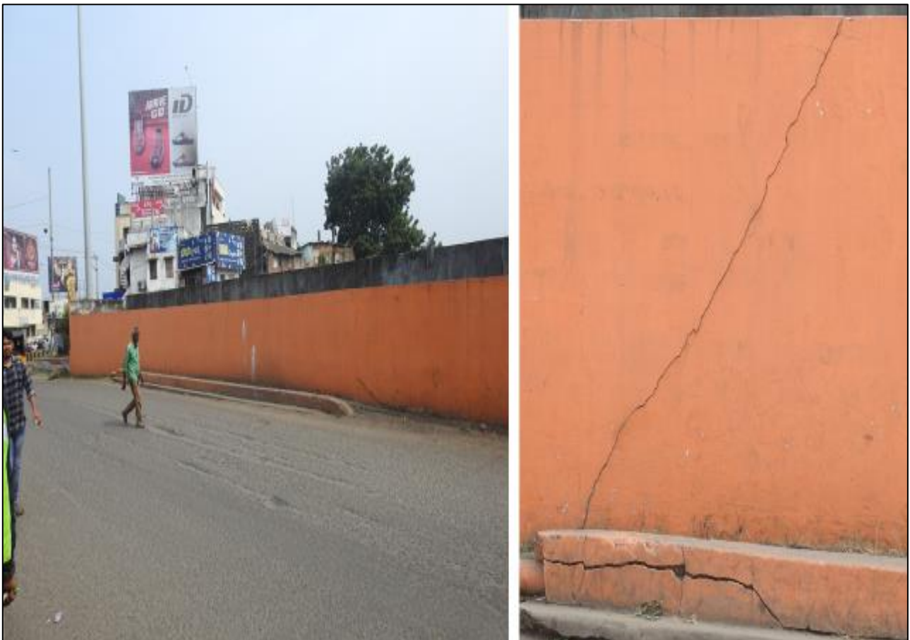
Fig: 3 Wearing coat & cracks observed on parapet wall
