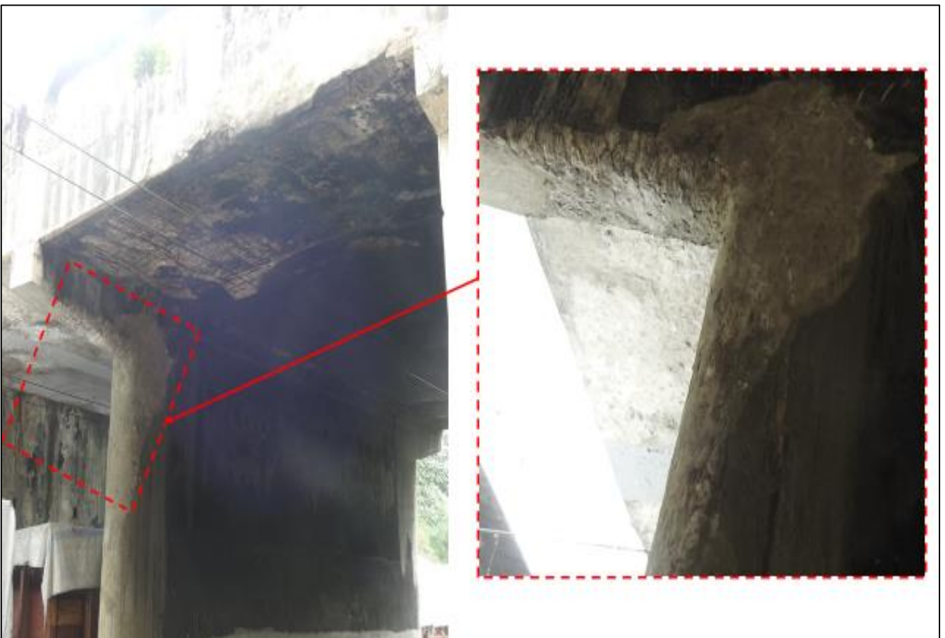
Fig 10: Cracks & Spalling observed at Pier
