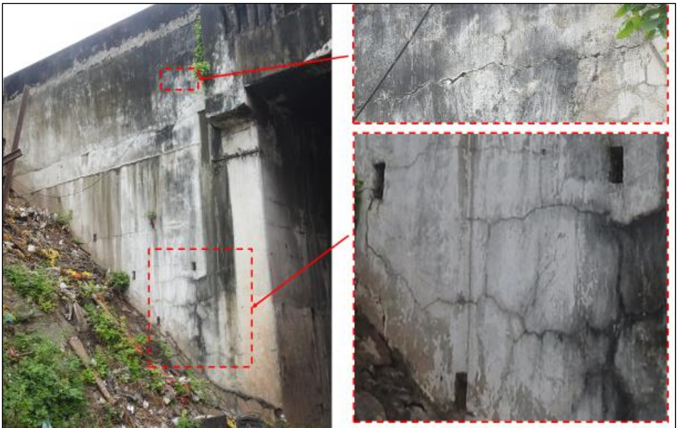
Fig: 5 Cracks observed at Abutment 1
