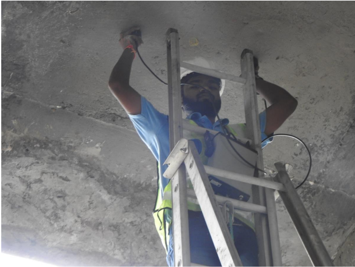
Fig 17: UPV test at Kadiyam ROB
