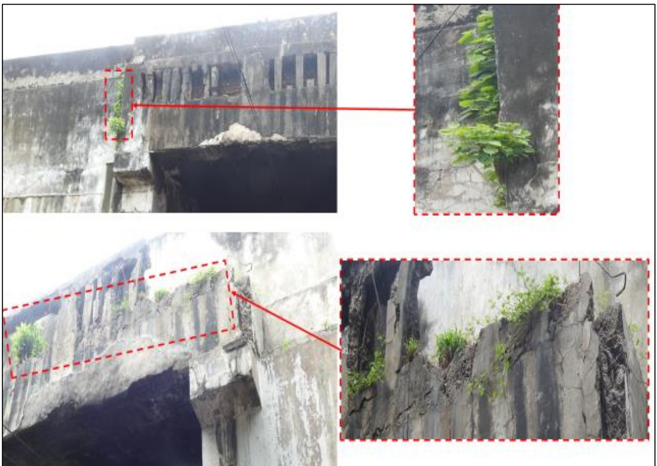
Fig 7: Vegetation growth observed at Abutment-1
