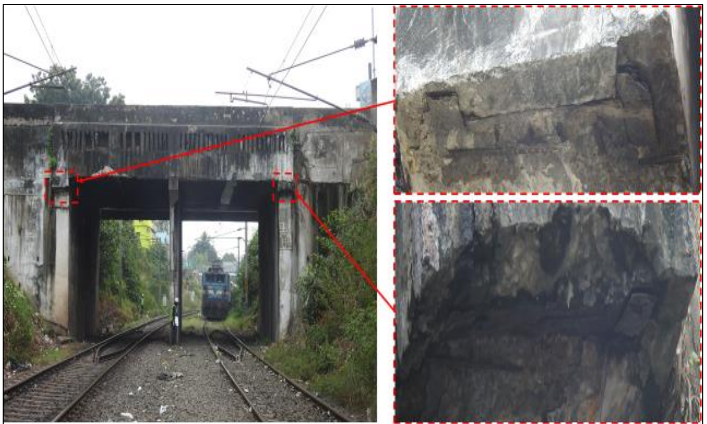
Fig 12: Spalling observed at both Abutment Pier caps
