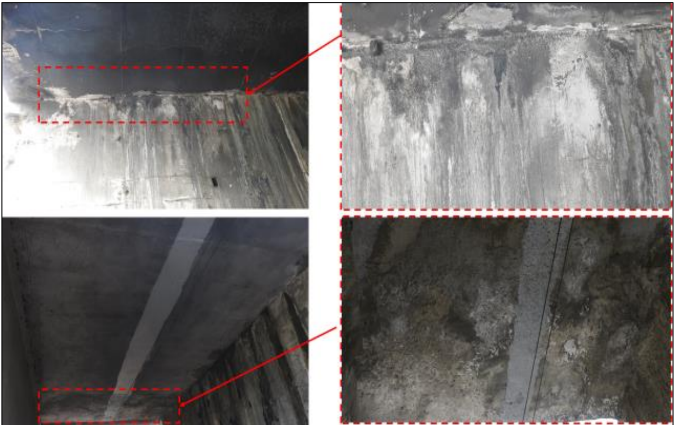
Fig 9: Leaching observed on Slab – 1 & Slab-2
