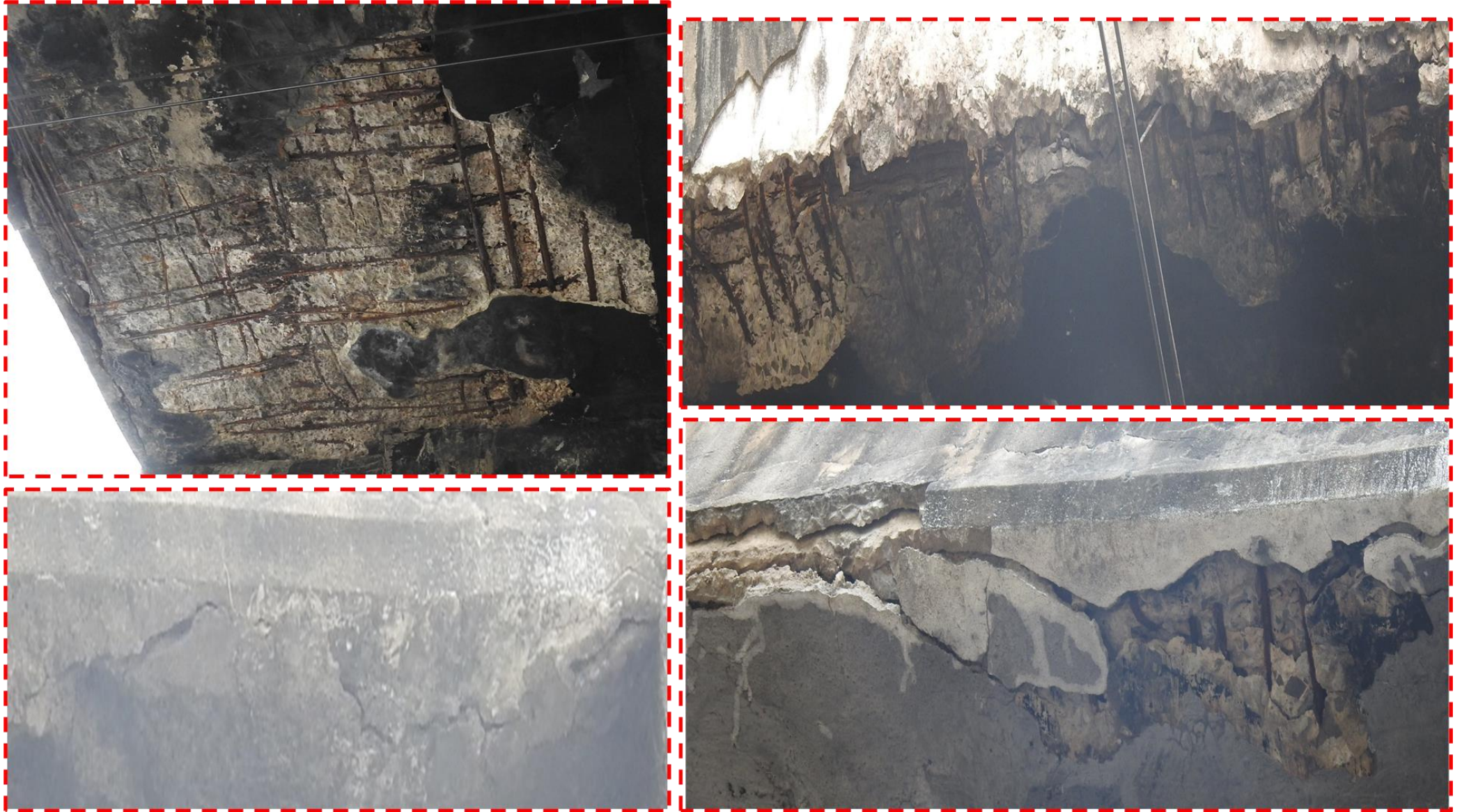
Fig: 20 Deterioration of Reinforcement and Major spalling of Deck slab.
