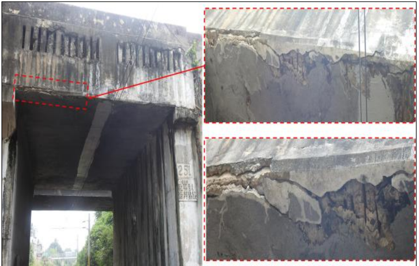
Fig 11: Reinforcement exposure observed at Span-2
