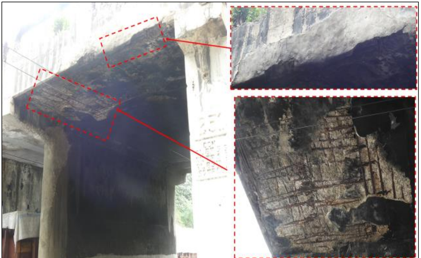
Fig 8: Reinforcement exposure & Spalling observed at Span-1
