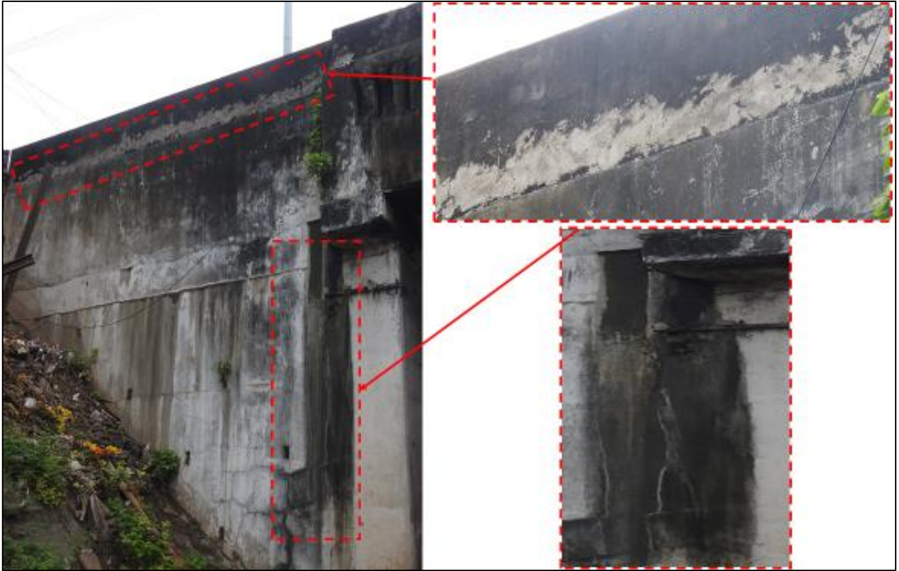
Fig:6 Patch work & Leaching observed at Abutment-1
