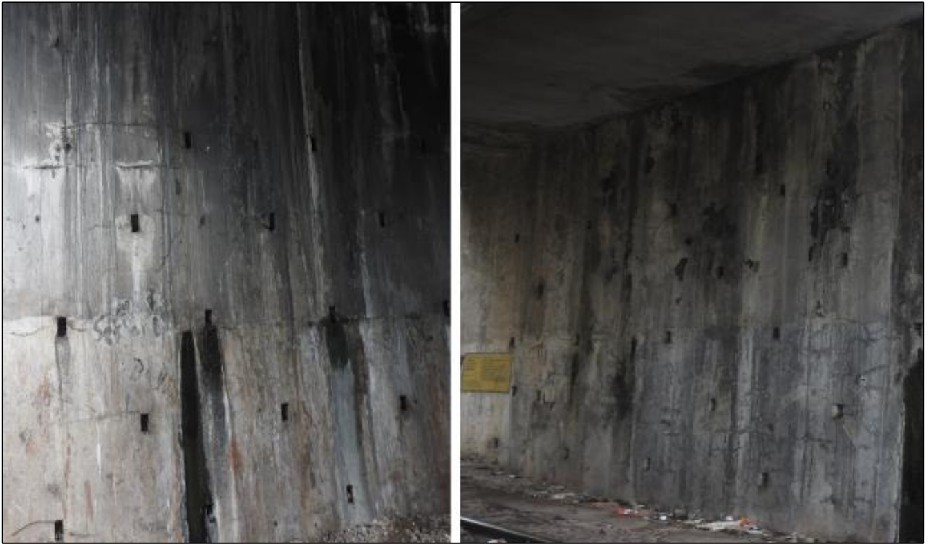
Fig 13: Shrinkage cracks observed on A1 & A2 Abutments
