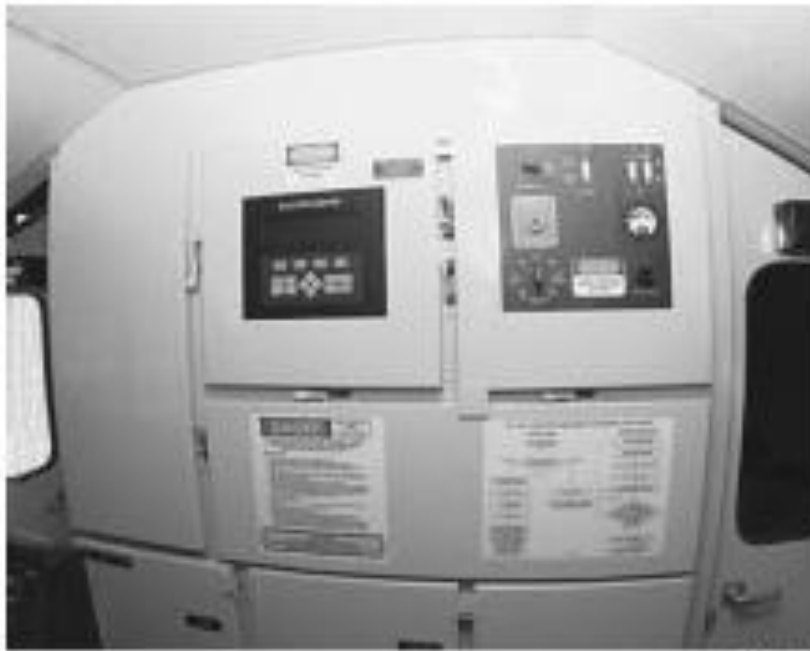
Figure 2-15. No.1 Electrical Control Cabinet (ECC1), Typical F41972
