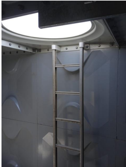
Internal FRP Ladder
