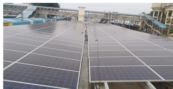
Solar COP at Vijayawada Railway station
