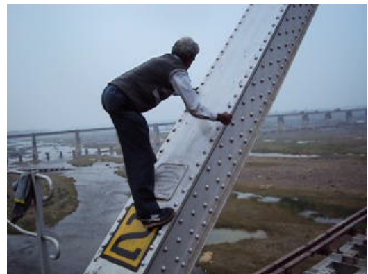
Figure 1: Bridge official climbing end raker of girder without inspection arrangement.
