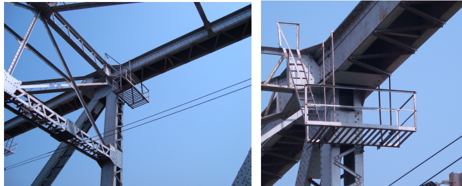
Figure 7: Long and close-up view of cradle provided at node of open web girder.
