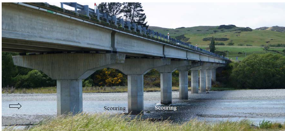
Fig. 1.1 Scour taking place at bridge piers in a field condition
