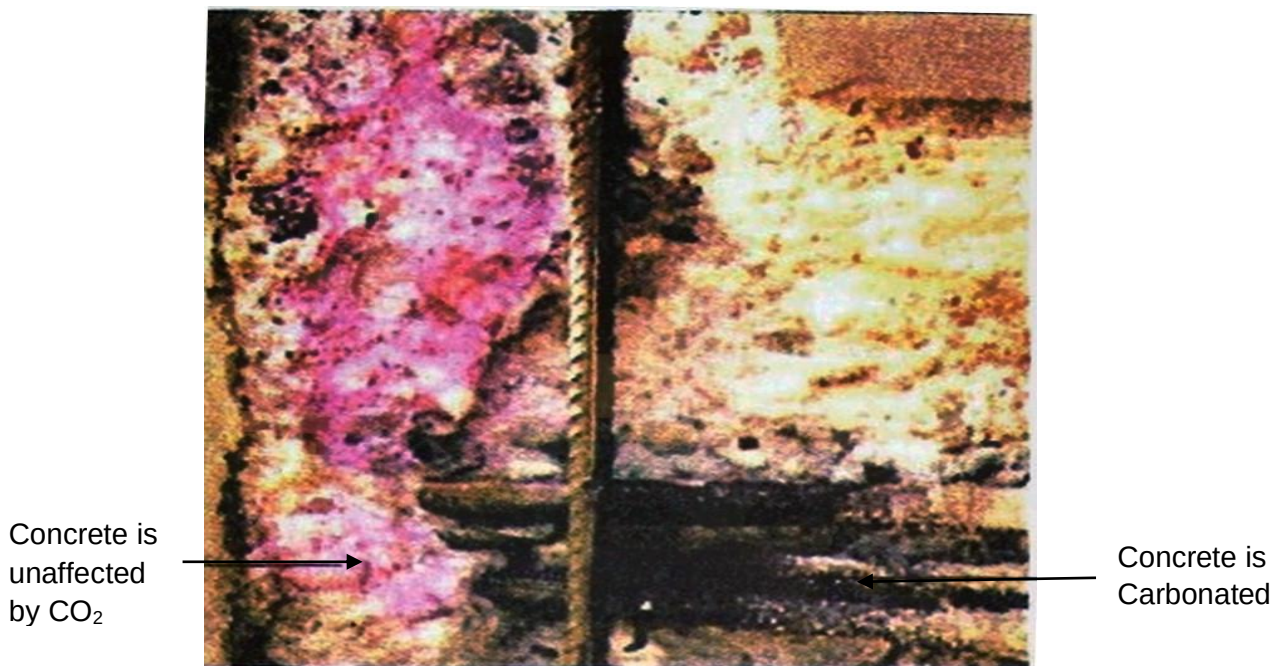
Fig: Pink Colour indicates that \text{Ca (OH)}_2 is unaffected by carbonization. The uncoloured portion indicates that concrete is carbonated.
