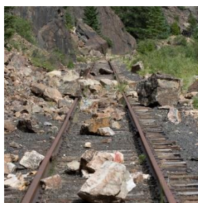
Obstruction on track
